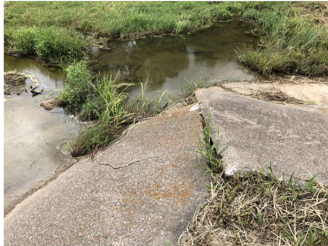
REPAIR M1403 SOUTH END RIPRAP SCOUR, UNDERMINING, AND SETTLEMENT
