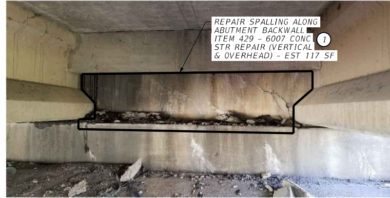
REPAIR SB2102 SW ABUTMENT CAP HAS CONCRETE SPALL WITH EXPOSED REBAR
