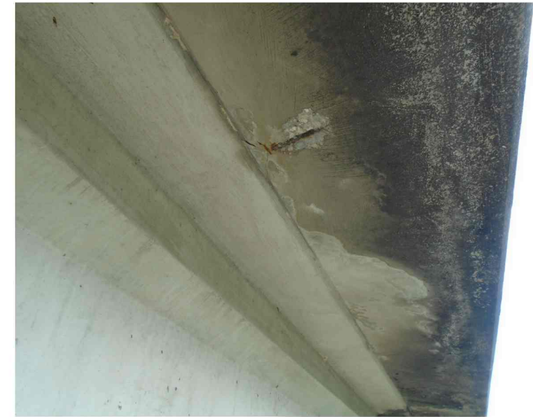
REPAIR D1303 SOUTH SIDE OF SPAN 1 DECK SOFFIT
