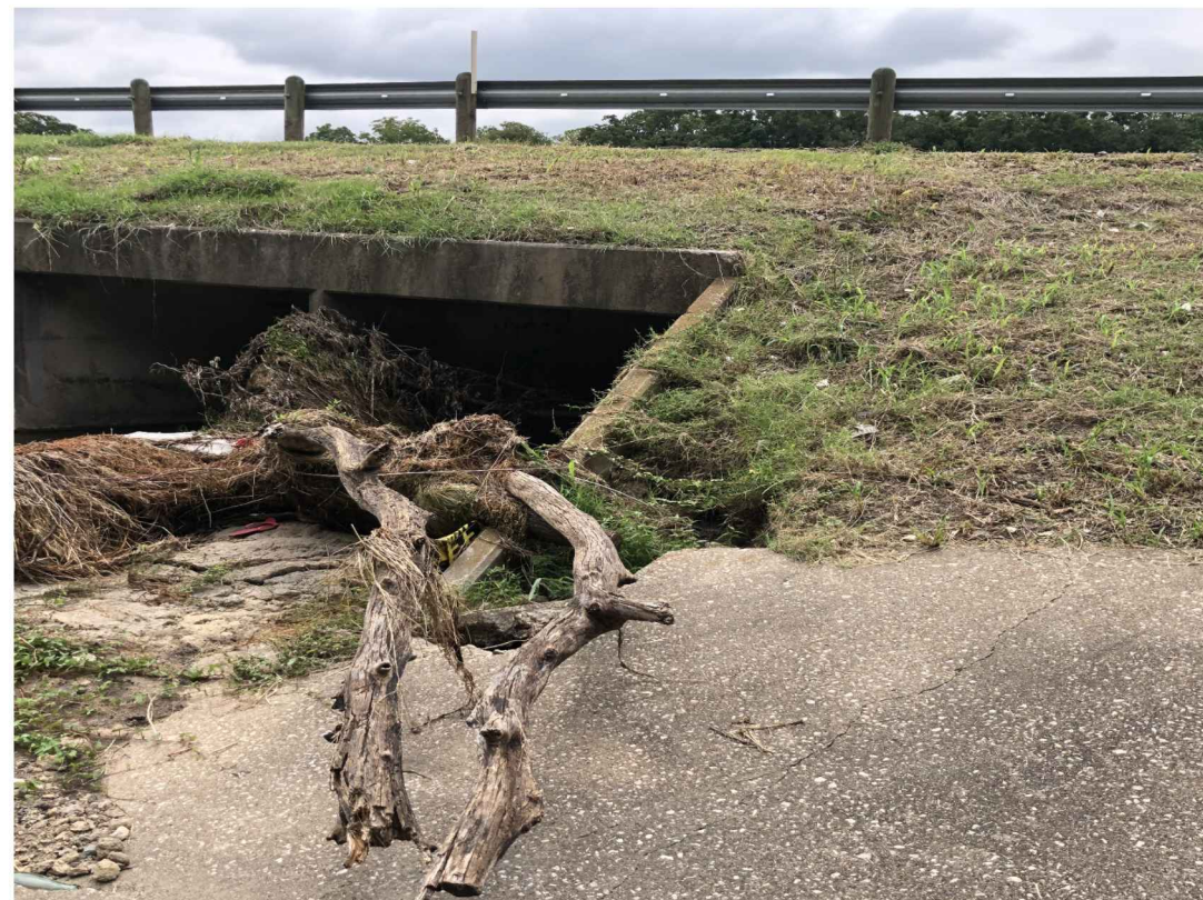
REPAIR M1406 NORTH END RIPRAP SCOUR, UNDERMINING, AND SETTLEMENT
