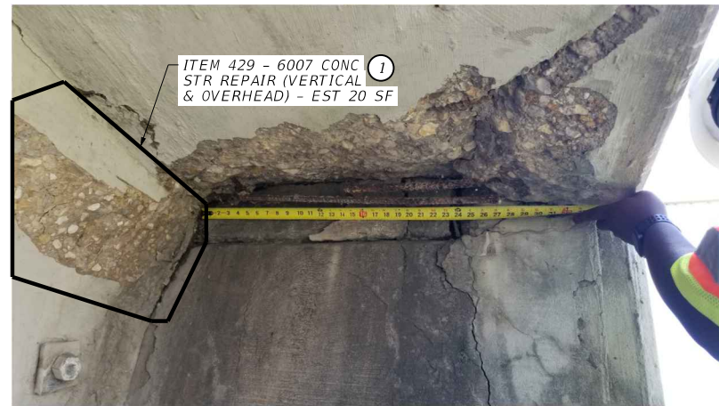
REPAIR SP2101 GIRDER ENDS AT SW ABUTMENT CAP HAVE AREAS OF SPALL/DELAMINATION
