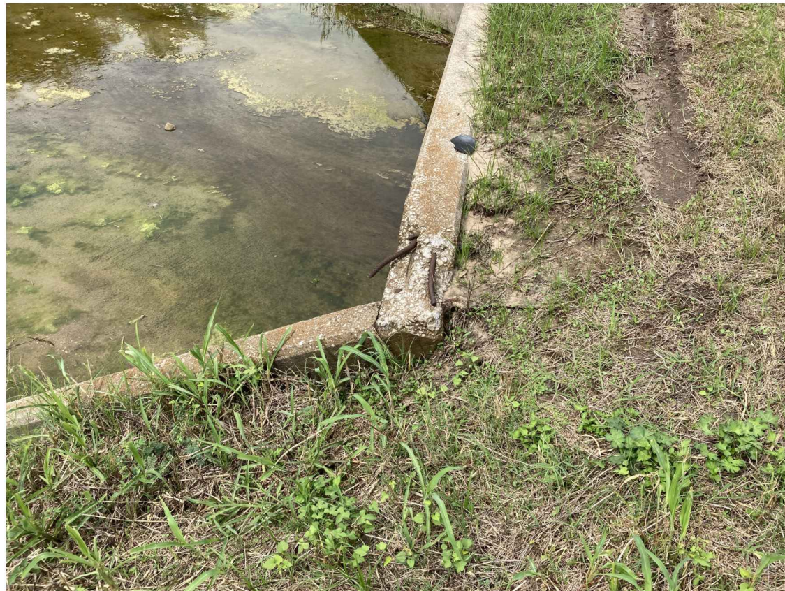
REPAIR SB1402 SOUTH END CURB WALL SPALL
