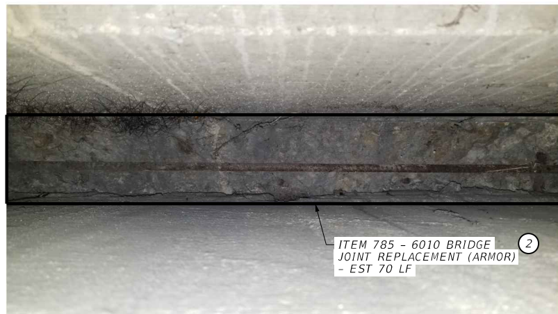
REPAIR D2102 SW END JOINT HAS FAILED
