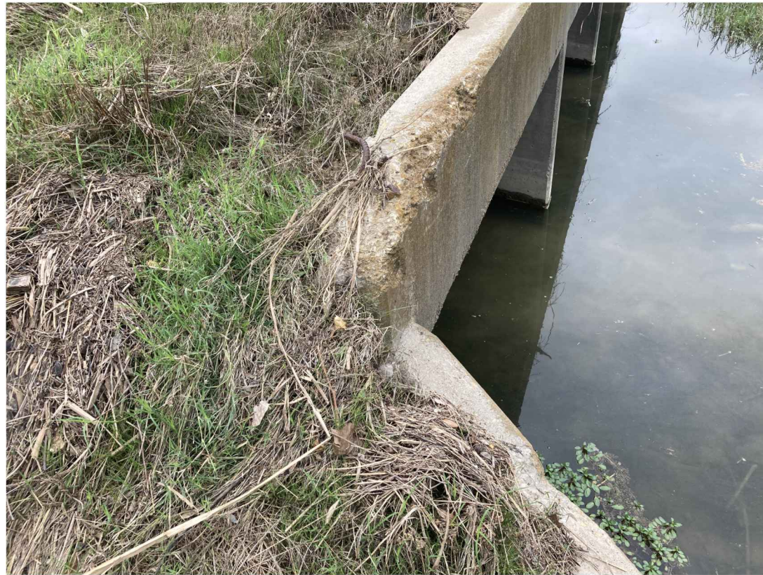
REPAIR SB0601 NORTHEAST CORNER SPALL
