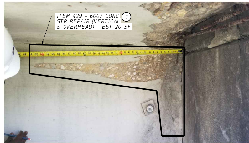
REPAIR SP2101 GIRDER ENDS AT SW ABUTMENT CAP HAVE AREAS OF SPALL/DELAMINATION
