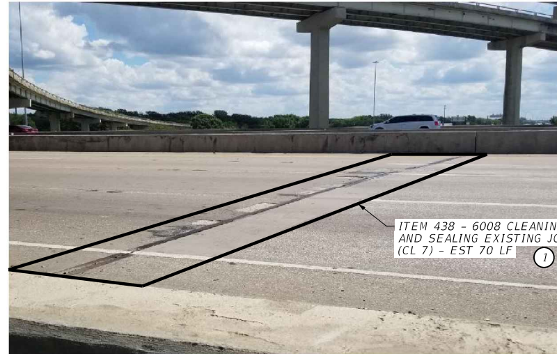
REPAIR D2201 SOUTHWEST EXPANSION JOINT NEEDS TO BE CLEANED
