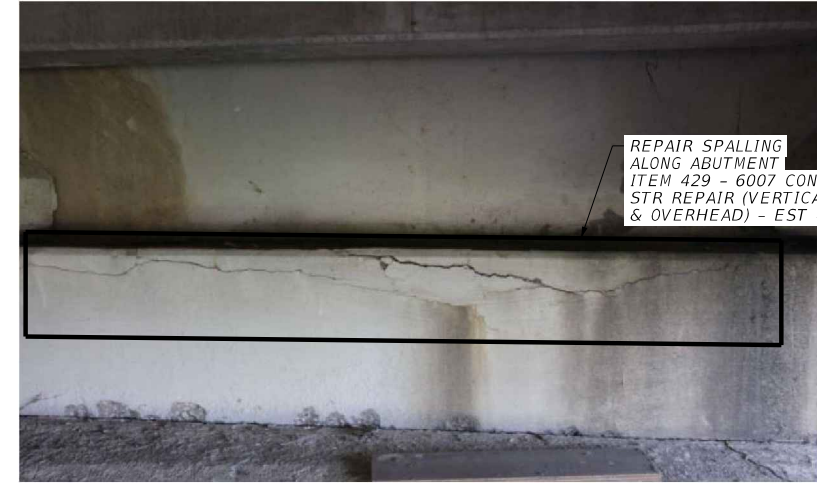
REPAIR SB2101 NE ABUTMENT CAP HAS CRACKED/SPALLED DELAMINATION
