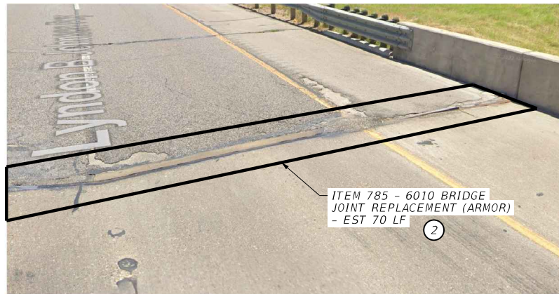
REPAIR D2102 SW END JOINT HAS FAILED
