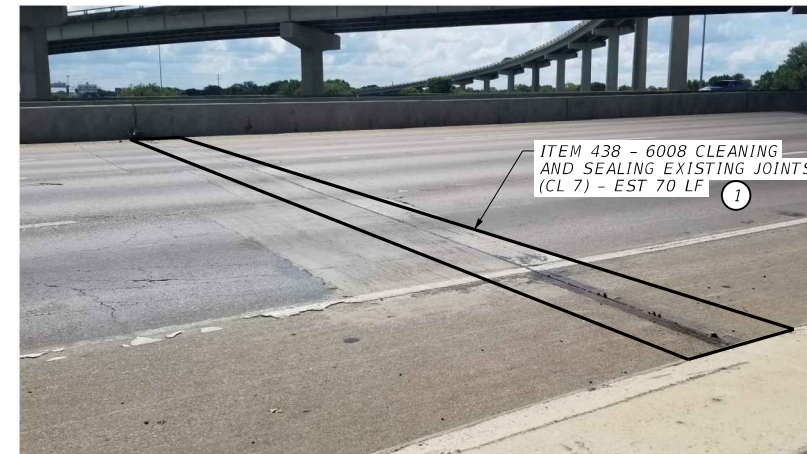
REPAIR D2201 NORTHEAST EXPANSION JOINT NEEDS TO BE CLEANED
