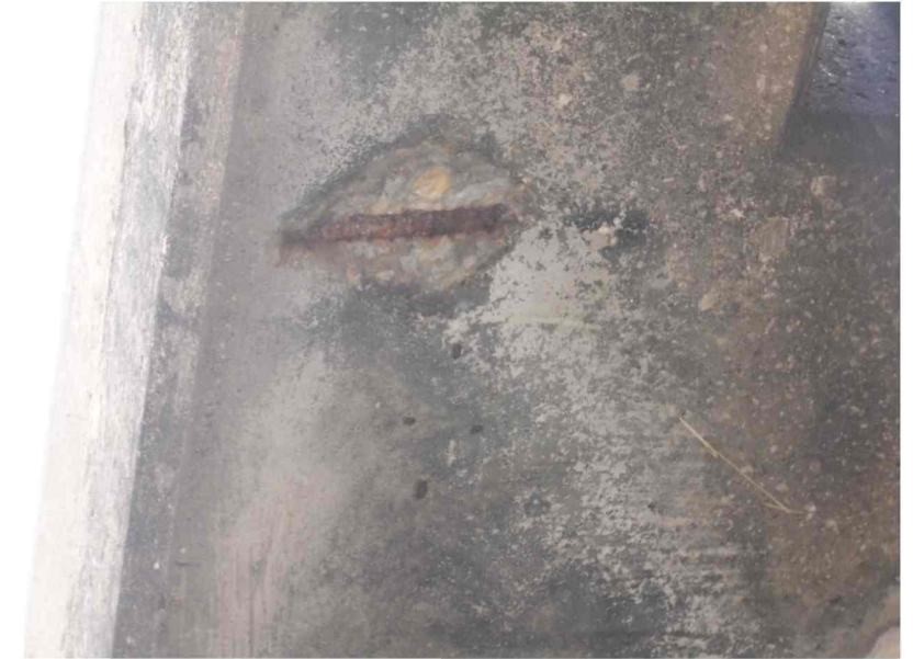
REPAIR D1203 SPAN 2 DECK SOFFIT NORTH SIDE FROM BELOW (REPAIR D0104 SIMILAR)
