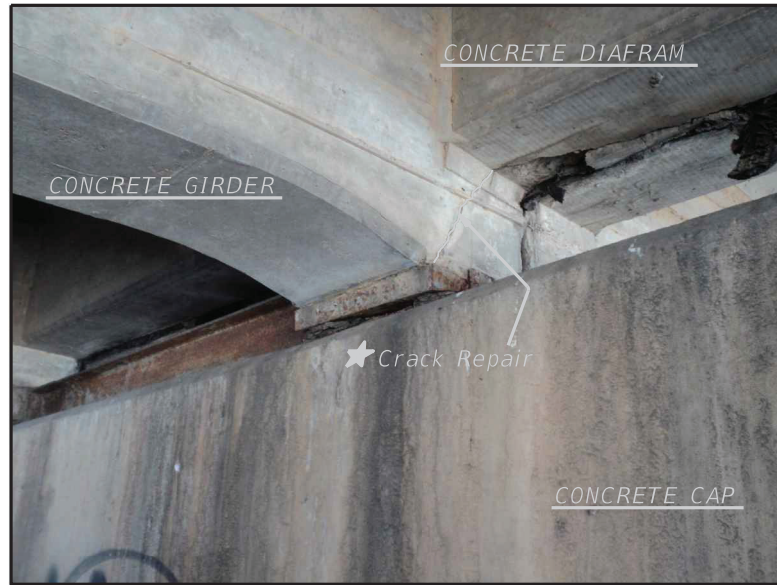
CRACKED GIRDER END - CONDITION "B"
