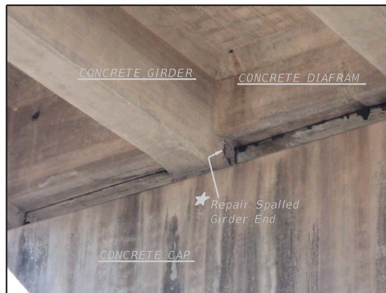
SPALLED/CRACKED GIRDER END - CONDITION "C" (SEE TABLE FOR CONDITION "C" LOCATIONS)
