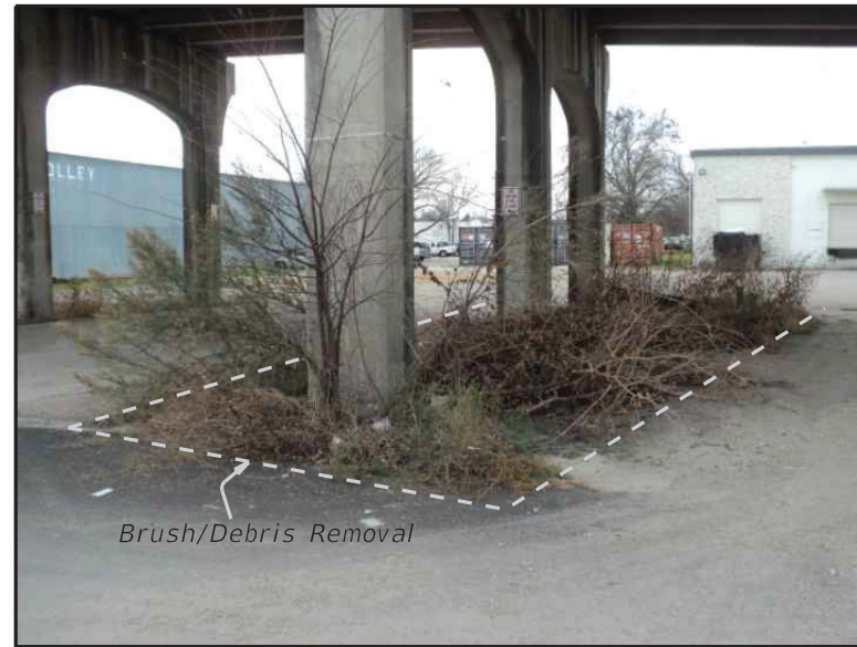
BRUSH/DEBRIS REMOVAL (SHOWING TYPICAL INTERIOR BENT LOCATION AT NORTH END) NOTE: SIMILAR AT VARIOUS LOCATIONS
