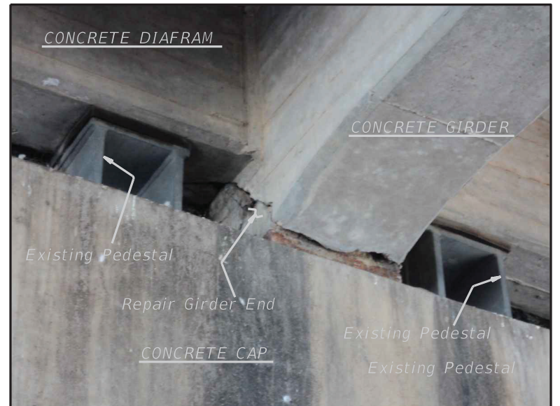
BROKEN GIRDER END - CONDITION "A" (SEE TABLE FOR CONDITION "A" LOCATIONS)
