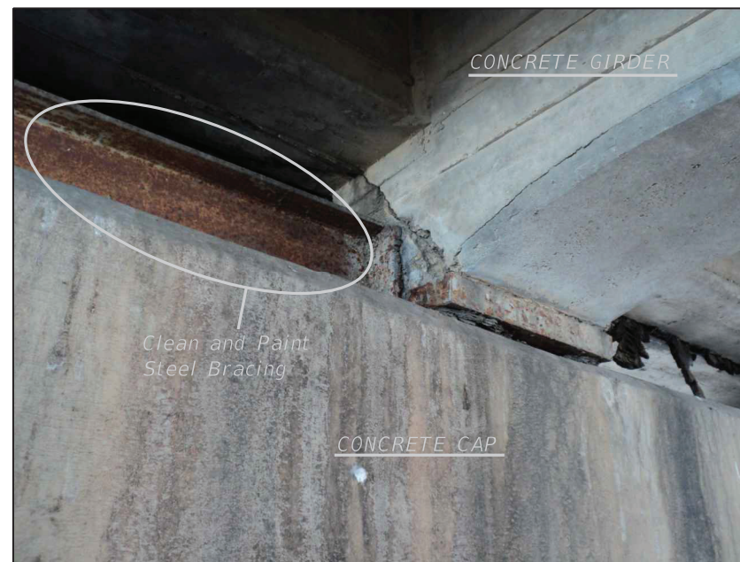
TYPICAL RUSTED STEEL BRACING (SHOWING CONDITION OF EXISTING STEEL BRACING)
