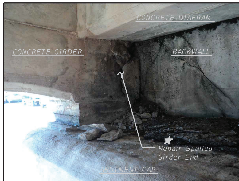
SPALLED GIRDER END - CONDITION "C" (SEE TABLE FOR CONDITION "C" LOCATIONS)
