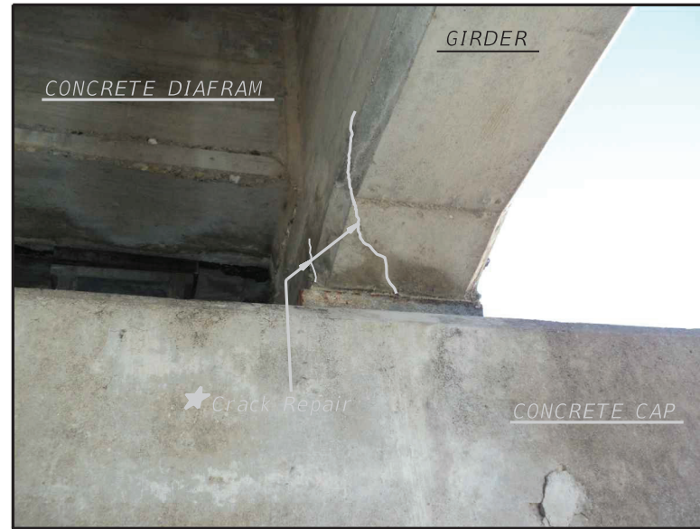
CRACKED GIRDER END - CONDITION "B"
