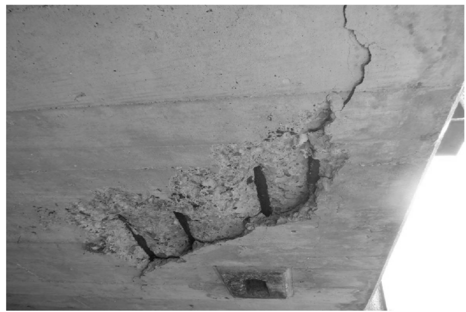
SPALL WITH EXPOSED REBAR ON SLAB SOFFIT AT SOUTH EDGE IN EAST SPAN LOOKING EAST
