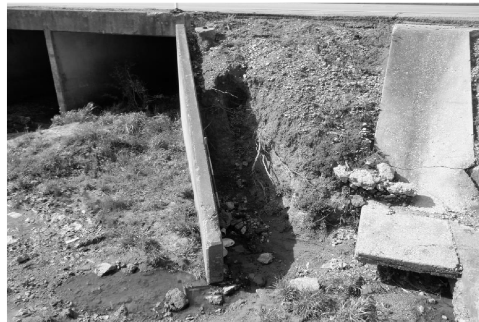
EMBANKMENT EROSION AT SE CULVERT CORNER EXPOSING BEHIND SE WINGWALL AND UNDERMINING CONCRETE DRAINAGE FLUME LOOKING NORTH
