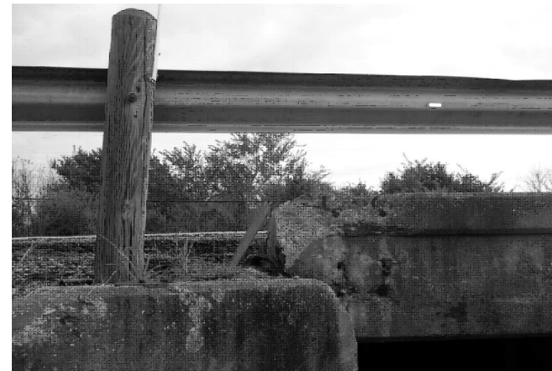
SPALL WITH EXPOSED REBAR AT WEST END OF SOUTH CONCRETE CURB AT MISSING STEEL RAILING POST LOCATION LOOKING NORTH
