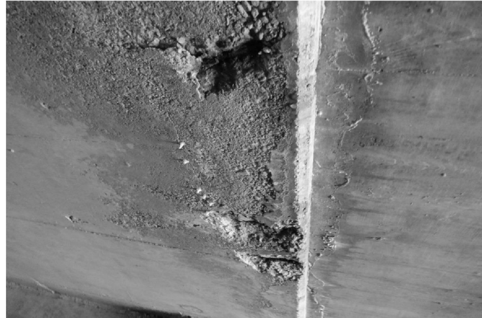
TYPICAL SPALLS WITH EXPOSED REBAR ON SLAB SOFFIT LOOKING WEST
