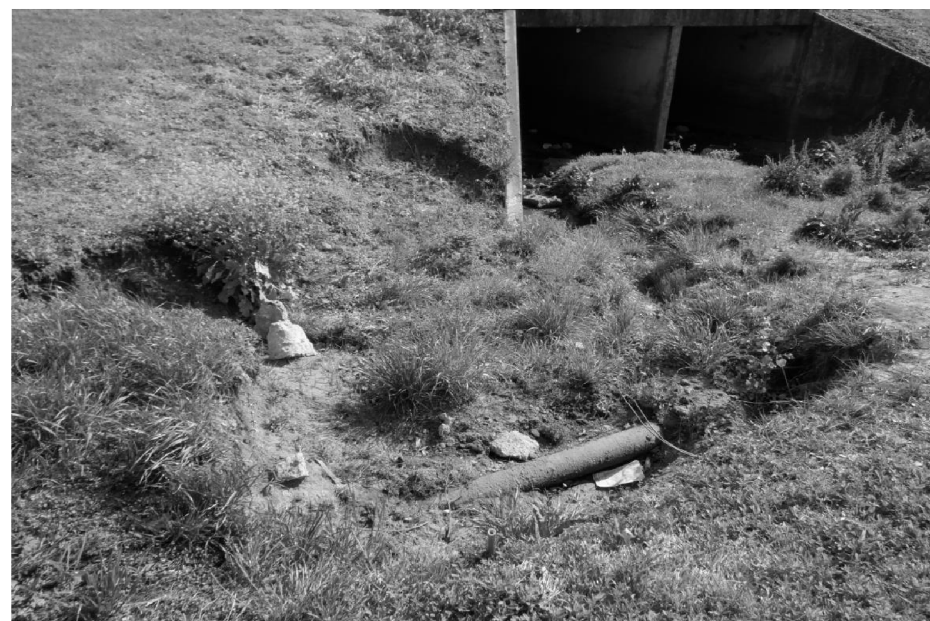
EROSION HOLE AT NE BRIDGE CORNER EXPOSING END OF WINGWALL LOOKING SOUTHWEST
