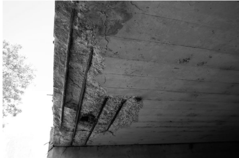
CRACKING, DELAMINATION, AND SPALLING WITH EXPOSED REBAR ON TOP SLAB SOFFIT AT SOUTH END OF BARREL 2 LOOKING WEST
