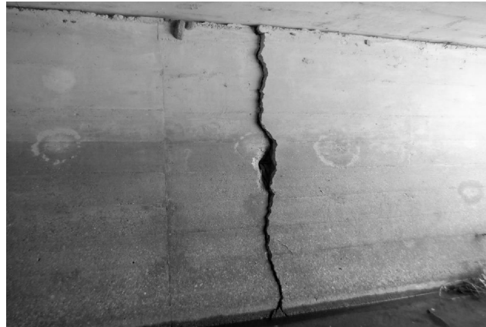
VERTICAL CRACKING AND ROTATION OF EAST ABUTMENT WALL LOOKING SOUTHEAST
