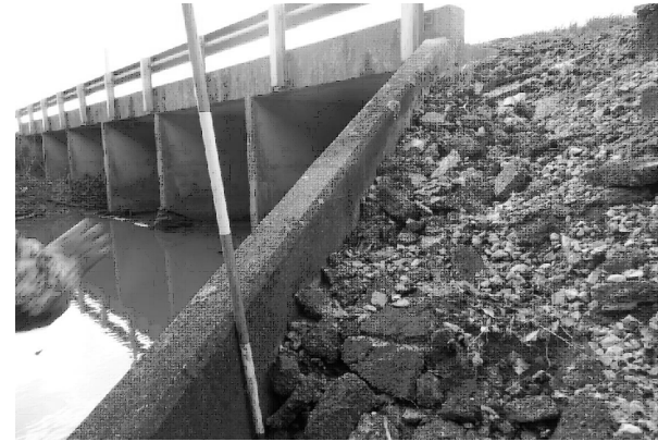
EMBANKMENT EROSION BEHIND NW WINGWALL LOOKING SOUTHEAST
