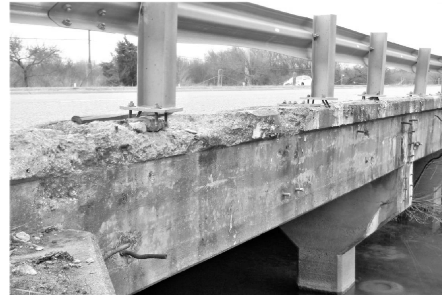
IMPACT DAMAGE TO SOUTH BRIDGE RAILING AND SPALLS WITH EXPOSED ON CONCRETE CURB LOOKING NORTHEAST
