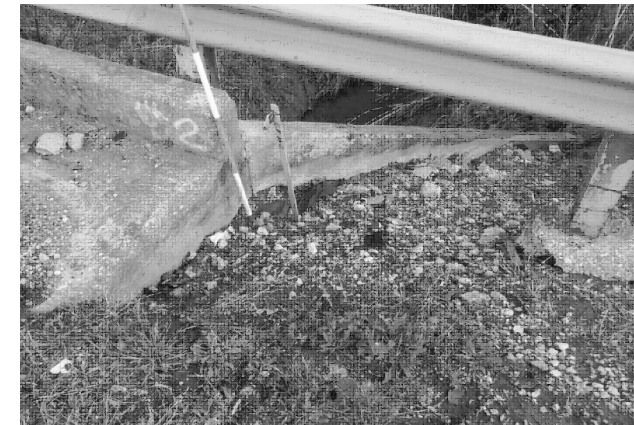
EMBANKMENT EROSION BEHIND NE WINGWALL LOOKING SOUTHEAST
