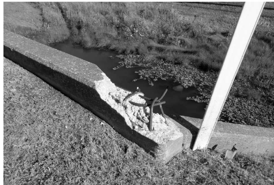
SPALLING WITH EXPOSED REBAR ON NORTH HEADWALL AT THE NE CORNER LOOKING NORTHWEST
