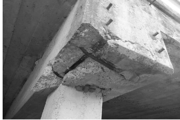
SPALLS WITH EXPOSED REBAR AT SOUTH END OF BENT CAP 2 LOOKING NORTHEAST
