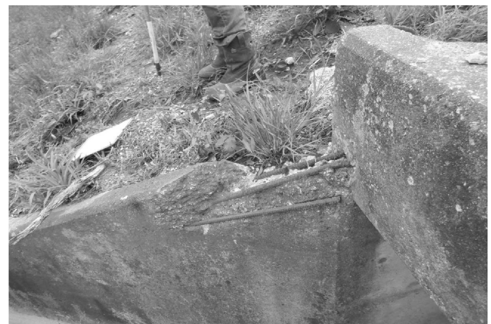
SPALL WITH EXPOSED REBAR ON TOP OF NE WINGWALL AT HEADWALL INTERFACE LOOKING EAST
