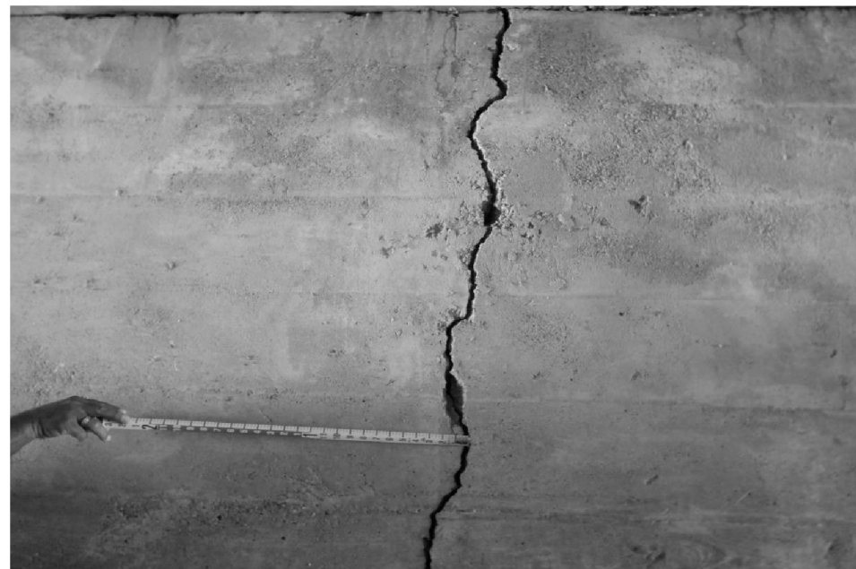
VERTICAL CRACK ON WEST ABUTMENT WALL LOOKING WEST
