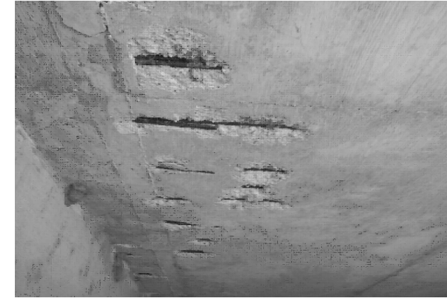
SPALLS WITH EXPOSED REBAR ON BOTTOM OF TOP SLAB IN BARREL 4 LOOKING SOUTH
