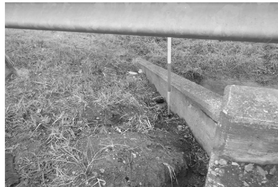
EMBANKMENT EROSION BEHIND NW WINGWALL LOOKING NORTHWEST
