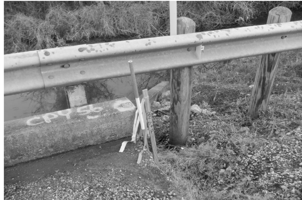
EMBANKMENT EROSION BEHIND NE WINGWALL LOOKING NORTHEAST
