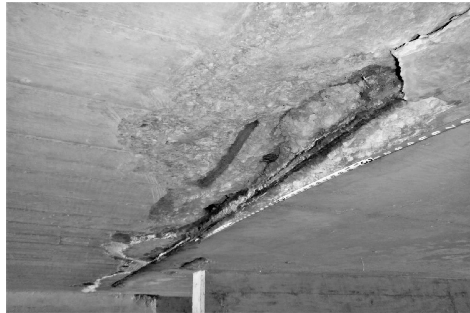
SPALL WITH EXPOSED REBAR ON SLAB SOFFIT IN SPAN 2 LOOKING WEST
