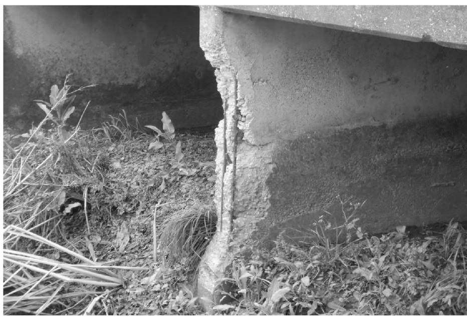
SPALL WITH EXPOSED REBAR AT NORTH END OF INTERMEDIATE WALL 2 FROM WEST LOOKING SOUTHEAST
