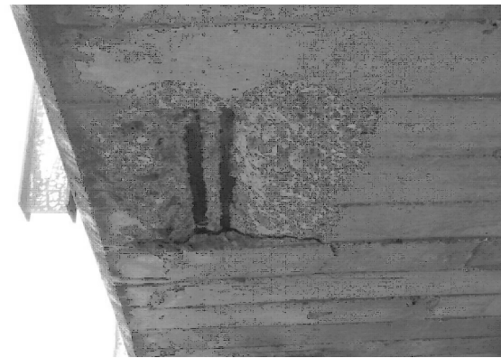
DELAMINATION AND SPALL WITH EXPOSED REBAR ON SLAB SOFFIT IN SPAN 2 AT SOUTH END LOOKING WEST
