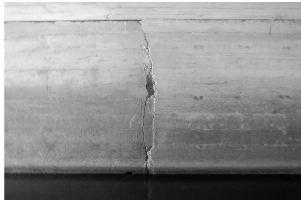
VERTICAL CRACKING ON WEST ABUTMENT WALL LOOKING WEST
