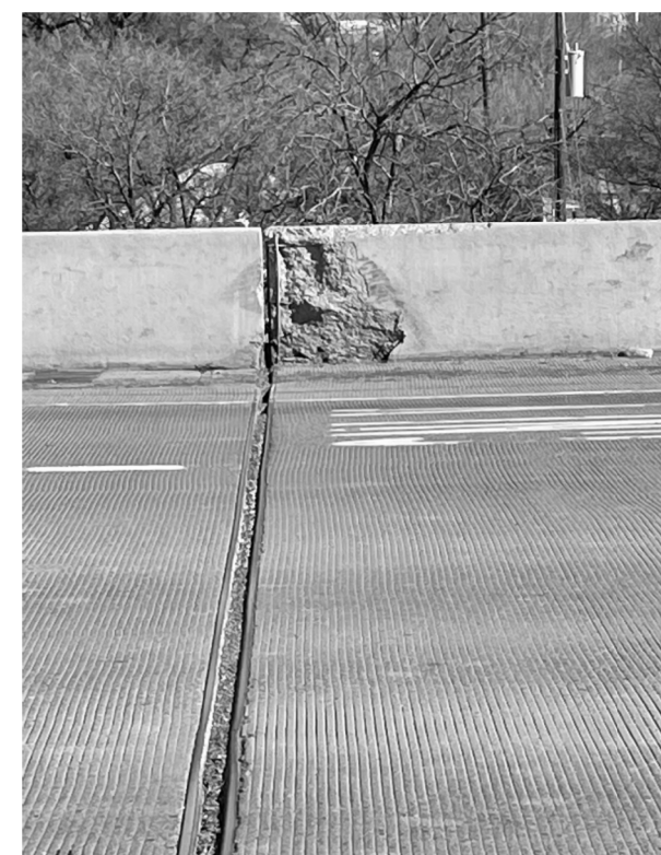
BRIDGE RAIL DAMAGE AT BENT 6 STA. 971+74 FAR INSIDE LANE FACING NORTH PHOTO TAKEN MAY 2022
