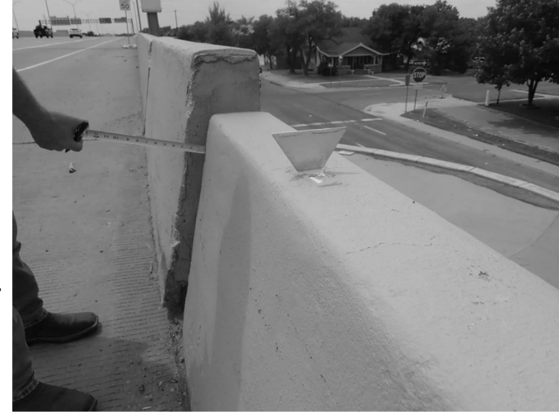
PROTRUDING BRIDGE RAIL ABUTMENT 12 FACING EAST PHOTO TAKEN JULY 2021
