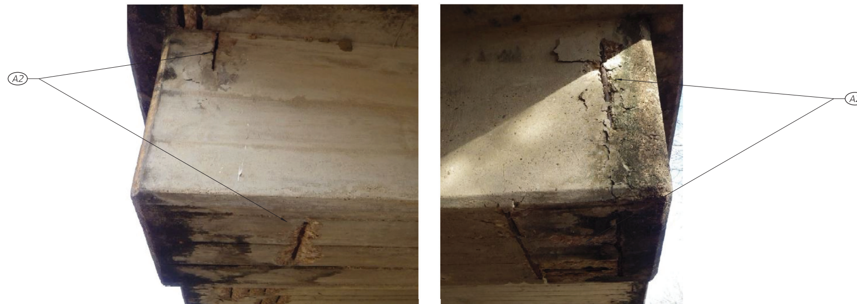
TYPICAL DAMAGE CONDITION AT VARIOUS LOCATIONS
