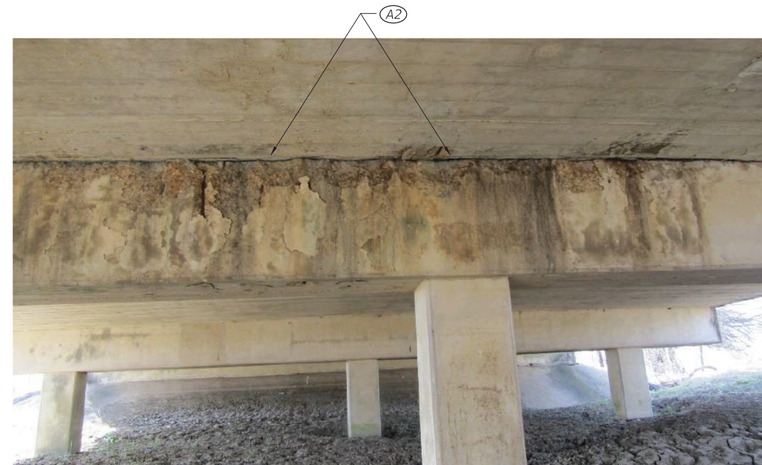
TYPICAL DAMAGE CONDITION AT VARIOUS LOCATIONS
