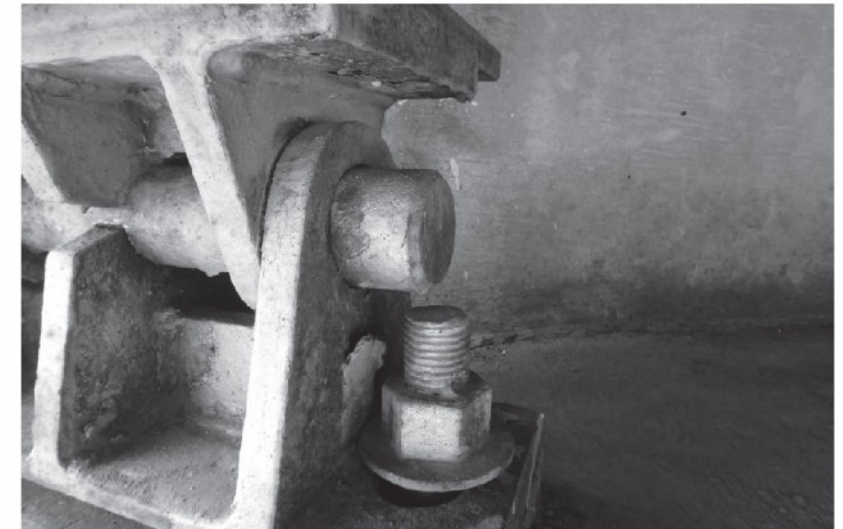
FIGURE 3: MISSING COTTER PIN AT SOUTH BEARING AT WEST ABUTMENT.
