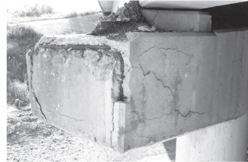
FIGURE 3: MODERATE SPALL IN SOUTH END IN EAST BENT CAP.
