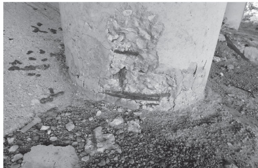
FIGURE 4: MINOR TO MODERATE SPALL IN BASE OF CENTER COLUMN OF WEST BENT.
