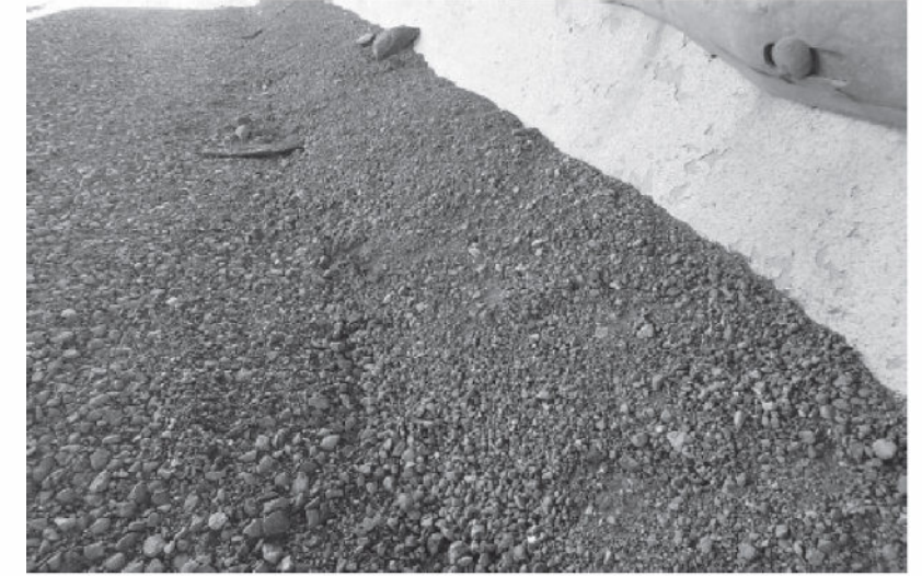
FIGURE 3: EXCESSIVE GRAVEL ACCUMULATION ALONG NW RAIL.
