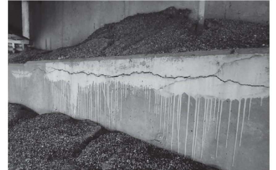
FIGURE 3: TYPICAL MODERATE DELAMINATION CRACKING IN ABUTMENT CAPS.
