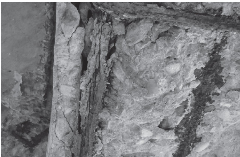
FIGURE 7: HEAVY CORROSION OF MAIN REBAR OF SPALL IN CENTER BENT CAP.
