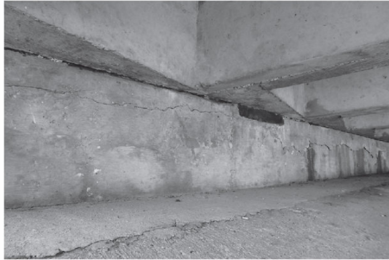
FIGURE 1: TYPICAL MODERATE DELAMINATION CRACKS IN ABUTMENT CAPS. NE CAP SHOWN.
