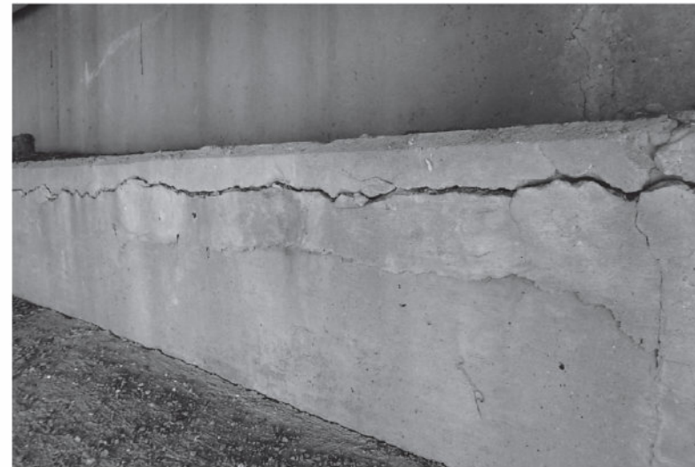
FIGURE 2: TYPICAL MODERATE DELAMINATION CRACKS IN ABUTMENT CAPS, NE CAP SHOWN.
