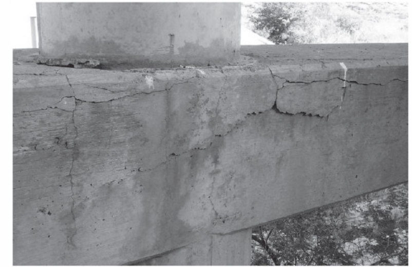
FIGURE 3: MODERATE DELAMINATION CRACKING IN TIE BEAM AT SE BENT - LOOKING NORTH
