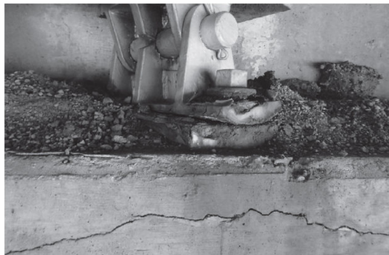
FIGURE 4: EXCESSIVE ASPHALT AROUND CENTER ROCKER BEARING AT WEST ABUTMENT.
