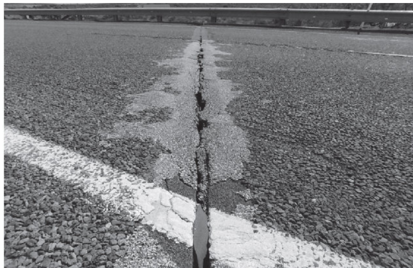
FIGURE 4: PATCHED HEADERS AND FAILED SEALANT AT WEST ABUTMENT JOINT.
