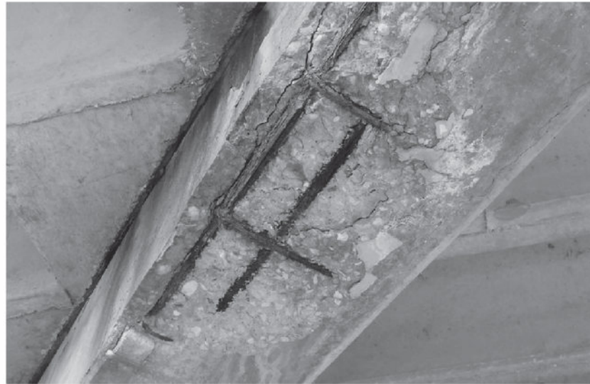
FIGURE 8: HEAVY SPALL WITH EXPOSED AND CORRODED REBAR IN SOFFIT OF NE BENT CAP.
