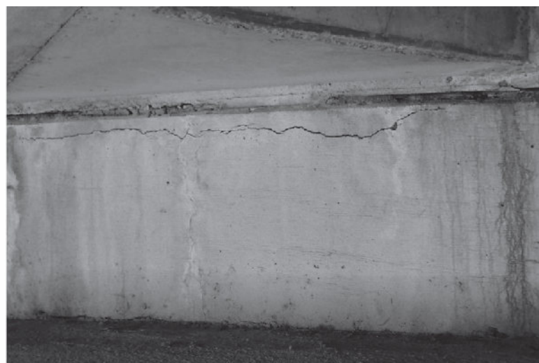
FIGURE 1: MODERATE DELAMINATION CRACK ALONG TOP CORNERS OF SE ABUTMENT CAP.
