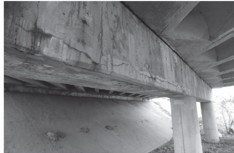
FIGURE 5: TYPICAL MODERATE DELAMINATION CRACKING IN BENT CAPS.
