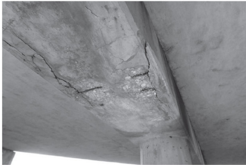
FIGURE 2: SPALL WITH EXPOSED REBAR IN CORNER OF FLAT SLAB AT NORTH END OF SW ABUTMENT.
