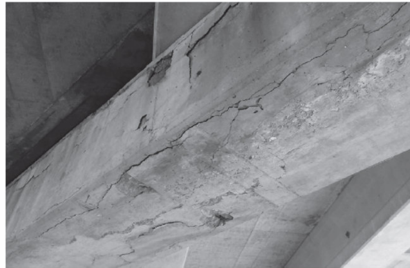
FIGURE 2: HEAVY DELAMINATIONS AND MODERATE SPALLS IN BENT CAP #4.
