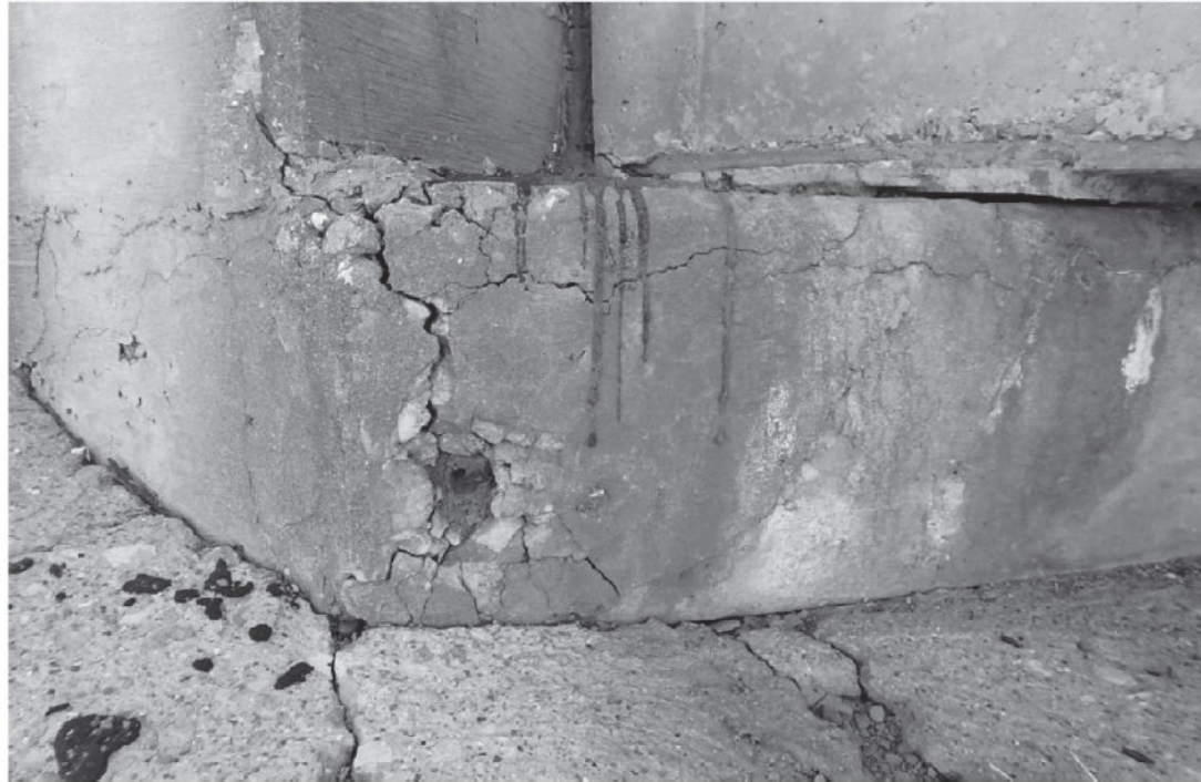
FIGURE 1: MODERATE DELAMINATION CRACKING IN NORTH END OF NE ABUTMENT CAP.
