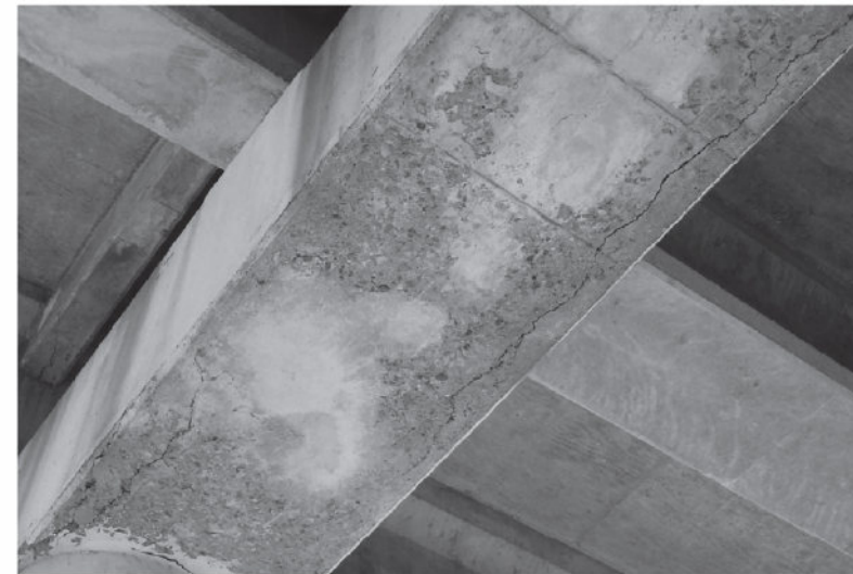
FIGURE 2: MODERATE SCALING AND MODERATE DELAMINATION CRACKS IN SOFFIT OF NE BENT CAP.
