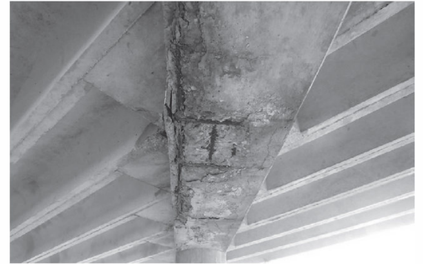
FIGURE 6: HEAVY SPALL WITH EXPOSED AND CORRODED REBAR IN SOFFIT OF CENTER BENT CAP.
