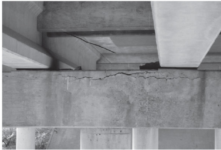
FIGURE 2: MODERATE TO HEAVY DELAMINATION CRACK ALONG TOP NW CORNER OF NW BENT CAP.
