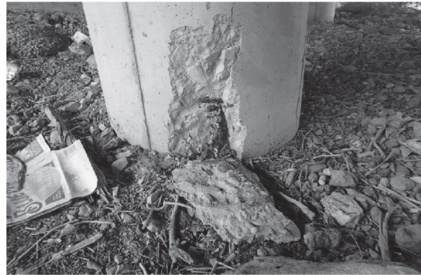
FIGURE 4: MODERATE SPALL IN BASE OF COLUMN 2 FROM SE IN SW BENT.
