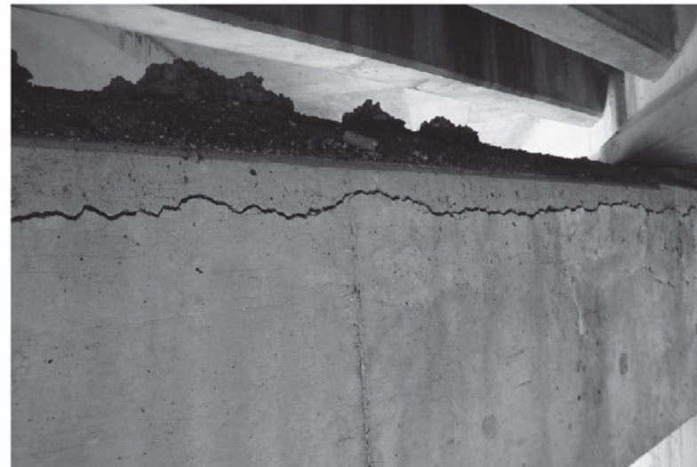
FIGURE 5: TYPICAL MODERATE TO HEAVE DELAMINATION. CRACKING ALONG TOP CORNERS OF BENT CAPS.
