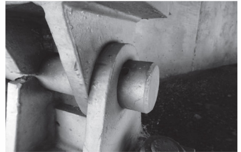
FIGURE 3: MISSING COTTER PIN FOR SE BEARING AT SW ABUTMENT.
