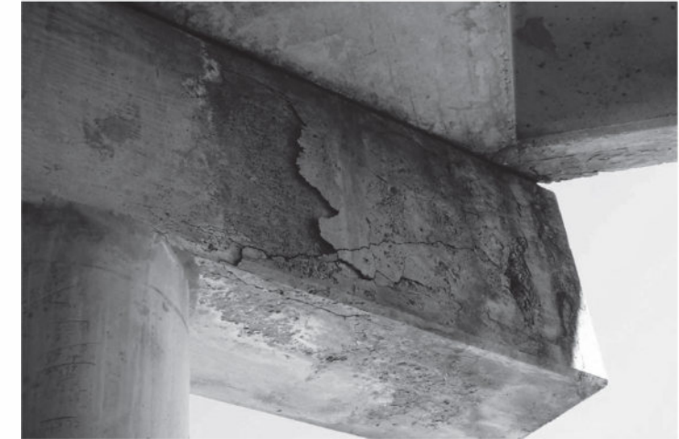
FIGURE 3: MODERATE DELAMINATION IN EAST END OF NW BENT CAP LOOKING NORTH.
