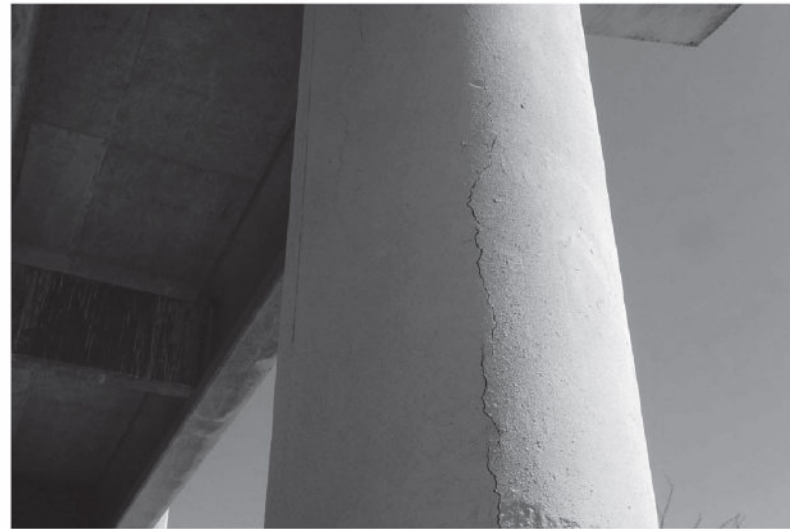
FIGURE 1: MODERATE VERTICAL DELAMINATION CRACKS IN SE COLUMN OF NE BENT.
