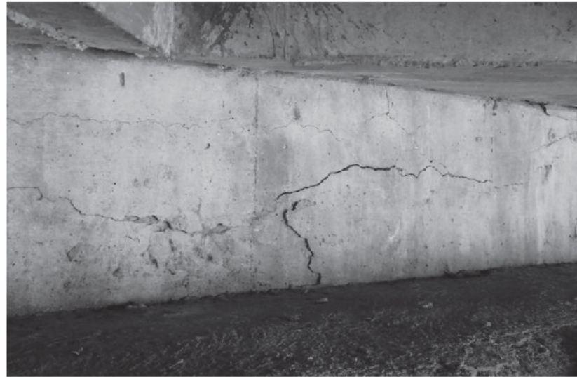
FIGURE 2: TYPICAL MODERATE DELAMINATION CRACKING IN ABUTMENT CAP.
