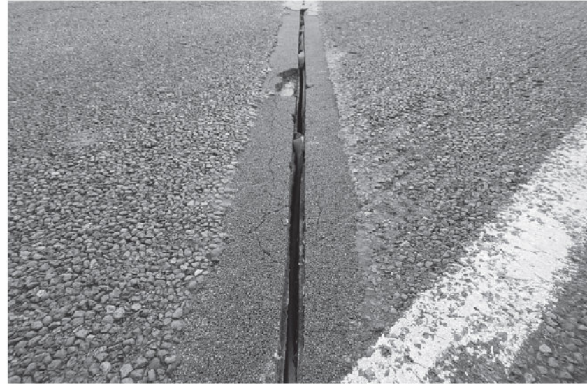
FIGURE 2: FAILED SEALANT IN ABUTMENT JOINTS.
