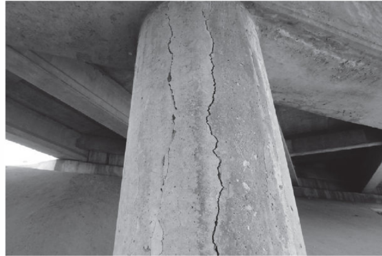
FIGURE 2: MODERATE VERTICAL DELAMINATION CRACKS IN WEST FACE OF CENTER COLUMN AT EAST BENT.
