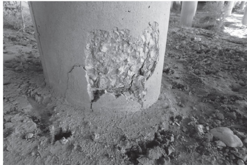
FIGURE 2: SPALL IN BASE OF COLUMN #3 FROM SOUTH IN SW BENT.
