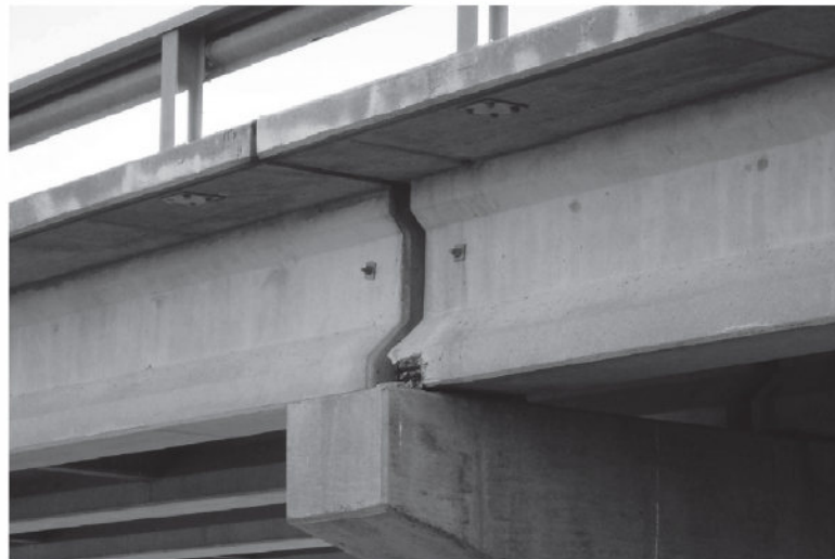
FIGURE 4: MODERATE SPALL WITH EXPOSED STRAND IN NW END OF SW BEAM IN SE SPAN-LOOKING NORTH.
