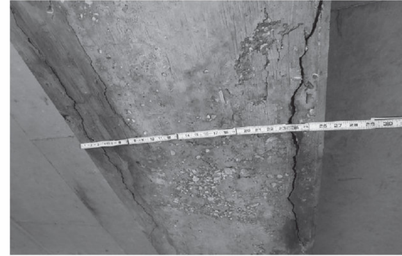
FIGURE 6: TYPICAL SIGNIFICANT DELAMINATION CRACKS IN BOTTOM OF BENT CAPS.
