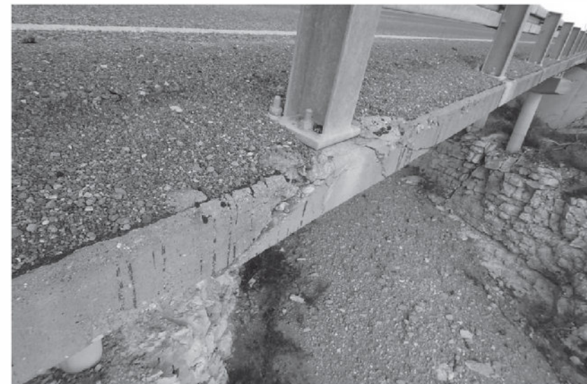
FIGURE 5: MODERATE CRACKS IN SOUTH EDGE OF DECK AT RAIL POST IN CENTER SPAN.
