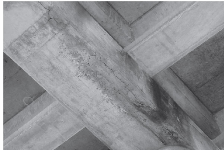
FIGURE 2: MODERATE DELAMINATION CRACK IN SE BOTTOM CORNER OF NW BENT CAP.
