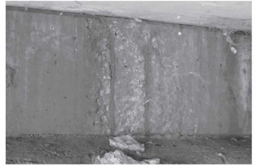
FIGURE 3: SPALL WITH EXPOSED REBAR IN FACE OF SW ABUTMENT CAP.
