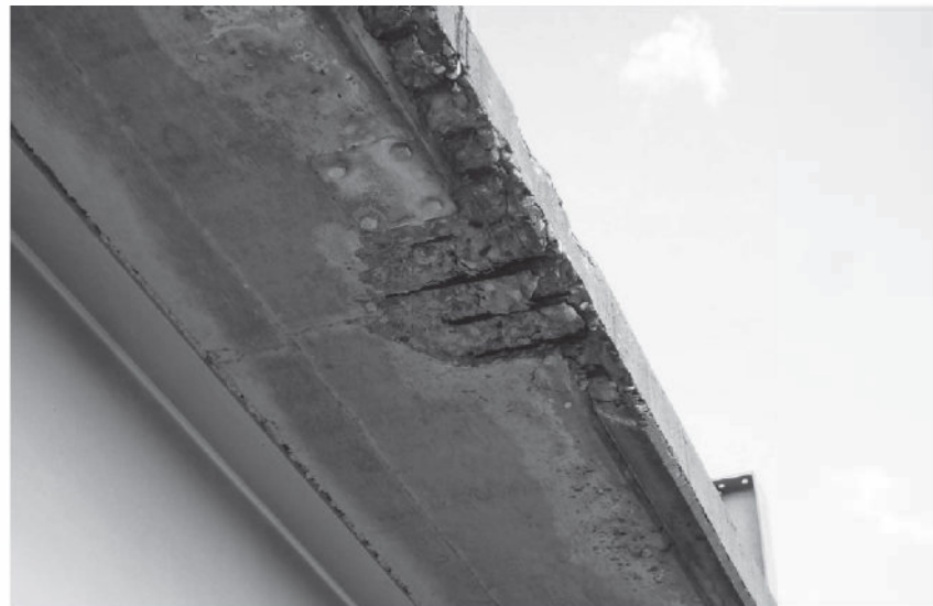
FIGURE 4: MODERATE SPALL WITH EXPOSE REBAR - SOUTH EDGE DECK IN WEST SPAN.
