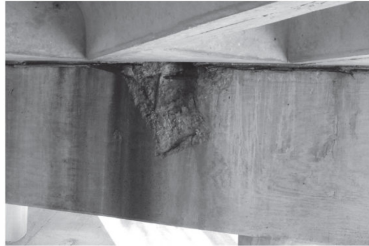
FIGURE 1: MODERATE SPALL IN NW FACE OF NW BENT.
