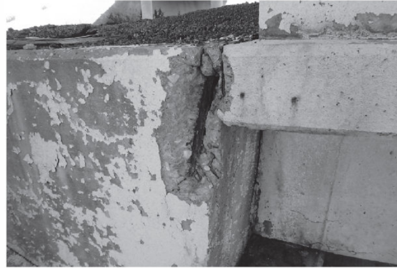
FIGURE 2: MODERATE SPALL IN NORTH END OF NE BACKWALL.
