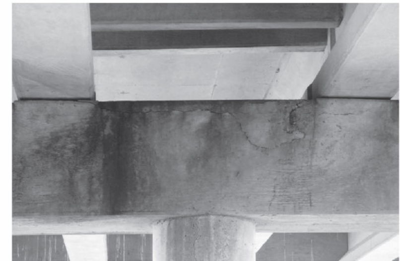
FIGURE 3: MODERATE DELAMINATION CRACK - TOP CORNER OF SE BENT LOOKING NW.
