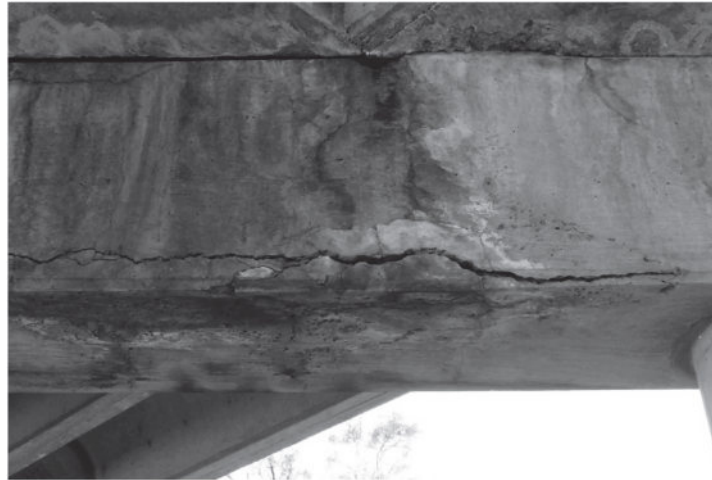
FIGURE 2: TYPICAL HEAVY DELAMINATION CRACK ALONG BOTTOM OF BENT CAPS.
