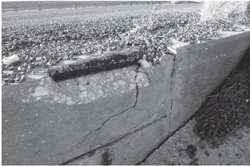
FIGURE 1: TYPICAL SPALLS AND DELAMINATION IN BOTTOM OF BENTS CAPS
