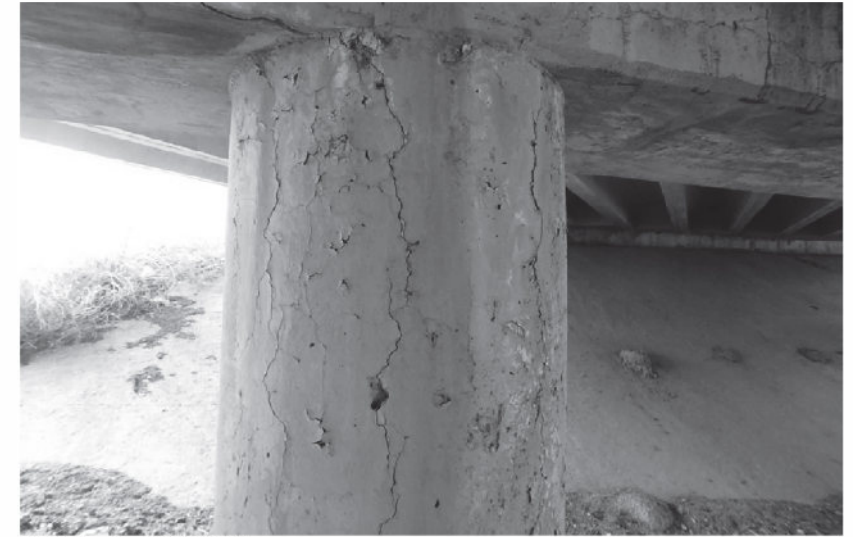
FIGURE 3: MODERATE DELAMINATION CRACKS IN COLUMN 2 FROM SE IN SW BENT.
