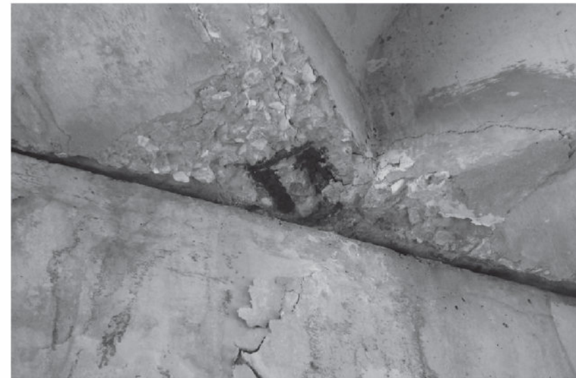
FIGURE 9: TYPICAL MINOR SPALLS WITH EXPOSED REBAR IN BOTTOM OF GIRDERS AT ENDS (ISOLATED).
