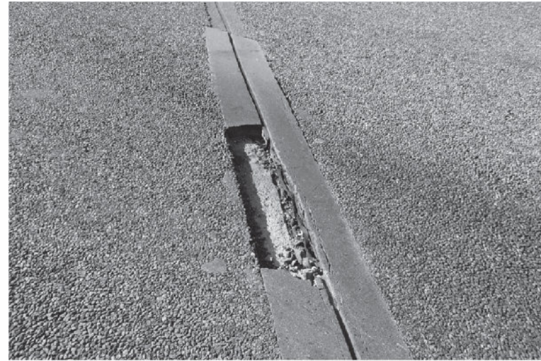
FIGURE 1: MODERATE SPALL IN EPOXY HEADERE AT EAST ABUTMENT JOINT.
