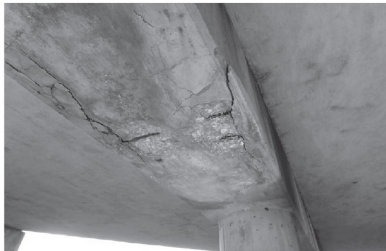
FIGURE 4: TYPICAL SPALLS AND DELAMINATION IN BOTTOM OF BENT CAPS.
