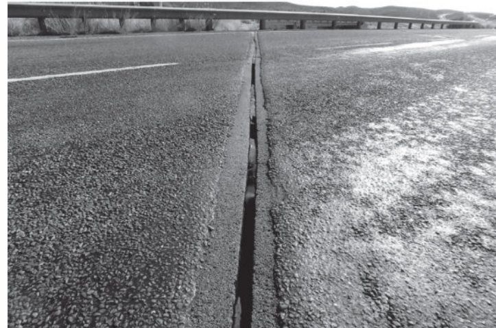
FIGURE 4: LOSS OF SEALANT IN NW ABUTMENT JOINT.
