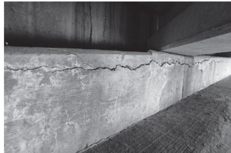
FIGURE 4: MODERATE DELAMINATION CRACK ALONG TOP CORNER- WEST ABUTMENT CAP.
