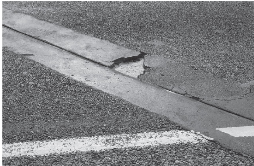
FIGURE 1: SPALL IN EPOXY HEADER AT NE ABUTMENT JOINT.
