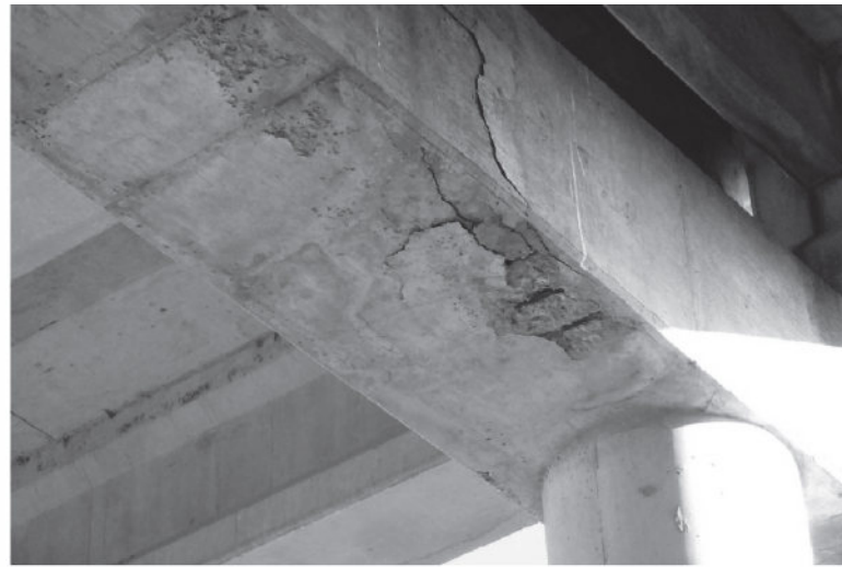
FIGURE 1: MODERATE SPALL IN SOFFIT OF SE BENT CAP.
