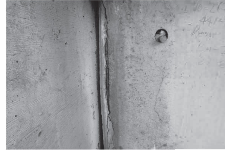
FIGURE 2: MINOR DELAMINATION/SPALL IN END OF NW BEAM AT NE ABUTMENT.
