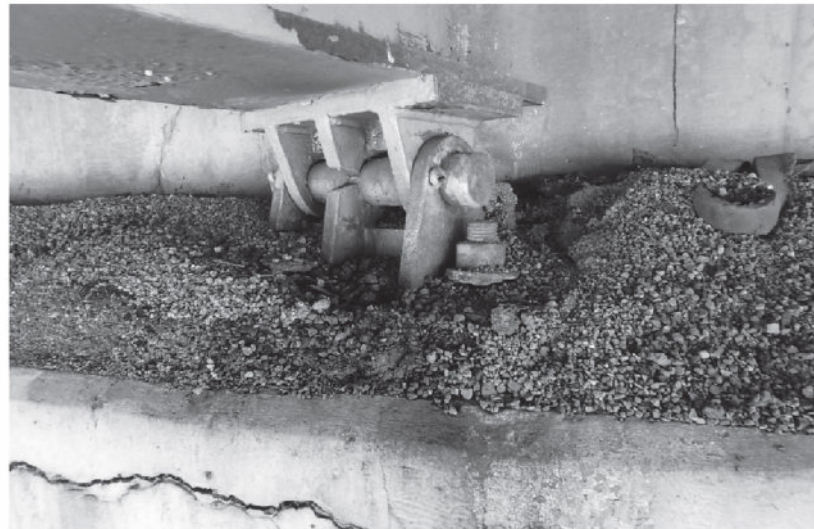
FIGURE 1: EXCESSIVE ASPHALT AROUND CENTER ROCKER BEARING AT WEST ABUTMENT.
