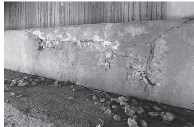
FIGURE 5: MODERATE DELAMINATION CRACKING AND SPALL IN WEST ABUTMENT CAP.
