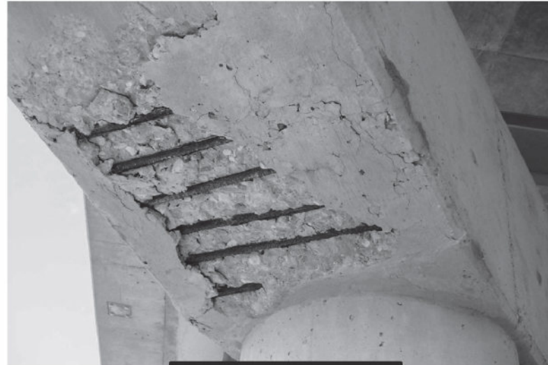
FIGURE 1: MODERATE SPALL WITH EXPOSED STIRRUPS IN SOFFIT OF NW END OF NE BENT CAP - LOOKING EAST
