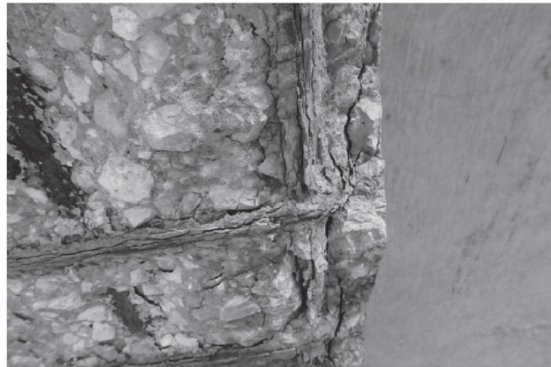
FIGURE 1: CORRODED REBAR IN SOFFIT OF NE BENT CAP.
