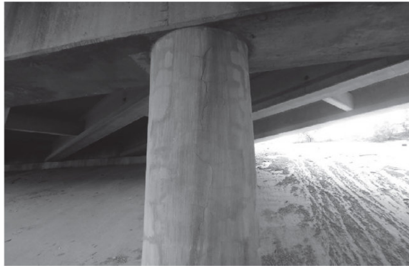
FIGURE 1: PATCHED CENTER COLUMN OF EAST BENT - LOOKING EAST.
