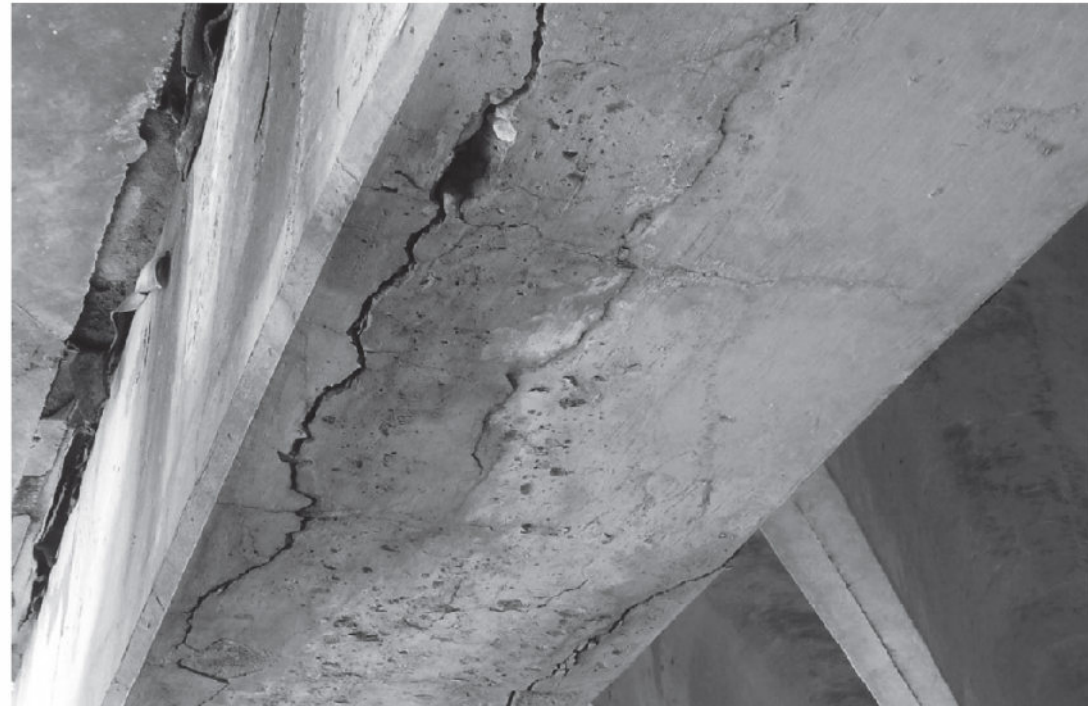
FIGURE 2: TYPICAL MODERATE TO HEAVY DELAMINATION CRACKING ALONG BOTTOM CORNERS OF BENT CAPS.
