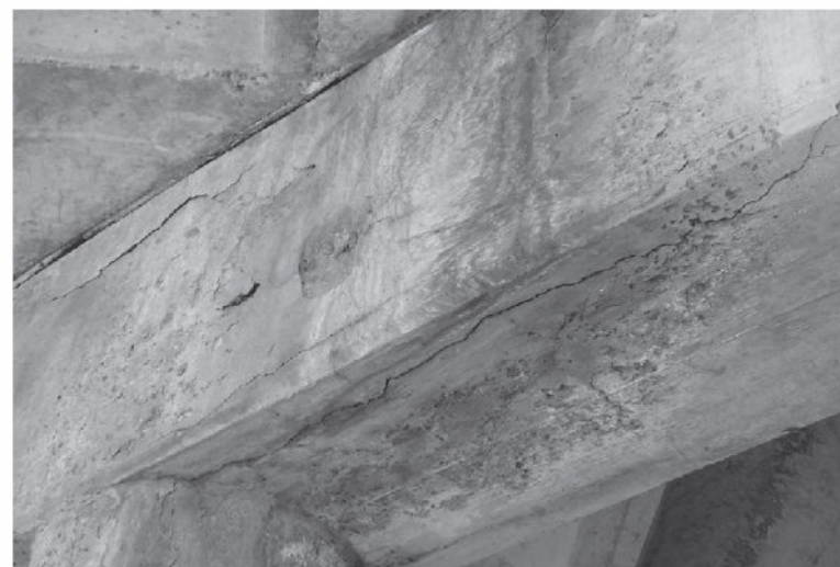
FIGURE 2: MODERATE DELAMINATION CRACKS AND HEAVY SCALING IN EAST END OF SE BENT CAP.
