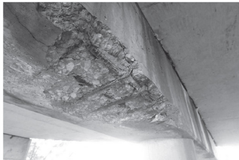
FIGURE 4: MODERATE SPALL WITH EXPOSED AND CORRODED REBAR IN SOFFIT OF NE BENT CAP.
