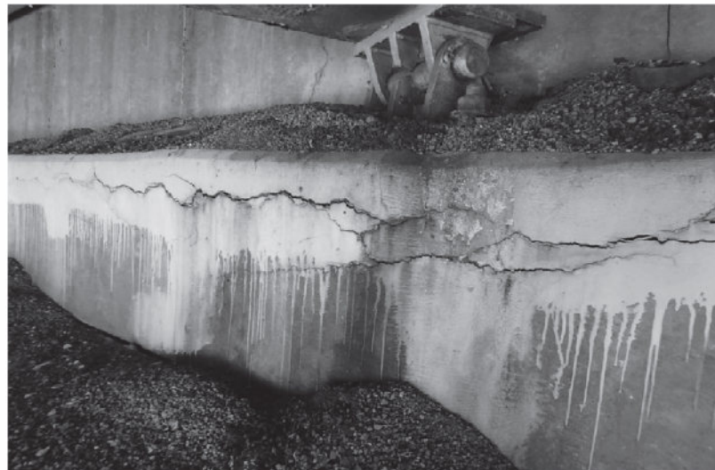
FIGURE 2: MODERATE DELAMINATION CRACKS ALONG TOP CORNER OF WEST ABUTMENT CAP. SIMILAR FOR EAST ABUTMENT CAP.
