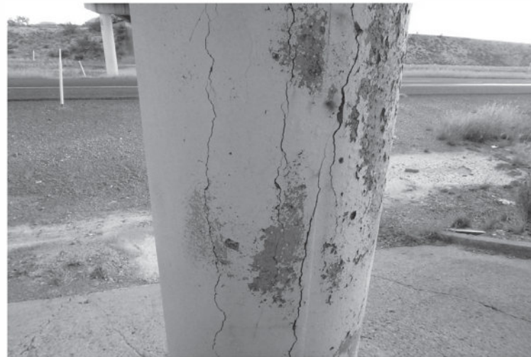
FIGURE 1: MODERATE VERTICAL DELAMINATION CRACKS IN NW COLUMN OF NE BENT-LOOKING SW.
