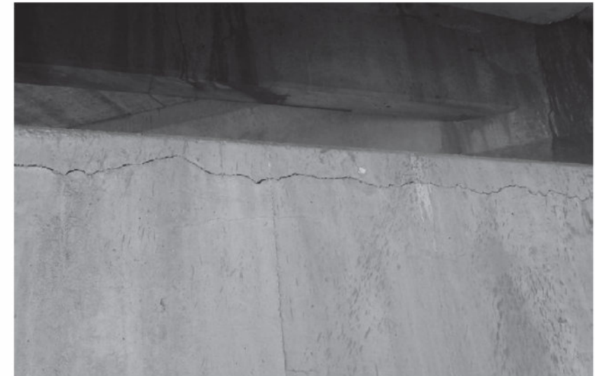
FIGURE 3: TYPICAL MODERATE CRACK ALONG TOP CORNERS OF BENT CAPS.
