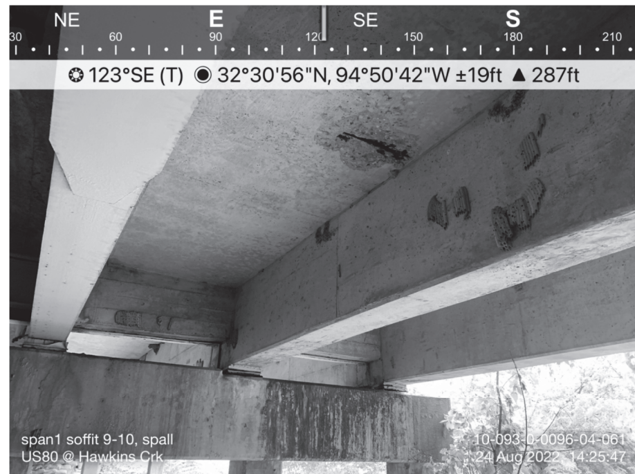
SPALLING IN DECK SOFFIT
