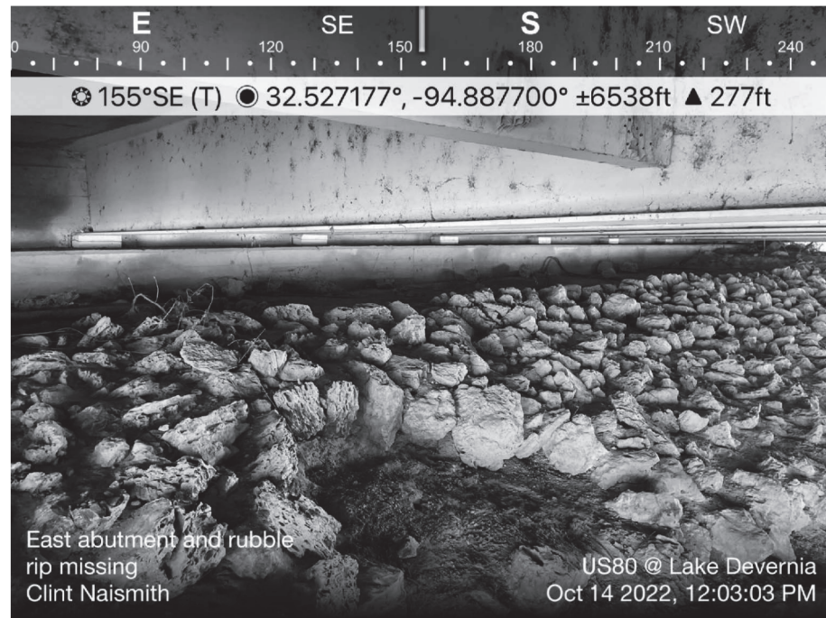
EROSION AT NORTH-EAST ABUTMENT
