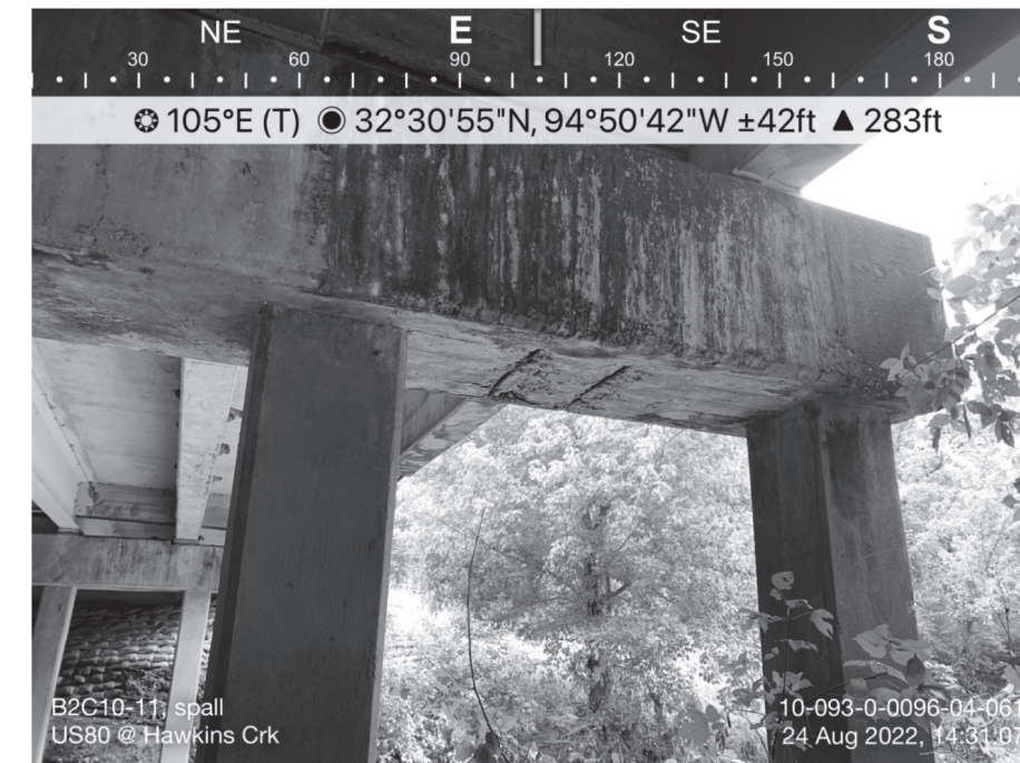
SPALLING IN BENT CAP SOFFIT
