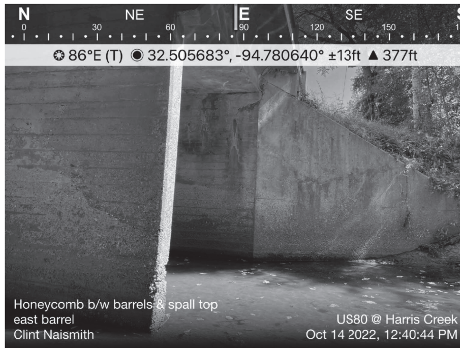
DETERIORATING CONCRETE AT SOUTH END OF CULVERT
