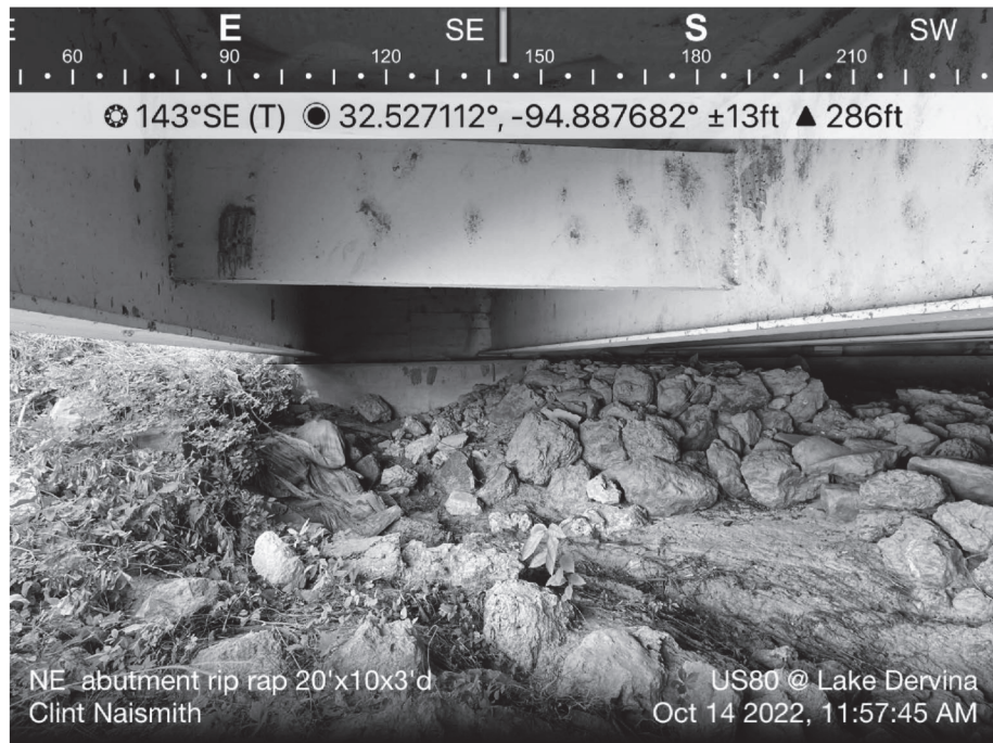
EROSION AT NORTH-EAST ABUTMENT
