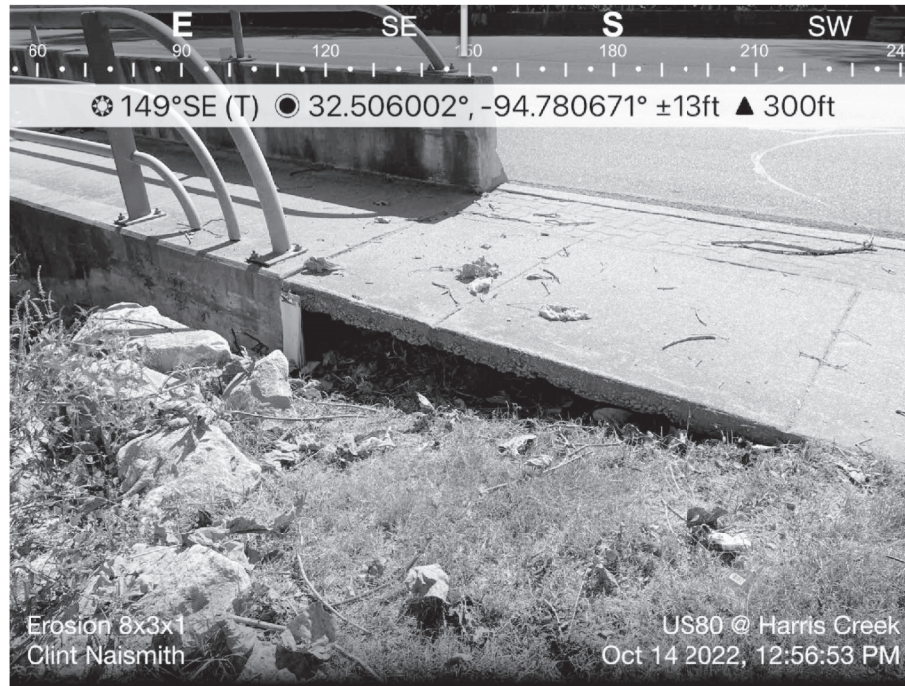
UNDERMINING AT NORTH-WEST CORNER SIDEWALK
