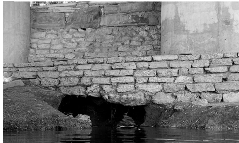
UNDERMINING AT THE RETAINING WALL AT ABUTMENT 1 EMBANKMENT ①②③④
