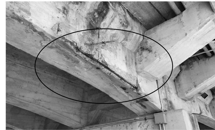
GIRDER E, BENT 1, LOWER EAST EDGE, EXTENSIVE SPALLING WITH UP TO 100% SECTION LOSS IN EXPOSED SHEAR AND LONGITUDINAL REINFORCING
