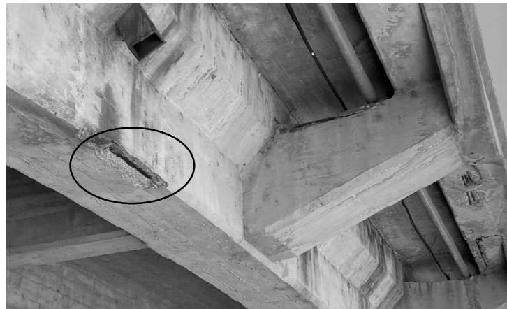
EAST FASCIA, SPALLING ON GIRDER E, CANTILEVER BEAM, AND WEST FASCIA BEAM AT SPAN 3
