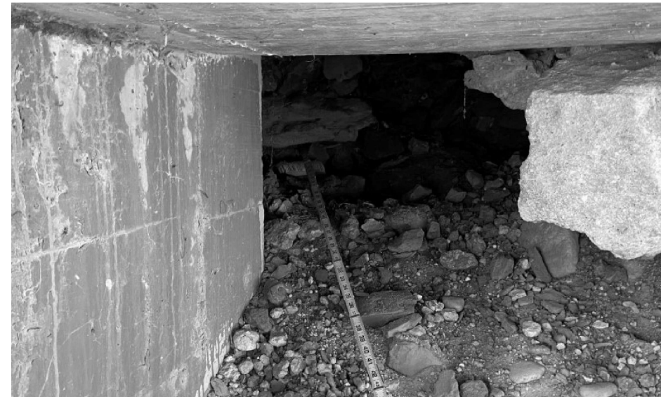
UNDERMINING AT ABUTMENT 2 COLUMN 3 BACKWALL ①②④
