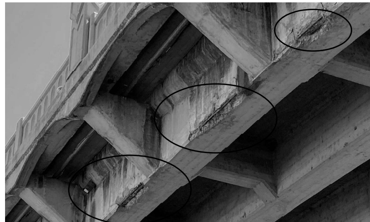
GIRDER E, SPAN 8, EXTENSIVE SPALLING ALONG THE BOTTOM EAST EDGE WITH EXTENSIVE CONCRETE SPALLING AND EXPOSED REINFORCING STEEL
