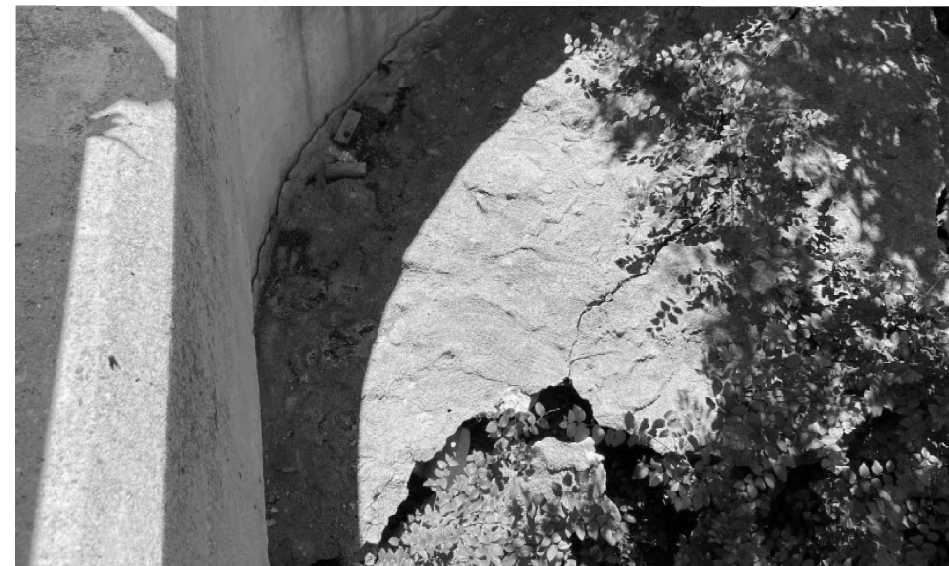
UNDERMINING AT THE ABUTMENT 2 EMBANKMENT ①②③④
