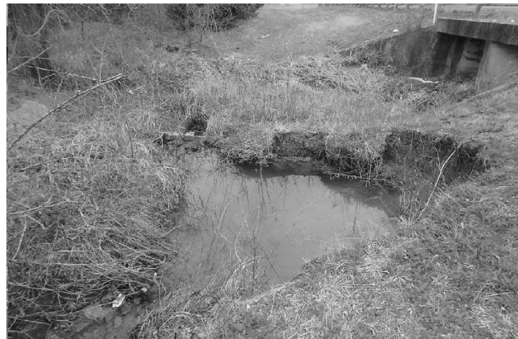
NORTH OF CULVERT LOOKING EAST NW DRAINAGE DITCH SCOUR (20' FROM CHANNEL BED) (TRAPEZOIDAL SHAPE BOTTOM BASE WIDTH 29', TOP WIDTH 16.5', HEIGHT 10', & AVG DEPTH 1')
