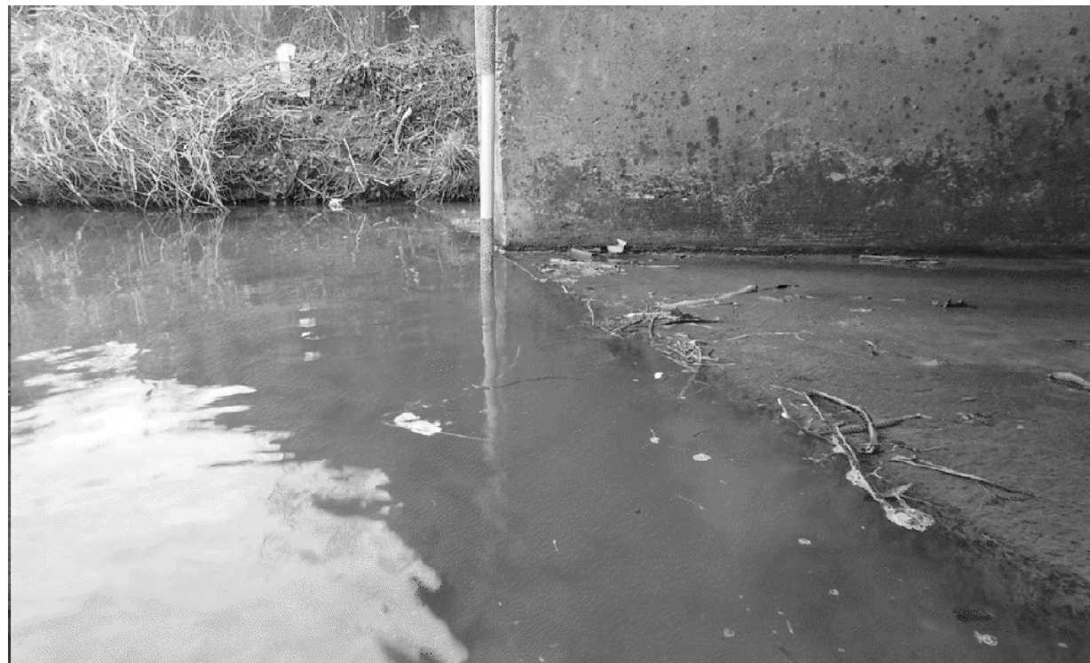
NORTH OF CULVERT LOOKING EAST US CULVERT TOE WALL IS EXPOSED (SCOUR) (1.5')
