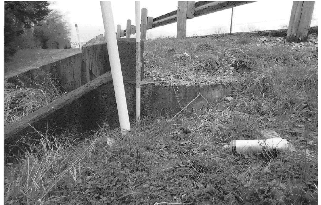
SOUTH SIDE OF CULVERT LOOKING WEST RUNOFF EROSION AT SE BR CORNER (1')
