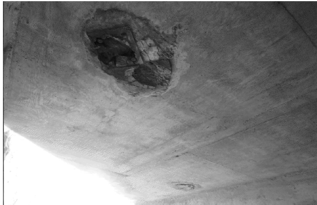
WEST BARREL TOP SLAB AT NORTH END SPALLS/PATCH ON SLAB (APPROXIMATELY 3 SY)
