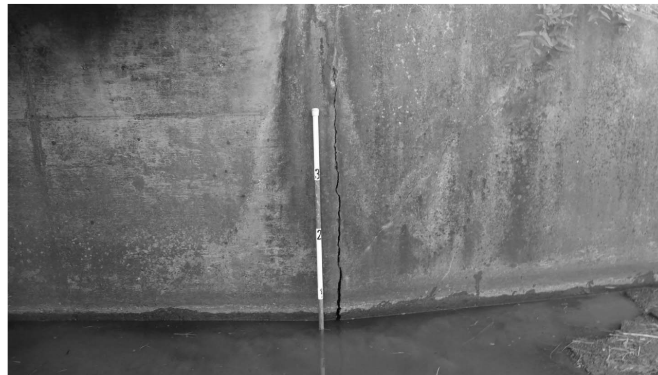
CRACKING IN WINGWALL - LOOKING SOUTHWEST
