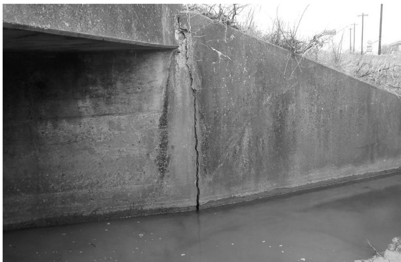
NW WINGWALL HAS A 3/4" WIDE FULL HEIGHT CRACK NEAR CONNECTION WITH ABUTMENT WALL
