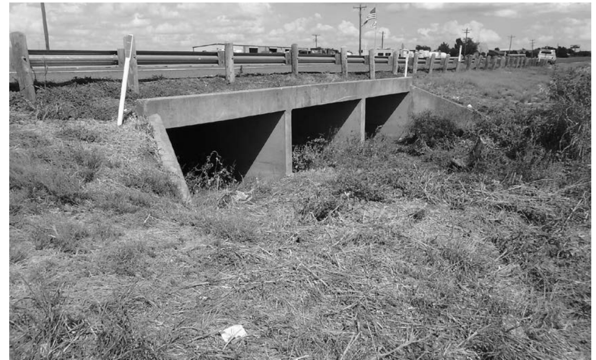
SEDIMENT BUILDUP IN BARRELL - LOOKING NORTH
