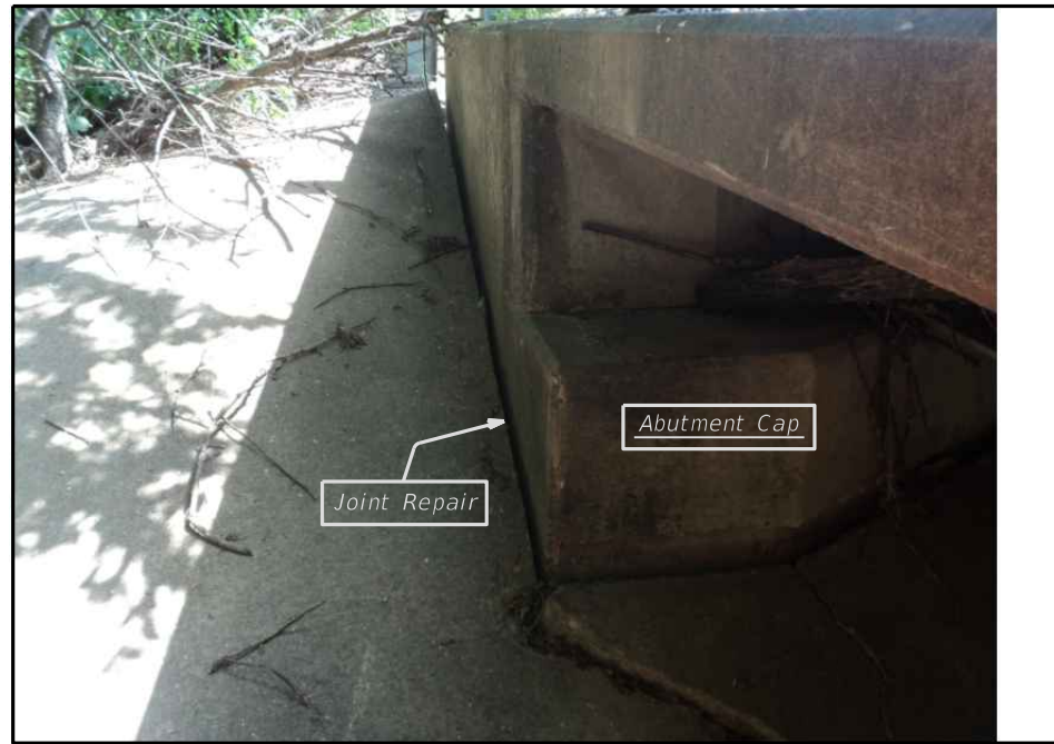
JOINT REPAIR AT EXISTING WINGWALLS SHOWING GAP BETWEEN RIPRAP AND WINGWALL
