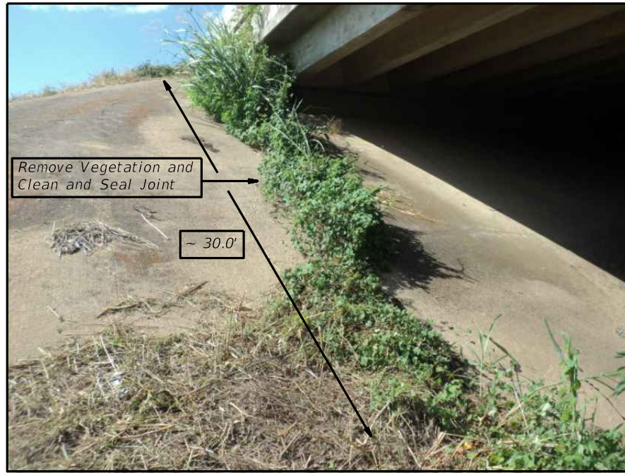
RIPRAP JOINT REPAIR SHOWING LIMITS OF VEGETATION ALONG RIPRAP
