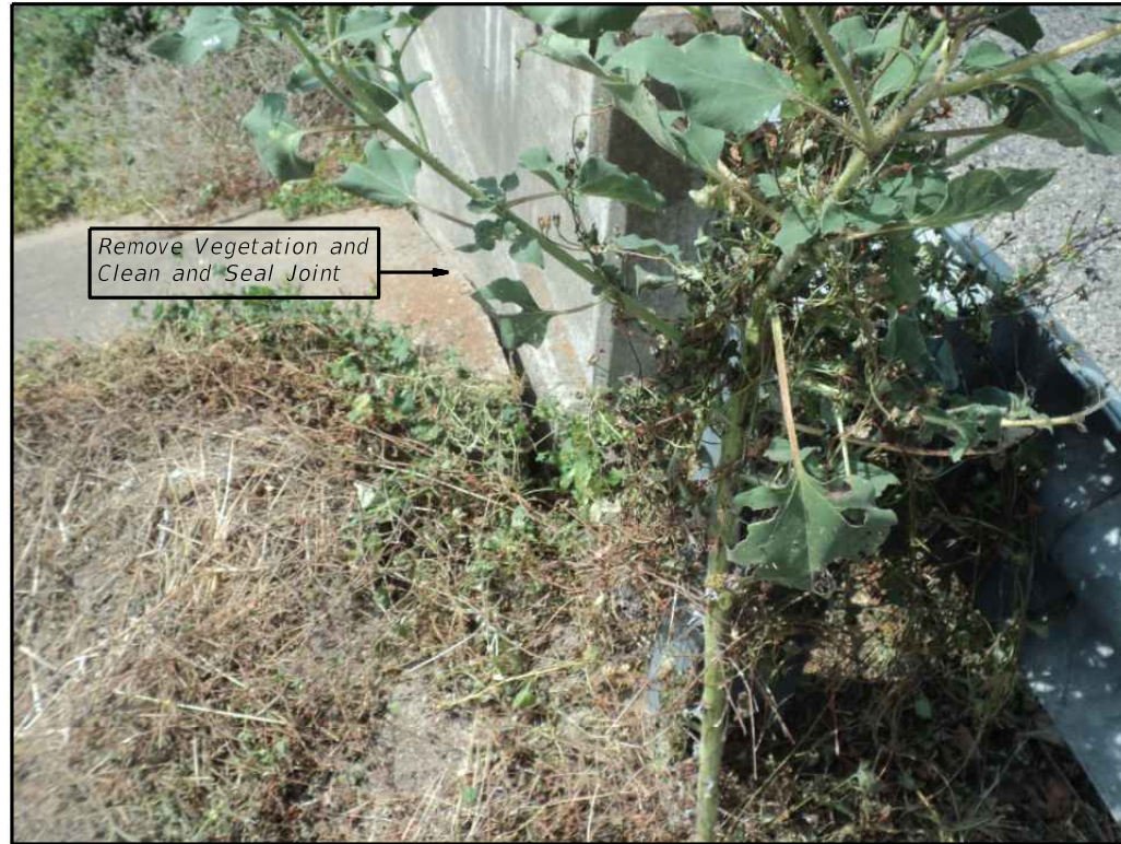
JOINT REPAIR AT EXISTING WINGWALLS SHOWING GAP BETWEEN RIPRAP AND WINGWALLS
