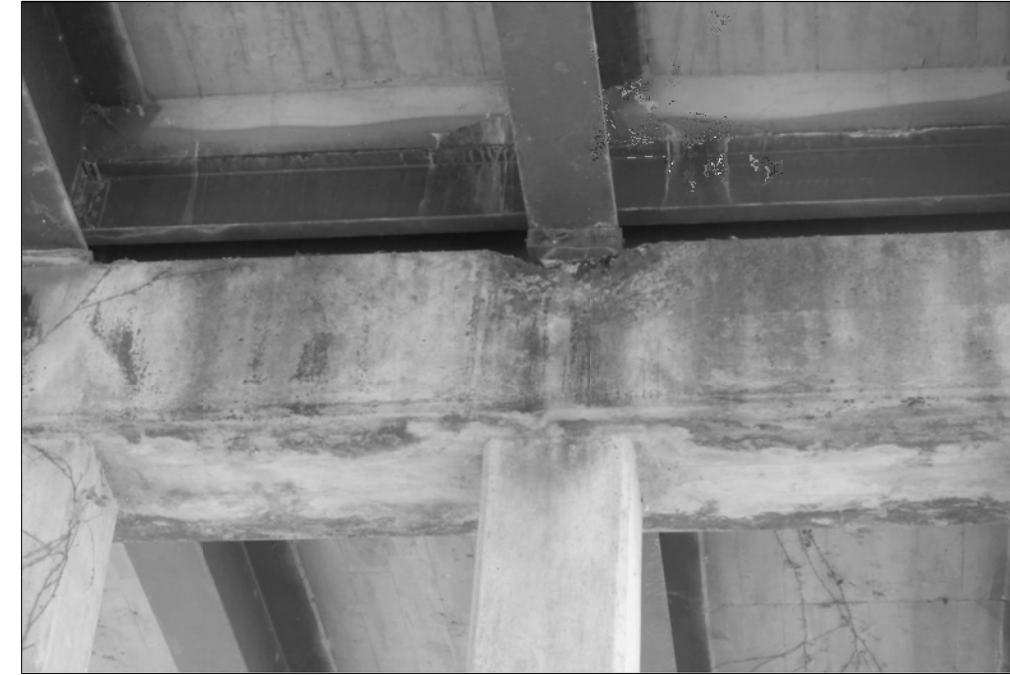
US 87 AT GUADALUPE RIVER - SPALL WITH EXPOSED REBAR ON TOP OF BENT CAP 15 UNDER AN INTERIOR BEAM LOOKING SOUTHWEST. SITE CONDITIONS AS OF 11/04/2020.
