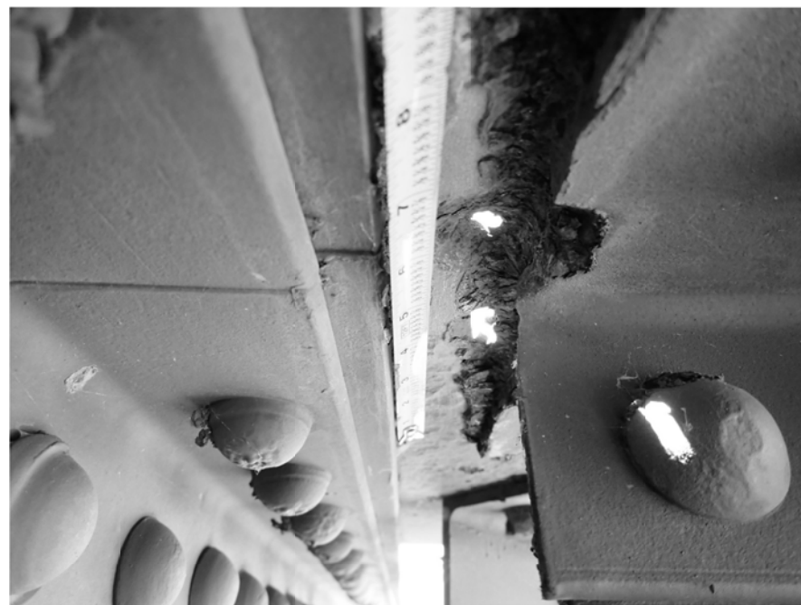
SEVERAL UPPER CHORD GUSSET PLATES WITH HEAVY RUST AND CORROSION HOLES. SITE CONDITIONS AS OF 04/16/2020.
