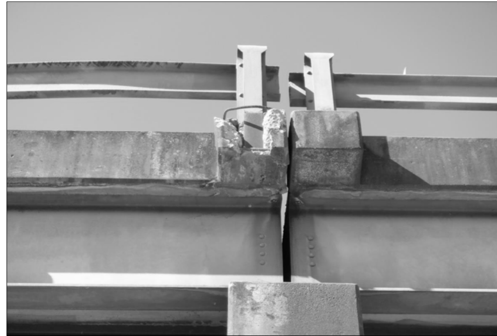
IMPACT DAMAGE TO CONCRETE AND STEEL SE RAILING POST OVER BENT 13 LOOKING NORTHWEST. SITE CONDITIONS AS OF 11/04/2020
