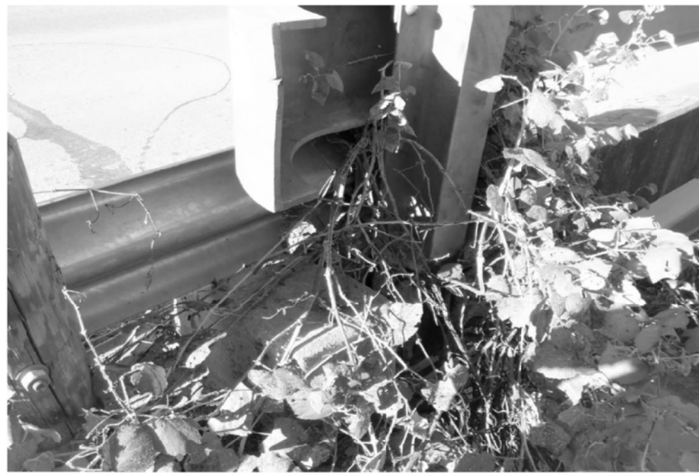
US 77 - SOUTHWEST CORNER CONCRETE FOOTING RAIL. SITE CONDITIONS AS OF 11/04/2020.
