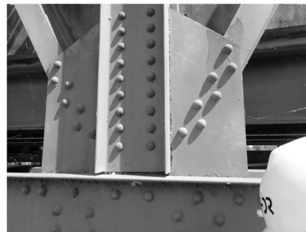
DETERIORATION AT L5 GUSSET. SITE CONDITIONS AS OF 04/16/2020.
