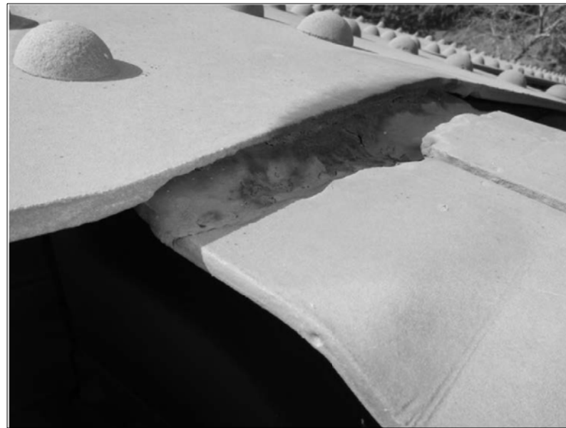
UP TO 1/4" DEEP BY FULL WIDTH PITTING TO UPPER CONNECTION PLATE AT HORIZONTAL STRUT (EAST TRUSS, U8 LOOKING SOUTH). SITE CONDITIONS AS OF 04/29/2014.
