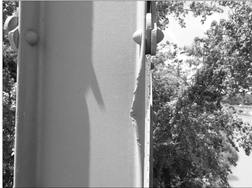
CLOSE-UP OF SECTION LOSS UP AT 1/4" AT UPPER GUSSET PLATE AT THE EXTERIOR GUSSET PLATE/UPPER CHORD CONNECTION, T1 - U4 LOOKING NORTHWEST. SITE CONDITIONS AS OF 04/16/2020.
