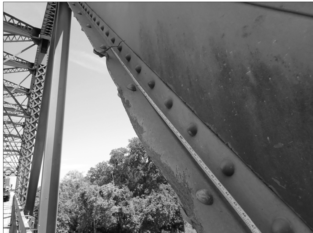
SECTION LOSS UP TO 1/4" AT UPPER GUSSET PLATE AT THE EXTERIOR GUSSET PLATE/UPPER CHORD CONNECTION, T1 - U4 LOOKING NORTHWEST. SITE CONDITIONS AS OF 04/16/2020.
