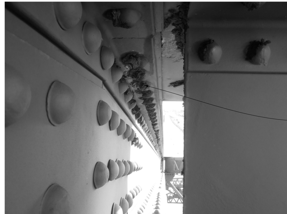
TYPICAL 50% SECTION LOSS TO TOP CHORD RIVET HEADS. SITE CONDITIONS AS OF 04/10/2018.
