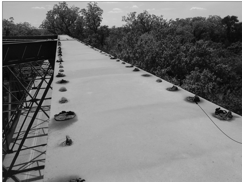
TOPSIDE OF UPPER CHORD WITH UP TO 100% LOSS ON RIVET HEADS. SITE CONDITIONS AS OF 04/16/2020.
