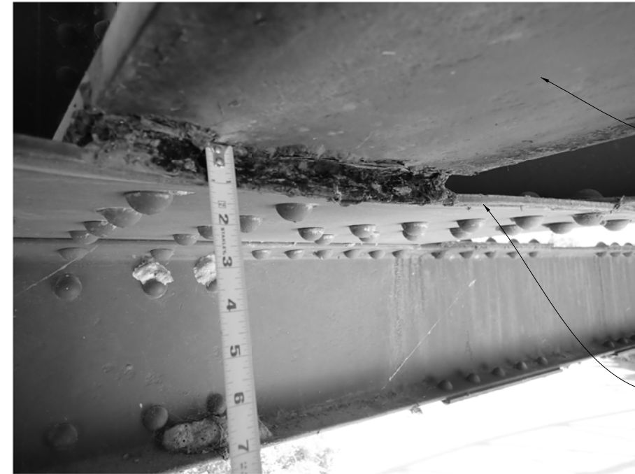
CORROSION UNDER FLOOR BEAM AND BOTTOM GUSSET PLATE (TYPICAL). SITE CONDITIONS AS OF 4/16/2020.
