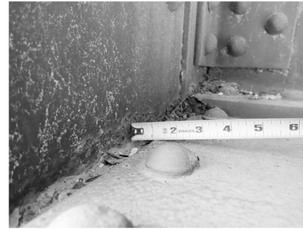
FLOORBEAM 6 AT TRUSS 1, VERTICAL GUSSET PLATE HAS SECTION LOSS WITH 50% SECTION REMAINING. SITE CONDITIONS AS OF 04/16/2020.
