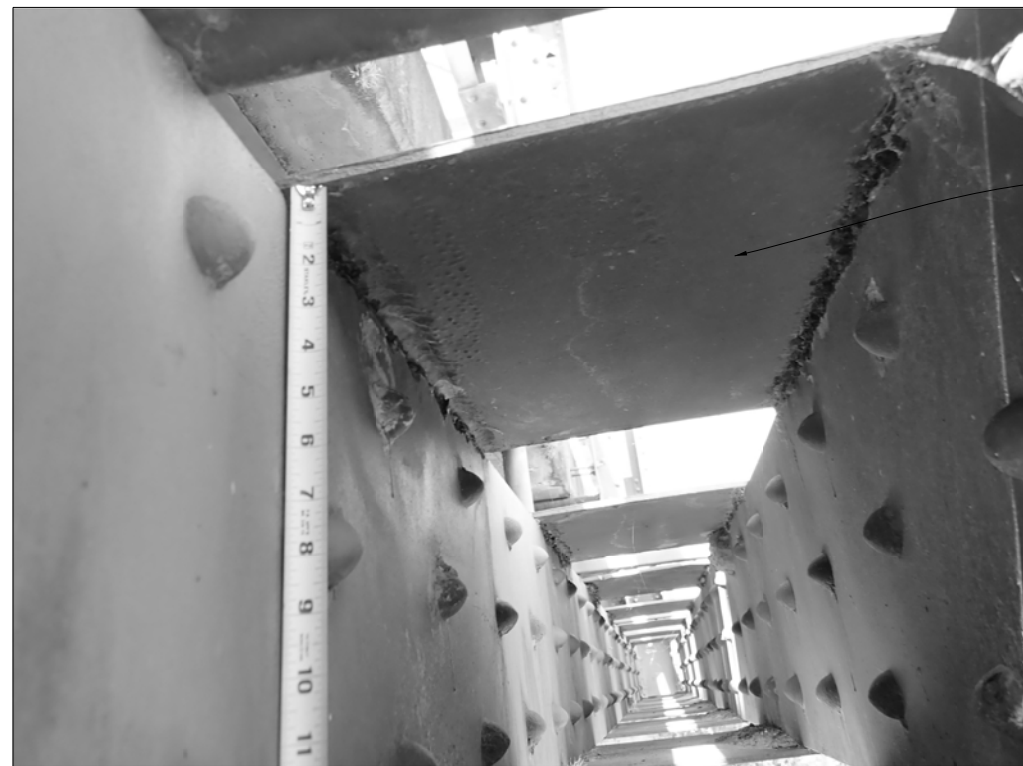
TYPICAL LOWER CHORD BATTEN PLATE SECTION LOSS. SITE CONDITIONS AS OF 04/16/2020.
