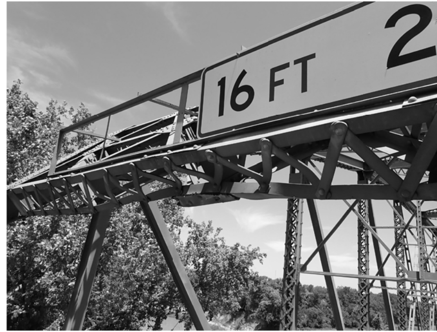
TYPICAL PORTAL FRAME IMPACT DAMAGE. SITE CONDITIONS AS OF 04/16/2020.
