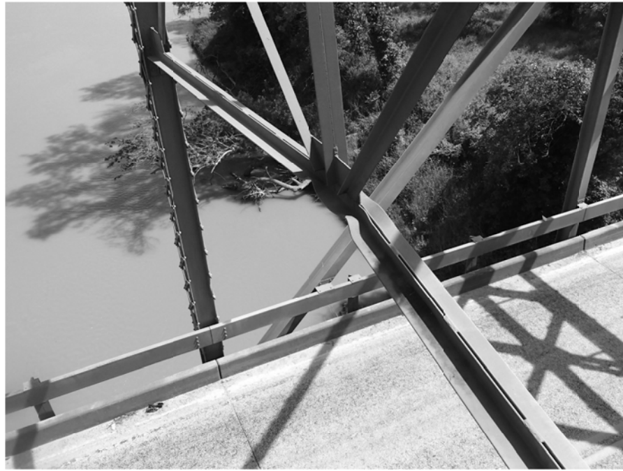
TYPICAL INTERIOR PORTAL FRAME IMPACT DAMAGE. SITE CONDITIONS AS OF 04/16/2020.
