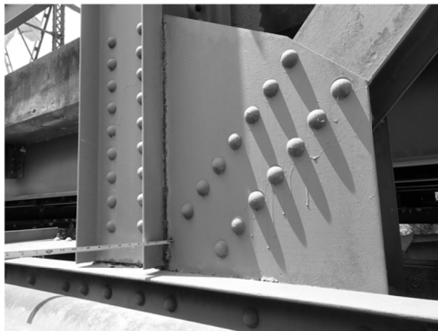
FLOORBEAM 2 AT TRUSS 1, UP TO 1/4" PACK RUST BETWEEN GUSSET PLATES AND EXTERIOR CHANNEL. SITE CONDITIONS AS OF 04/16/2020.
