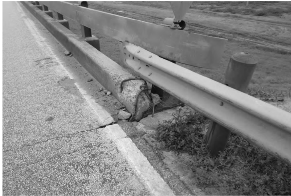
DAMAGE TO SOUTH CORNER CURB LOOKING EAST SITE CONDITIONS AS OF 3/15/2015
