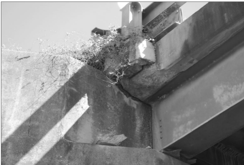
IMPACT SPALL WITH EXPOSED REBAR TO NE END OF NW CONCRETE RAILING POST AND DECK OVERHANG LOOKING EAST. SITE CONDITIONS AS OF 11/04/2020.
