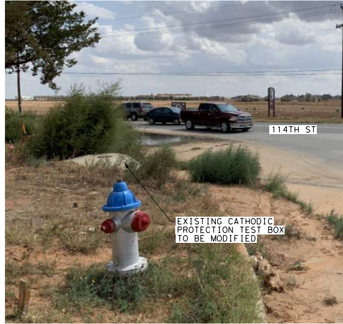
EXISTING CATHODIC PROTECTION STATION AT NE CORNER OF 114TH ST & MEMPHIS AVE LOOKING SE
