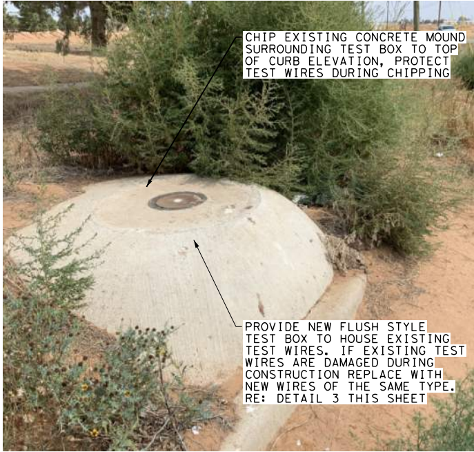
EXISTING CATHODIC PROTECTION TEST BOX MODIFICATION
