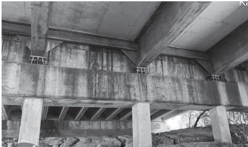
PAINT FAILURE ON STEEL BEAMS, BEARINGS & DIAPHRAGMS
