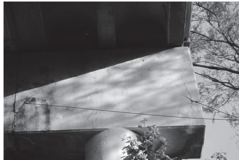
DELAMINATION/CRACK ON SW SIDE OF BENT #10 (LOOKING SE)
