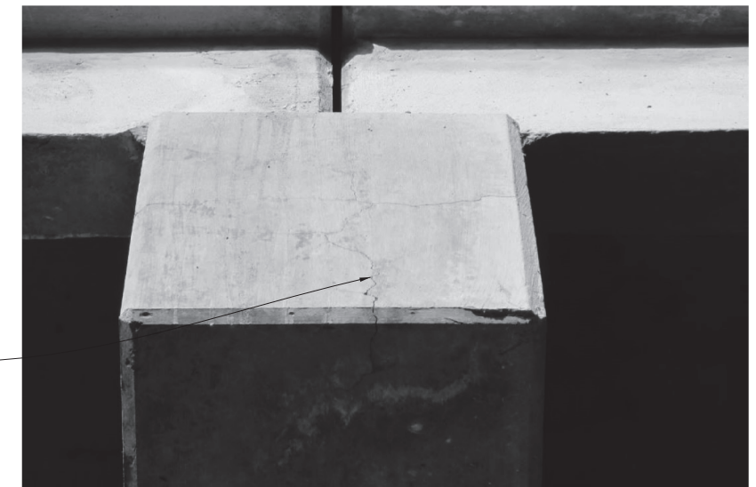
TYPICAL CRACKS ON ENDS OF BENT CAPS
