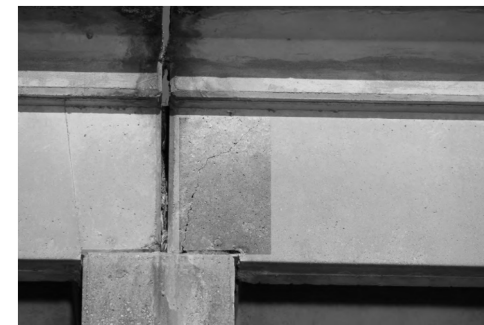
Pan Girder Concrete crack
