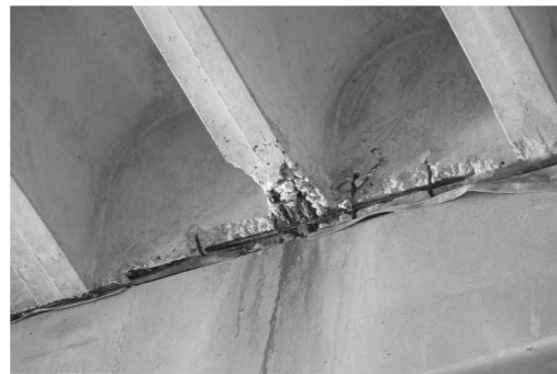
Pan Girder Spall
