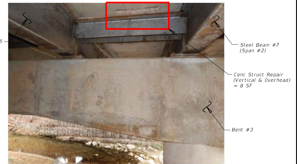
PHOTO #6 (Showing Spall to underside of Bridge Deck)
