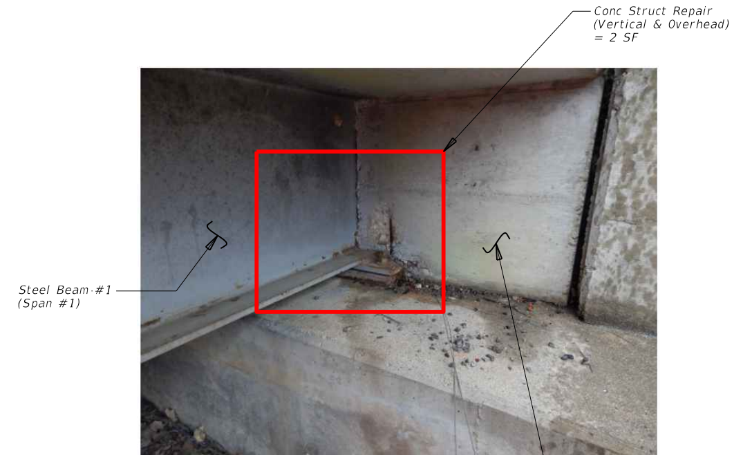
PHOTO #3 (Showing Spall at Backwall at Abutment #1)
