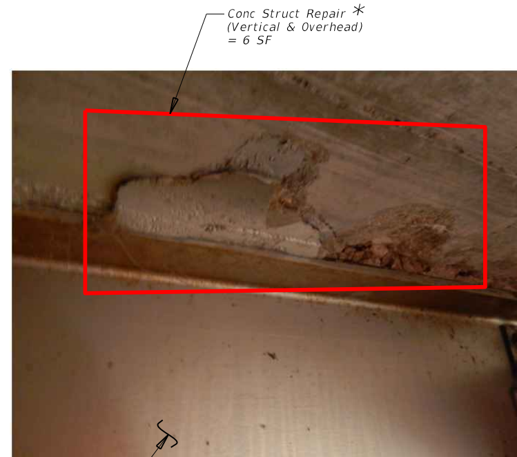
PHOTO #2 (Showing Spall to underside of Bridge Deck)
