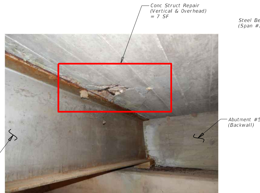
PHOTO #5 (Showing Spall to underside of Bridge Deck)
