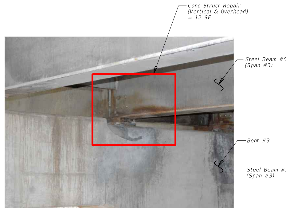
PHOTO #4 (Showing Spall at Cap at Beam 5)
