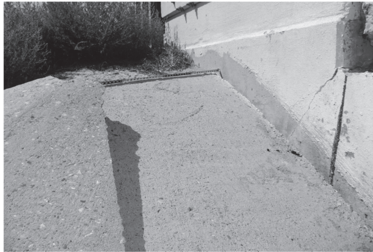
LP 335 NB AT ABANDONED RR RIPRAP HAS SETTLED AND FRACTURED AT SE CORNER
