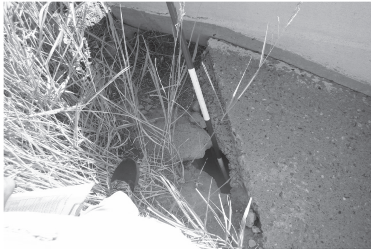
LP 335 NB AT ABANDONED RR EROSION AT TOP EDGE OF RIPRAP AT NW CORNER
