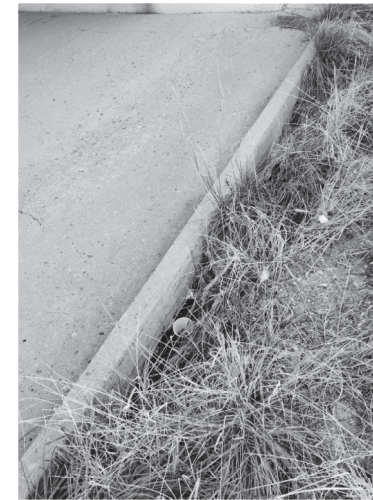
LP 335 WB AT EASTERN ST UNDERMINING EROSION ALONG NW RIPRAP
