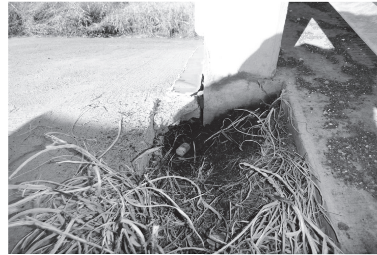
SH 152 EB AT DIXON CREEK EMBANKMENT EROSION AT SW CORNER
