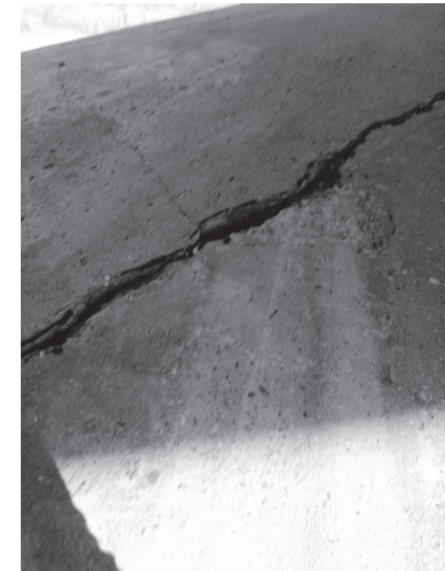
IH-27 NB AT P.D.T FORK RED RIVER EROSION AT ABUTMENT 1
