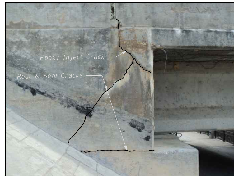
WINGWALL CRACK REPAIR - NW CORNER SHOWING LIMITS OF DIAGONAL CRACKING - LOOKING EAST
