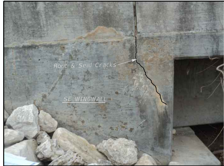
WINGWALL CRACK REPAIR - SE CORNER SHOWING LIMITS OF DIAGONAL CRACKING - LOOKING WEST
