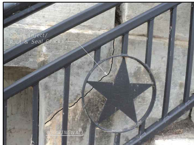
WINGWALL CRACK REPAIR - NE CORNER SHOWING LIMITS OF DIAGONAL CRACKING - LOOKING WEST
