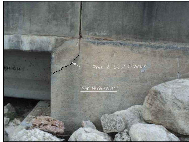
WINGWALL CRACK REPAIR - SW CORNER SHOWING LIMITS OF DIAGONAL CRACKING - LOOKING EAST
