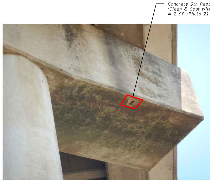
PHOTO 24 Showing Cap Spall at Bent #2
