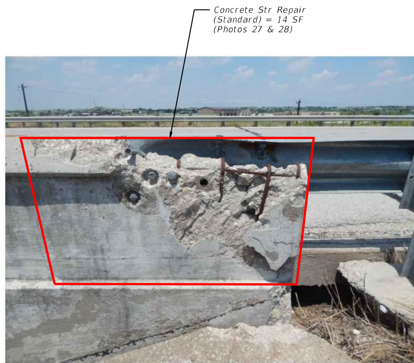
PHOTO 28 Showing Rail Damage (Southwest Wingwall)
