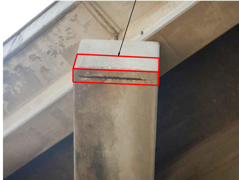
PHOTO 14 Showing Cap Spall at Bent #4 (South End of Cap)
