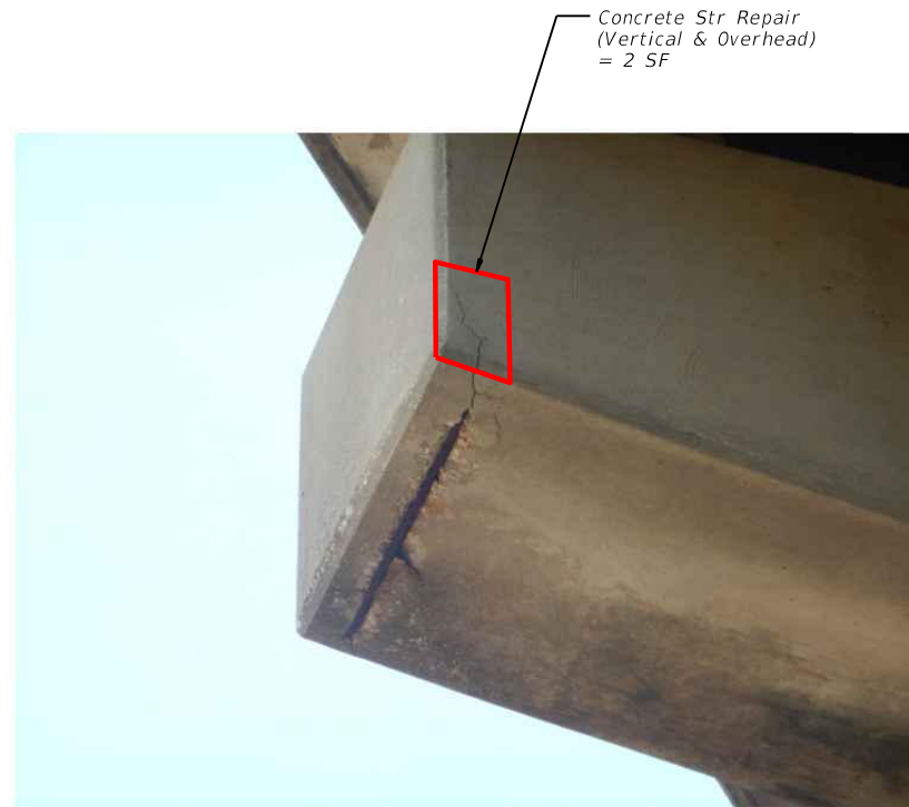
PHOTO 15 Showing Cap Spall at Bent #4 (South End of Cap)
