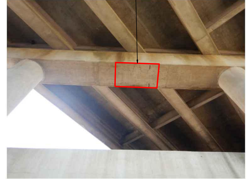
PHOTO 12 Showing Cap Spall at Bent #4
