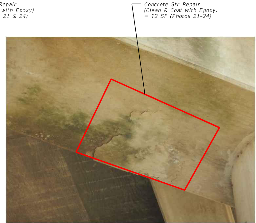
PHOTO 22 Showing Cap Spall at Bent #2
