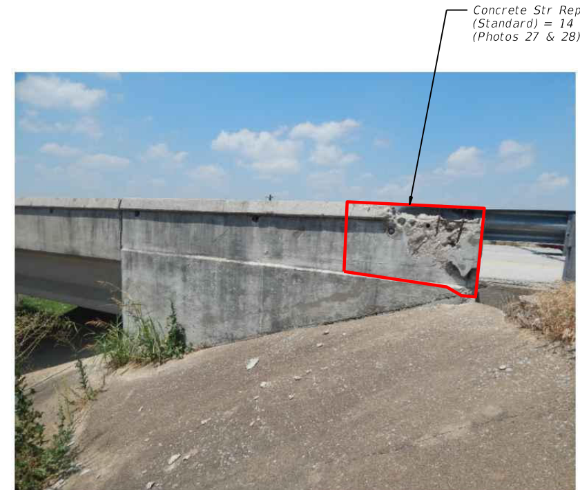
PHOTO 27 Showing Rail Damage (Southwest Wingwall)
