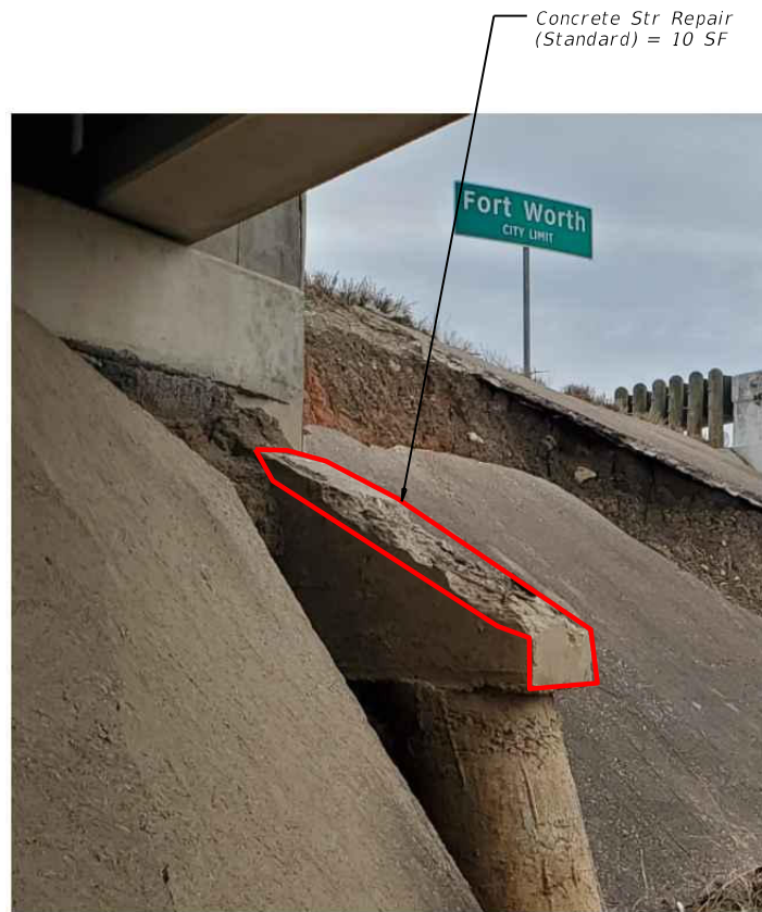
PHOTO 25 Showing Pier Cap Damage at Abutment #5
