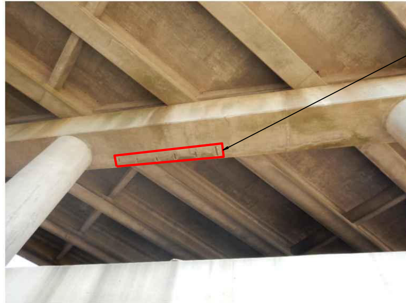
PHOTO 10 Showing Cap Spall at Bent #4
