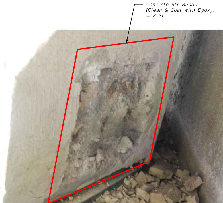
PHOTO 26 Showing Spall at Abutment #5 (End of Beam #5)
