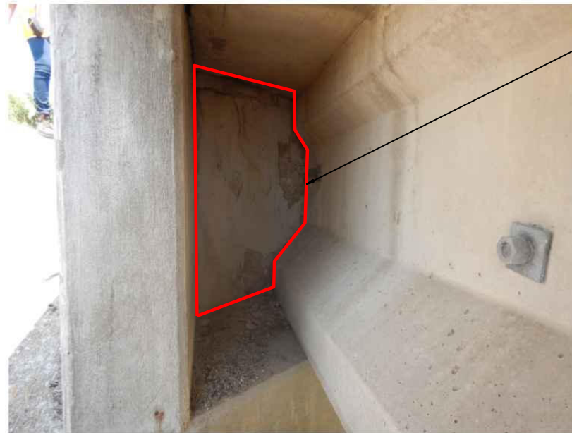
PHOTO 30 Showing Spall at Abutment #1 (West Corner of Backwall)
