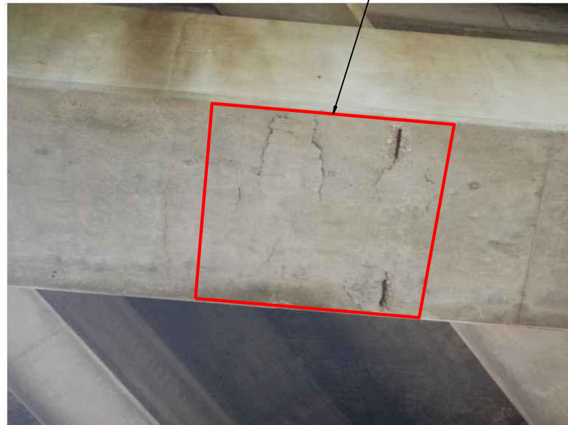
PHOTO 13 Showing Cap Spall at Bent #4
