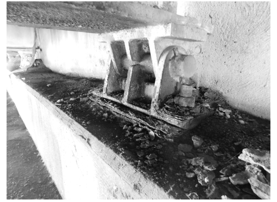
PHOTO 1: CORRODED BEARING @ ABUT. 5 @ BEAM 6 FROM WEST
