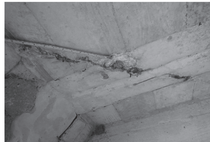
SPAN 2, BAY 5, 34-IN LONG CRACK TO BE SEALED
