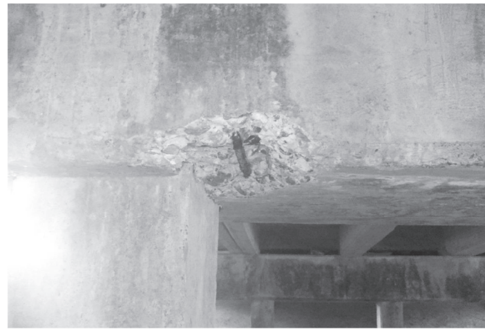
BENT CAP 10 SOFFIT SPALLING
