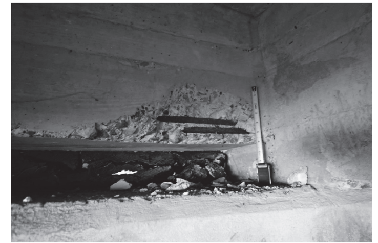
EXPOSED REBARS UNDER BEAM END AT BENT 8
