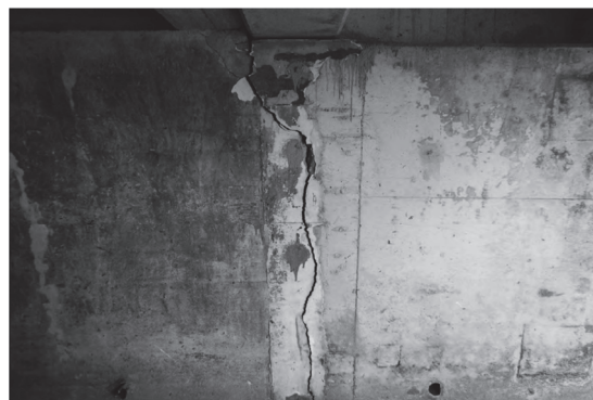
CRACK ON NORTH ABUTMENT WALL ALONG WIDENING JOINT
