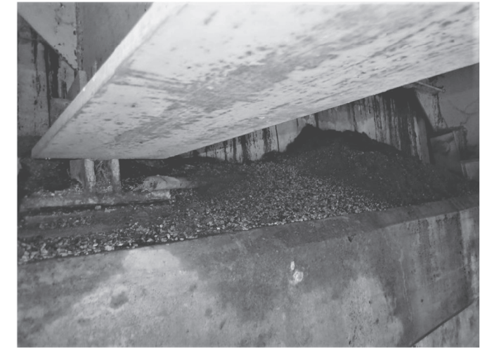
STEEL BEARING ON BENT 6 AND ACCUMULATED DEBRIS
