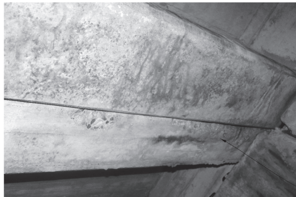
BEAM 3, ABUTMENT 1 SPALL
