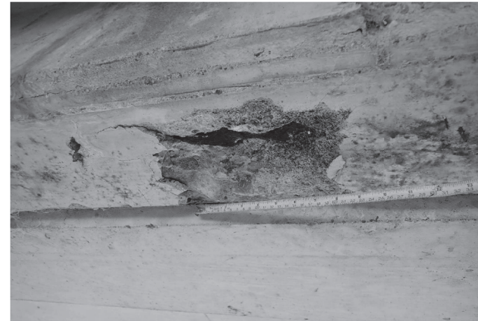
SPAN 2, BEAM 7 EXPOSED REBAR
