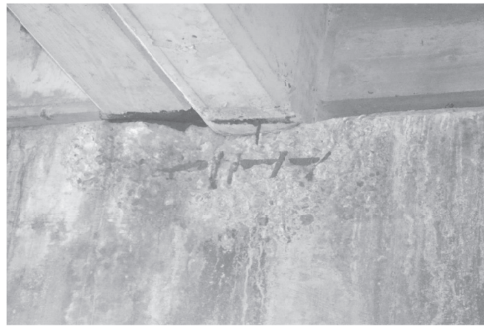
EXPOSED REBARS UNDER BEAM END AT BENT 8
