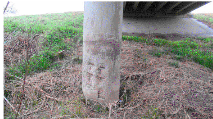
SOUTHWEST INTERIOR BENT - LOOKING SOUTHWEST NOTE: MODERATE SPALL WITH EXPOSED REBAR IN SOUTHEAST COLUMN OF SOUTHWEST INTERIOR BENT. VIEW 5776
