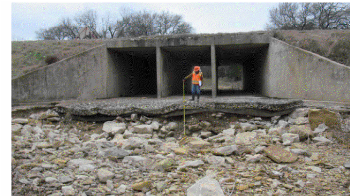
STREAM UNDER BRIDGE - LOOKING WEST VIEW 6253 NOTE: SEVERE SOUR AND UNDERMINED UP TO 64" DEEP ALONG GIBBON APRON TOEWALL AND 32" DEEP ALONG PORTION OF WING-WALL FOOTINGS.
