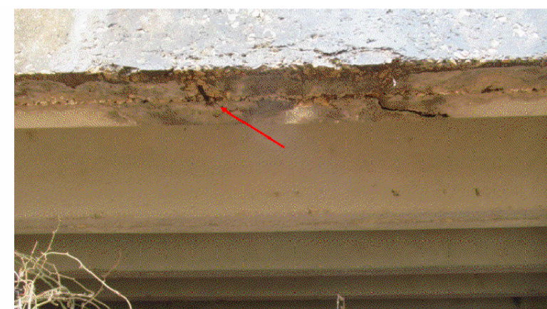
PHOTO #1 SOUTH EXTERIOR PAN GIRDER STEM - LOOKING NORTHWEST VIEW 6016 NOTE: SOUTH EXTERIOR PAN GIRDER STEM OF WEST SPAN HAS MINOR CRACKS AND MODERATE SCALING WITH EXPOSED REBAR NEAR WEST END.
