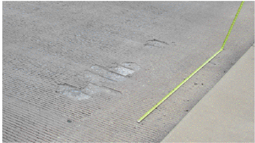
SPAN 9 DECK - LOOKING SOUTHEAST NOTE: MODERATE SPALLS WITH UP TO 6 SQUARE FEET OF EXPOSED REBAR IN SOUTHBOUND LANE IN SPAN 9 FROM NORTHWEST. VIEW 2076
