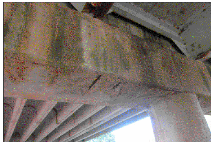
PHOTO #1 Note: Cap at bent 6 from NW has minor horizontal cracks along top edge and minor to moderate delaminations and spalls (up to 27"x18") with exposed rebar at underside.
