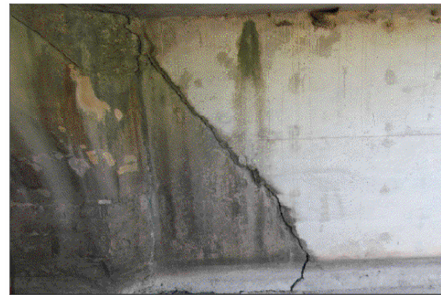
E EXTENSION N ABUTMENT WALL CRACKING Looking N IMG. 0845
