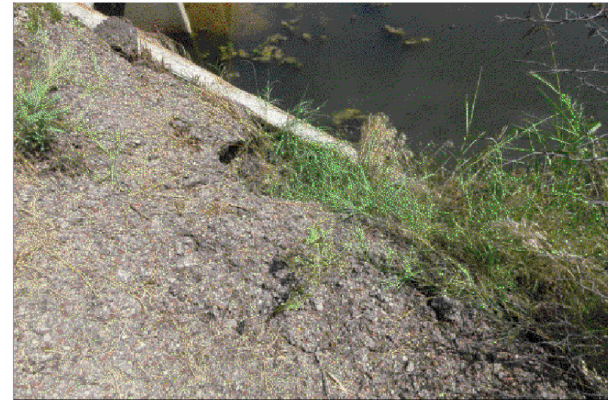
Note; Undermining of asphalt rip rap at SE corner.
