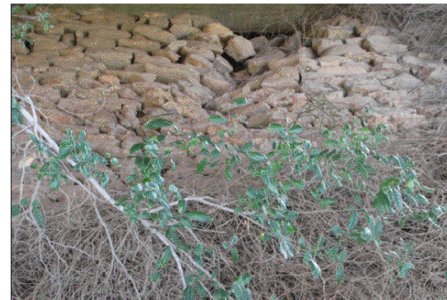
Note: Erosion at rip rap for the SW abutment.
