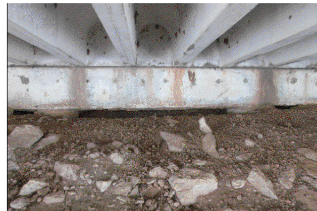
EROSION AT W ABUTMENT CAP Looking W IMG. 017
