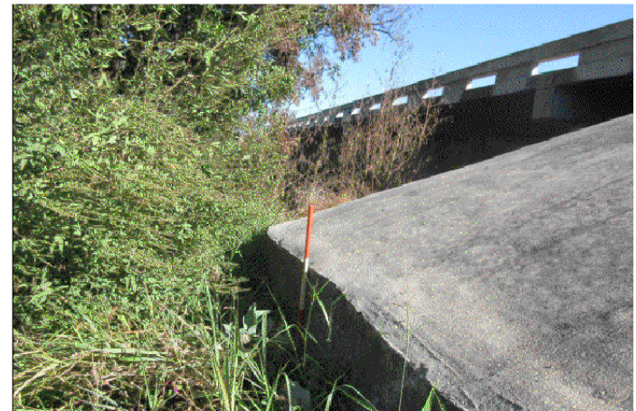
Note: Channel bank erosion at the SW drainage ditch has exposed the concrete riprap toe wall Approx. 3'
