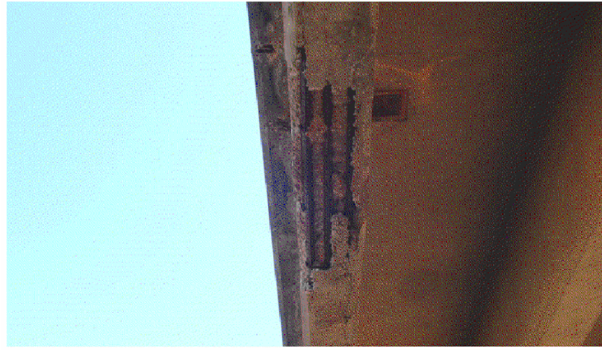
SPALL ON SPAN 1 EXTERIOR BEAM - LOOKING EAST VIEW 390
