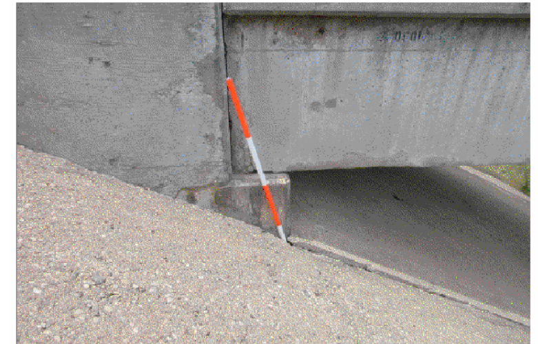
VOID Looking N IMG. 379
