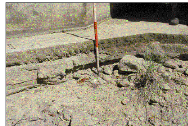
CHANNEL BED SCOUR DOWNSTREAM END Looking NW IMG. 0685
