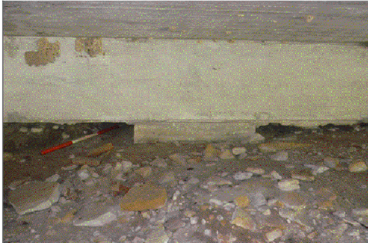
Note: Scour and erosion on the NW channel bank has undermined the NW abutment cap over a 20' of length and 1' below and 2.5' back beneath.
