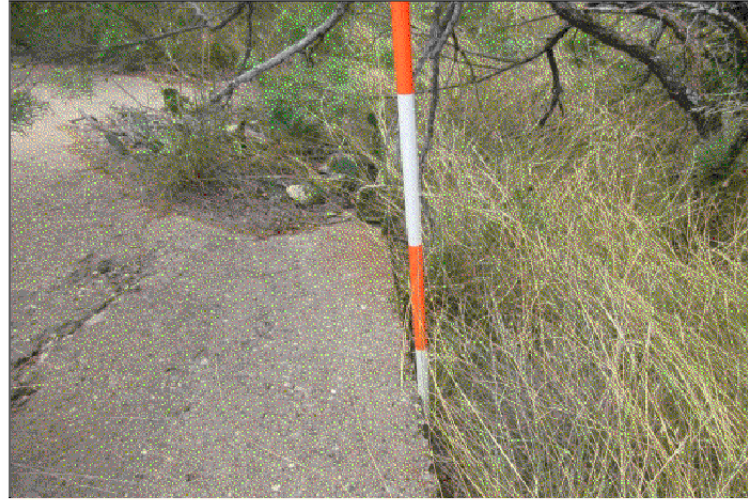
EROSION Looking N IMG. 381
