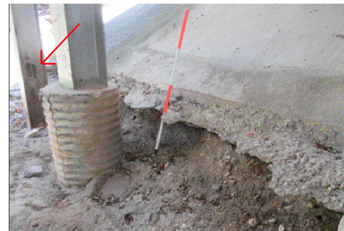
RIP RAP TOE EXPOSED AT SOUTH ABUTMENT
