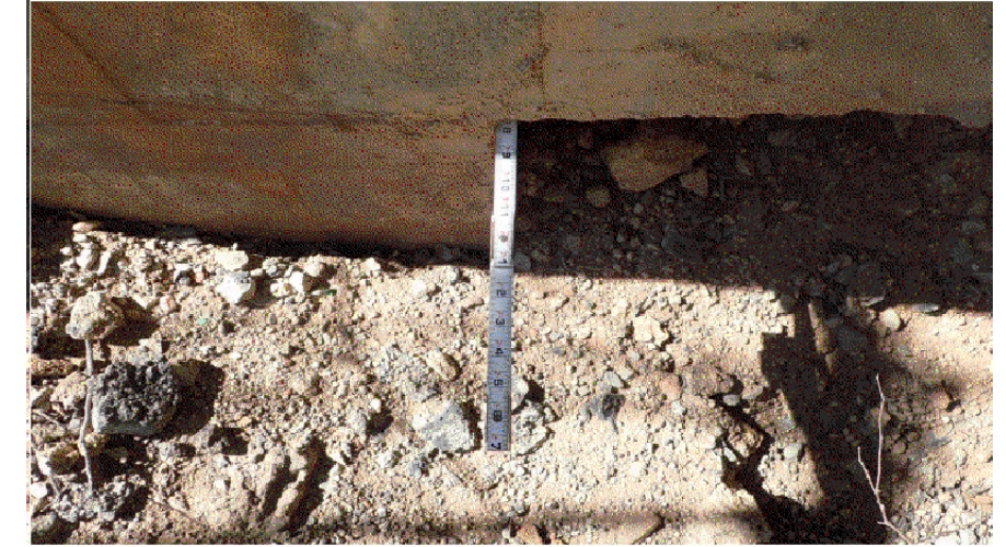
ABUTMENT 1 WALL UNDERMINING - LOOKING WEST VIEW 389
