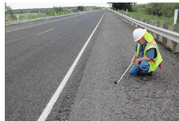
PHOTO #2 Note: Erosion hole approximately 3" in diameter and 4' from white stripe of Southbound lane and depth greater than 4' on SE end of bridge.
