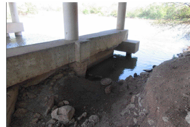
EROSION AT N END OF BENT 5 TIE BEAM Looking NW IMG. 021
