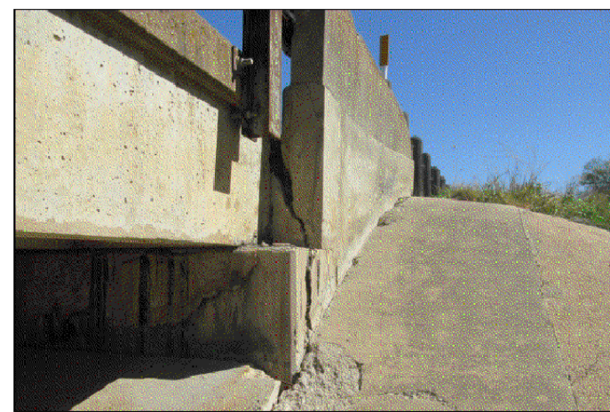
FRACTURE IN SE CORNER OF WINGWALL Looking E IMG. 114
