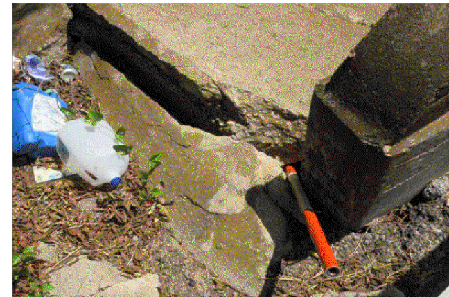
Note: Embankment erosion has undermined top of concrete riprap at NE corner approx. 2', causing the top corner of riprap to break away.
