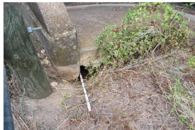
Note: Embankment erosion has undermined top of concrete riprap at SE corner approx. 3'.
