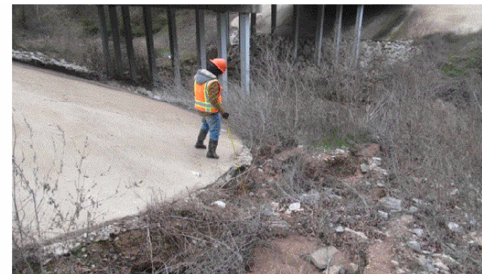
VIEW 6305 NOTE: EAST CHANNEL BANK HAS MODERATE EROSION ALONG EAST EMBANKMENT RIPRAP TOEWALL UP TO 42" DEEP.
