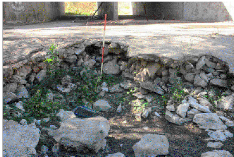
SCOUR AT DOWNSTREAM END Looking S IMG. 025
