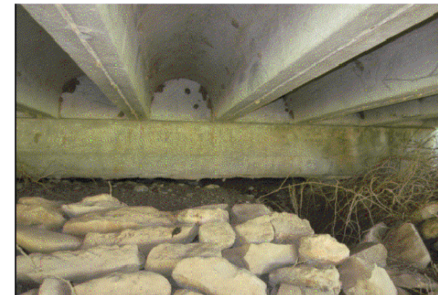
Note: Undermining at SW abutment cap.
