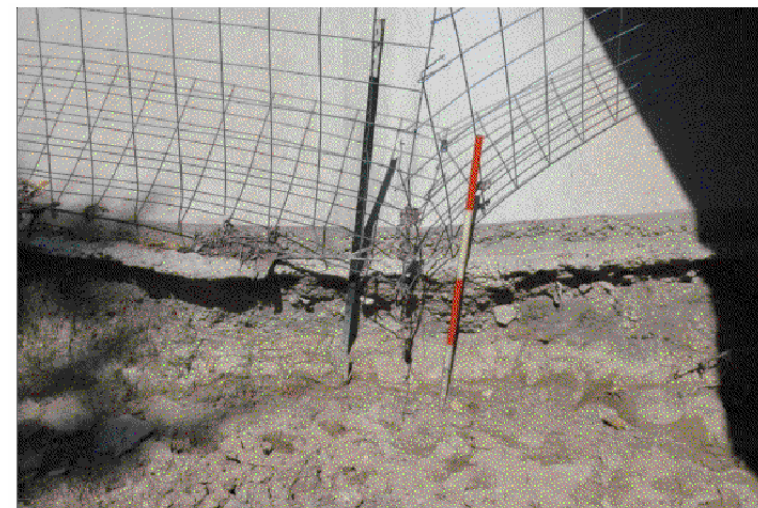
Note: Channel bed scour has exposed approx. 2.5' of concrete riprap toe of West abutment riprap at SW corner.
