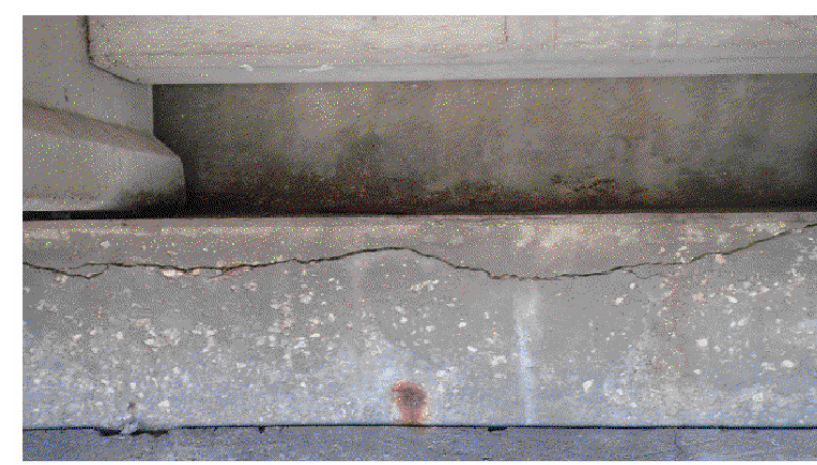
SOUTH ABUTMENT CAP - LOOKING SOUTH VIEW 120 NOTE: HORIZONTAL CRACKING UP TO 1/4" WIDE IN THE SOUTH ABUTMENT CAP. PHOTO #1
