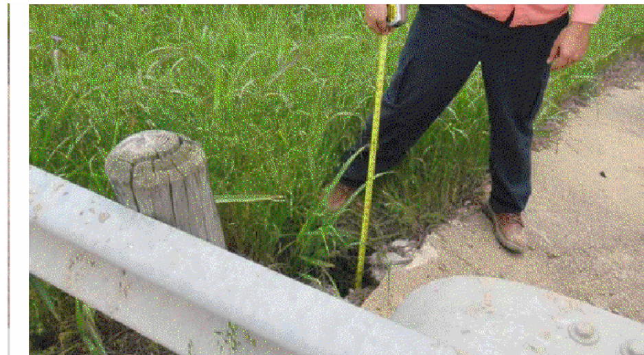
SOUTH EMBANKMENT - LOOKING SOUTHWEST VIEW 7483 NOTE: MODERATE EROSION SLOT 20" DEEP ALONG TOP EDGE OF SOUTH EMBANKMENT RIPRAP. PHOTO #1
