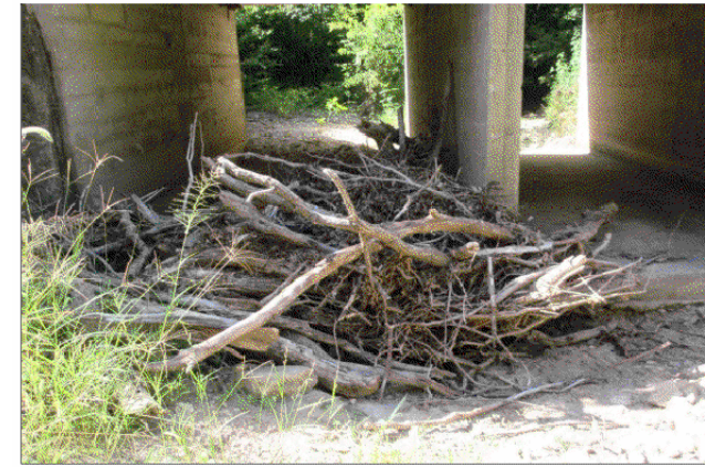
Note: Approx. 2' of drift is caught at upstream end of barrel 1.
