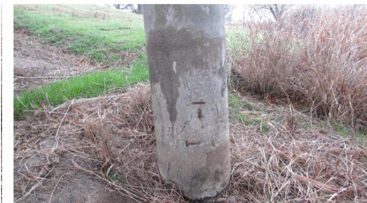
NORTHEAST INTERIOR BENT - LOOKING SOUTHEAST NOTE: MODERATE SPALL WITH EXPOSED REBAR IN SOUTHEAST COLUMN OF NORTHEAST INTERIOR BENT. VIEW 5774
