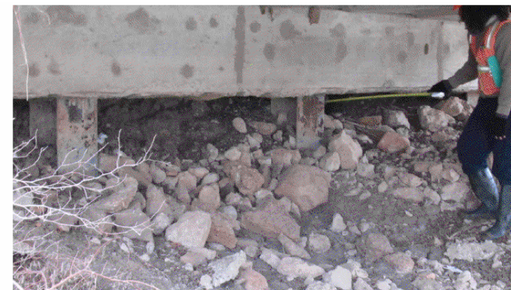
NORTHEAST ABUTMENT - LOOKING EAST VIEW 1460 NOTE: MODERATE TO ADVANCED EROSION 2' DEEP AND 21" BACK ALONG NORTHEAST ABUTMENT.
