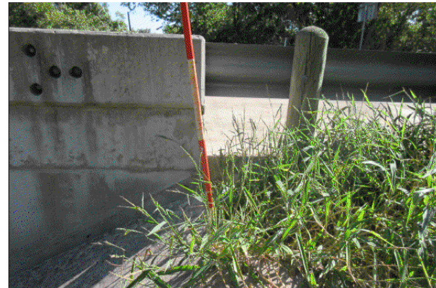
Note: Erosion at Southwest wingwall. PHOTO #1
