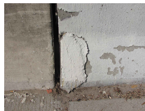
LOCATION OF CONC. CRACK REPAIR (STANDARD) ON NORTH FACE OF PARAPET FOUNDATION:
