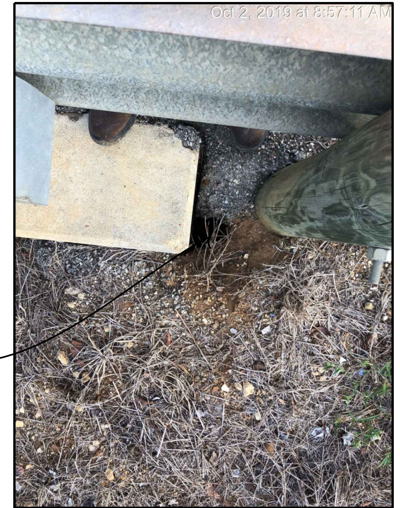
SCOUR/UNDERMINING END OF WINGWALL AT ABUTMENT NO. 18
