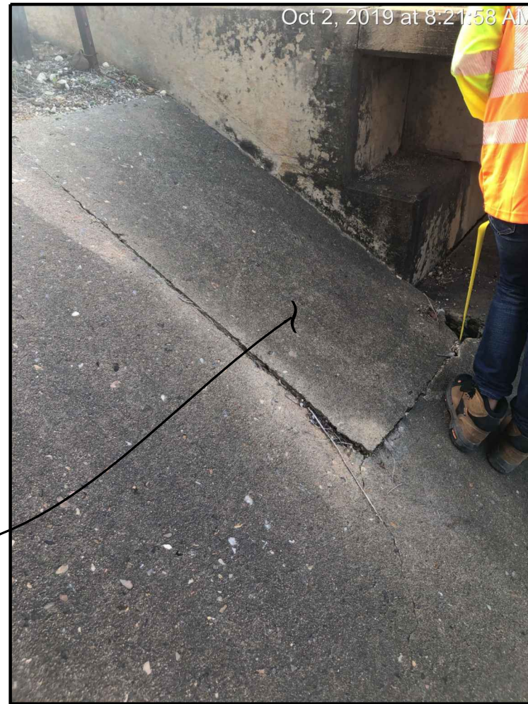
RIPRAP SETTLED AT ABUTMENT NO. 18
