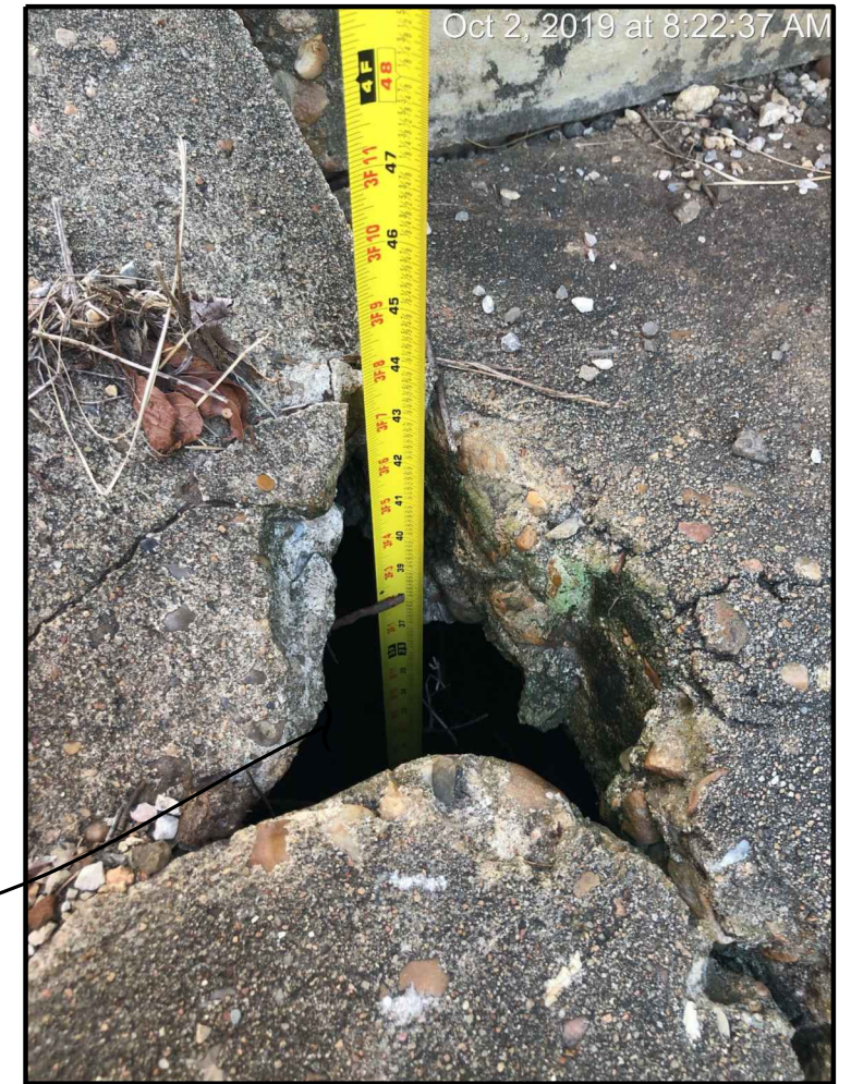
RIPRAP SETTLED AT ABUTMENT NO. 18 WITH NO FILL UNDERNEATH
