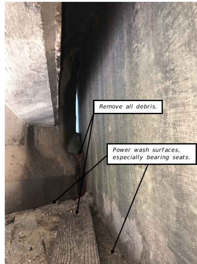
IH-610, Eastbound, East Abutment (debris picture)
