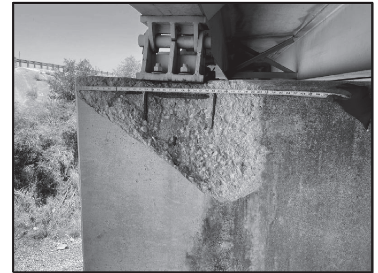
Spall at the corner of Pier 7, Span 7. Looking East
