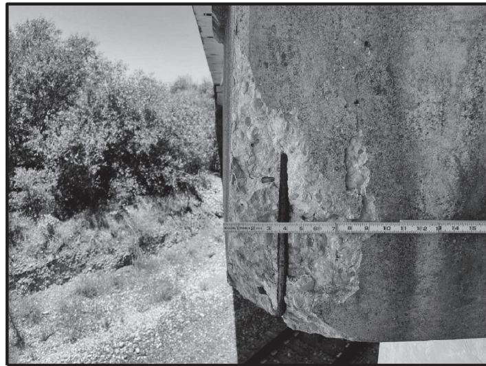
Spall at Pier 4, Span 3. Lookin West
