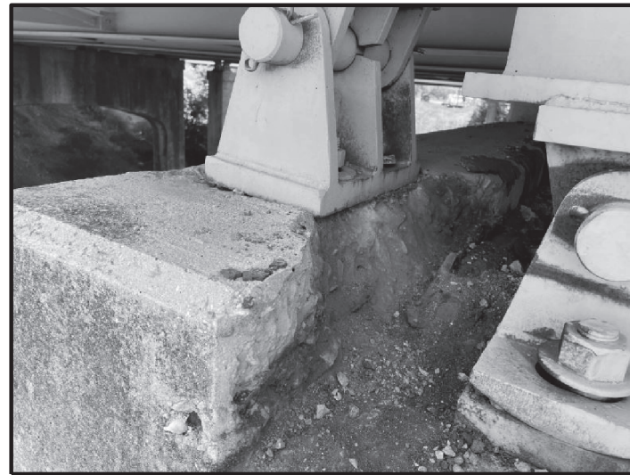
Spall under Bearing at Pier 6 Looking NW
