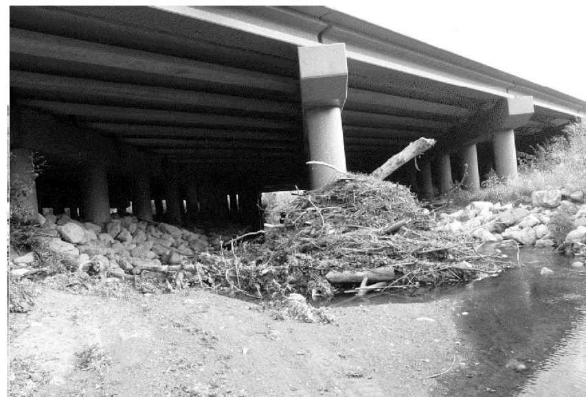
CLEAR DEBRIS AT BENT 6 COLUMNS AT IH 35E SBML BRIDGE (LOOKING EAST) ALSO CLEAR DEBRIS AT BENT 5 AND 7 COULMNS.
