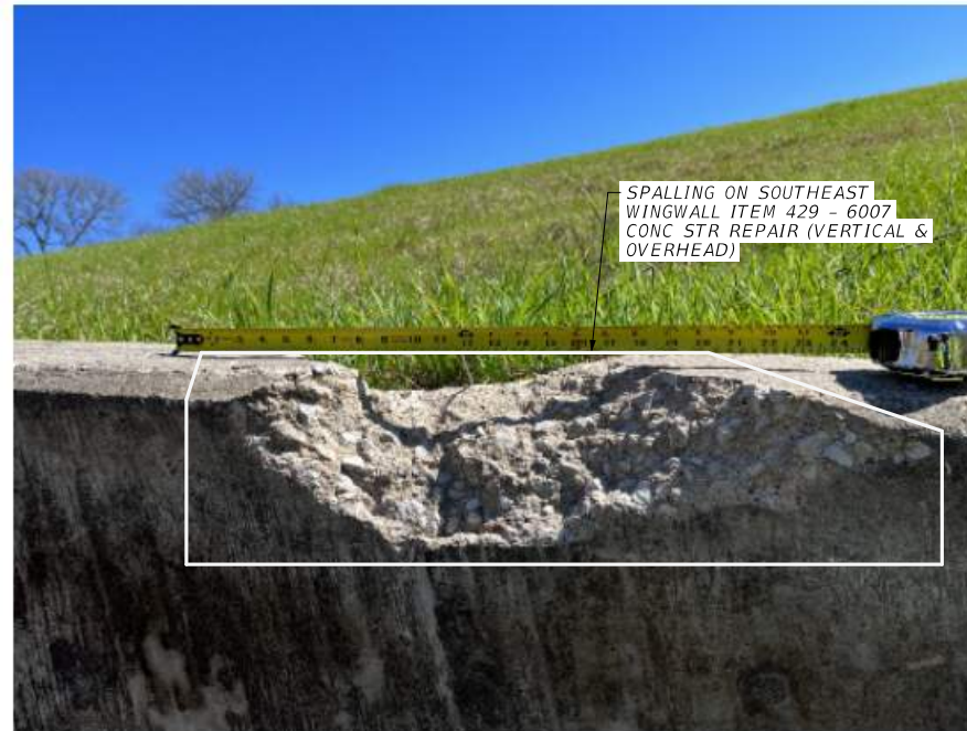
PHOTO 2 (MINOR CONCRETE SPALL IN SOUTHEAST WINGWALL)
