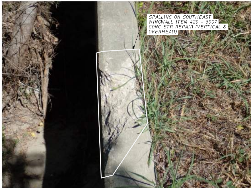
PHOTO 1 (MINOR CONCRETE SPALL IN SOUTHEAST WINGWALL)
