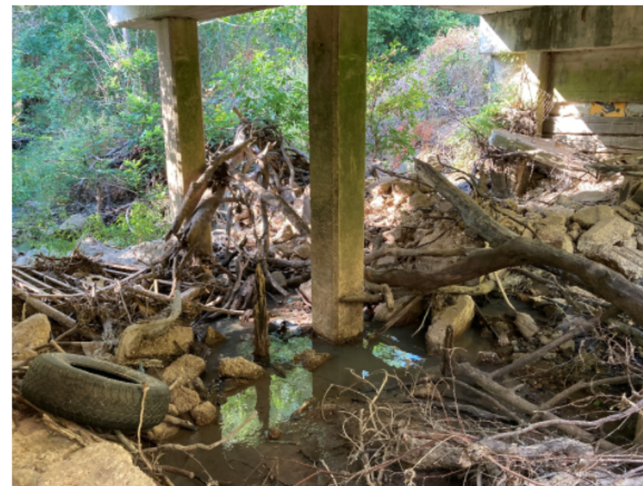
PHOTO 3 (SHOWING DRIFT AND DEBRIS ACCUMULATION UNDER BRIDGE)
