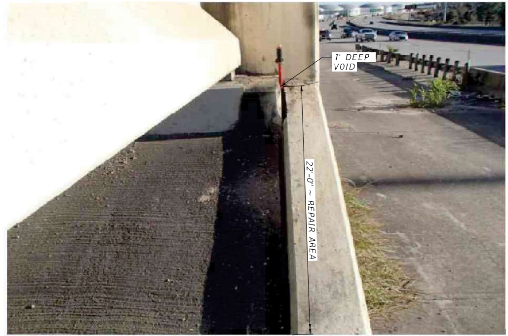
EXISTING VOID AT ABUTMENT 1 PHOTO- 12/07/2020
