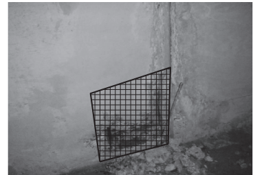
2 INTERIOR WALL CENTER OF BARREL No. 2 2 SOFT INTERMEDIATE SPALL REPAIR
