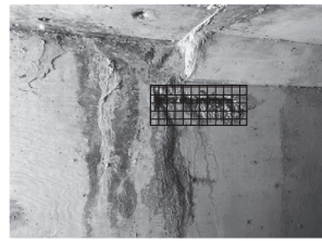
1 SIDEWALL BARREL No. 1 2 SOFT INTERMEDIATE SPALL REPAIR SIDEWALL BARREL No. 1 3 SOFT INTERMEDIATE SPALL REPAIR
