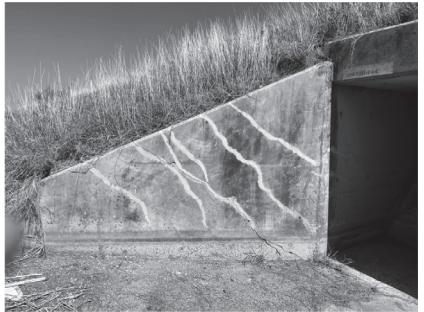
1 SOUTHWEST WINGWALL 10 LF CONCRETE CRACK REPAIR
