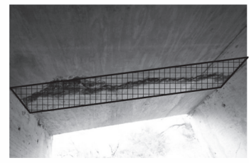
5 BOTTOM TOP SLAB BARREL No. 4 (WEST FR) 15 SOFT INTERMEDIATE SPALL REPAIR
