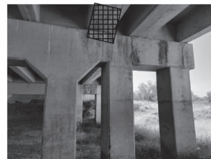
2 BENT 2 CAP 6 SQFT INTERMEDIATE SPALL REPAIR
