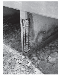
1 BARREL No. 3 2 SOFT INTERMEDIATE SPALL REPAIR
