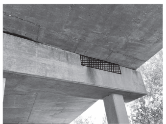
1 BENT CAP No. 3 8 SOFT INTERMEDIATE SPALL REPAIR 4 SOFT INTERMEDIATE SPALL REPAIR
