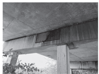
2 BENT CAP No. 4 12 SOFT INTERMEDIATE SPALL REPAIR 2 SOFT INTERMEDIATE SPALL REPAIR
