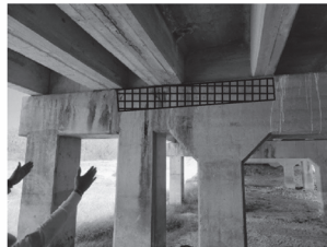
3 BENT 1 CAP 20 SQFT INTERMEDIATE SPALL REPAIR
