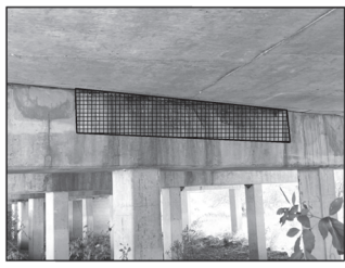
2 BENT CAP No. 6 12 SQFT INTERMEDIATE SPALL REPAIR
