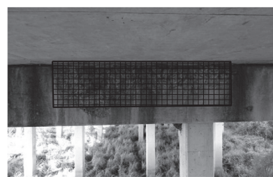
1 BENT 2 FROM NORTH ABUTMENT 14 SOFT INTERMEDIATE SPALL REPAIR
