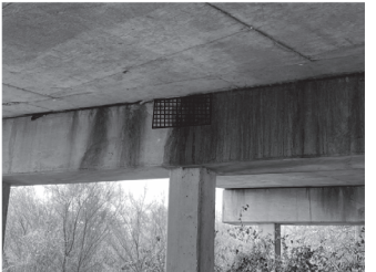
3 BENT CAP No. 6 6 SOFT INTERMEDIATE SPALL REPAIR
