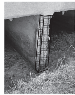
2 BARREL No. 4 8 SOFT INTERMEDIATE SPALL REPAIR
