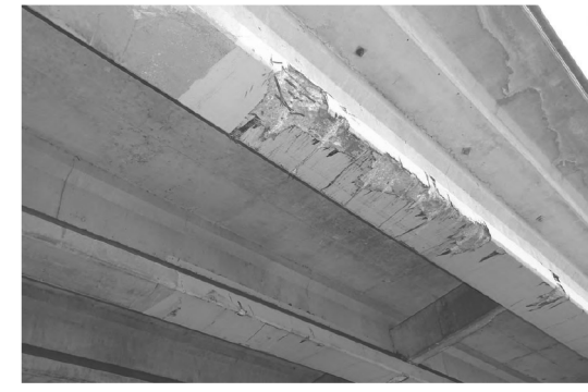
PHOTOS OF DAMAGED BEAM
