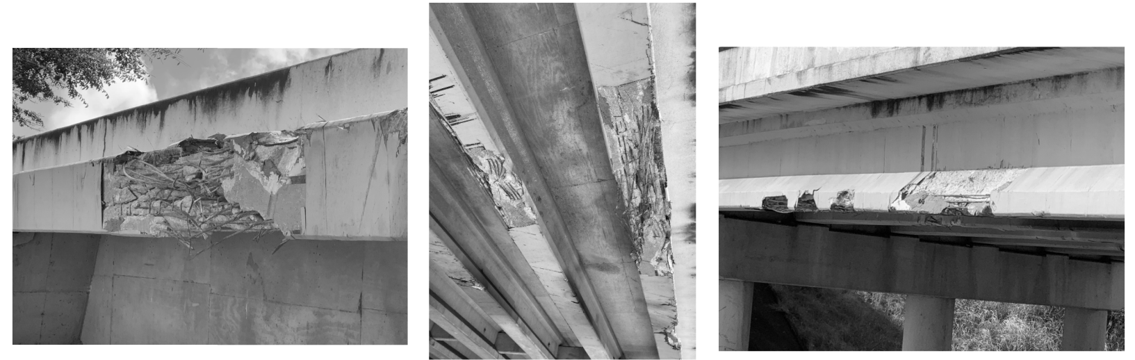
PHOTOS OF DAMAGED BEAM
