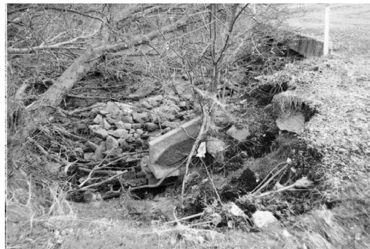
PIC:3 - LOOKING NORTH EROSION AT WEST CORNER BEHIND WEST WW BACKFILL & ROCK RIPRAP
