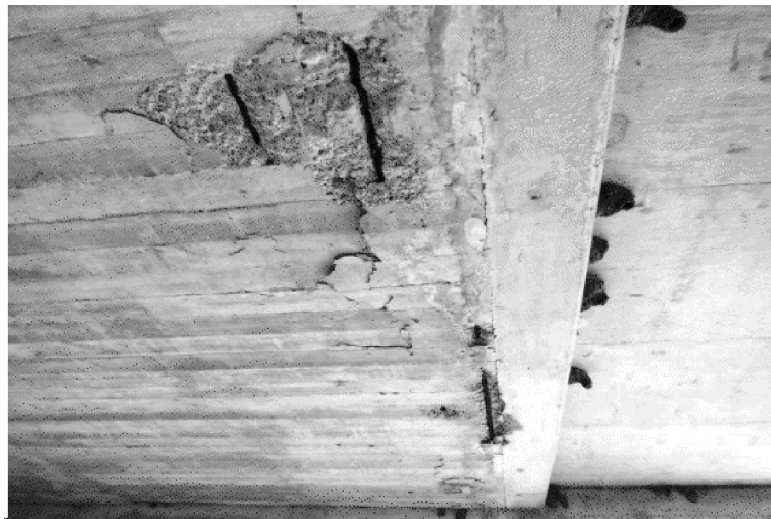
PIC:1 - LOOKING EAST SPAN 2 - DELAMINATION & SPALLING WITH EXPOSED REBAR ON SLAB SOFFIT CONC STR REPAIR (VERT & OVERHEAD)
