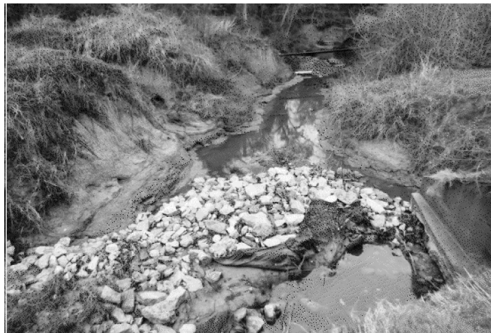
PIC:3 - LOOKING NORTH DEBRIS IN DOWNSTREAM RESHAPE DITCH
