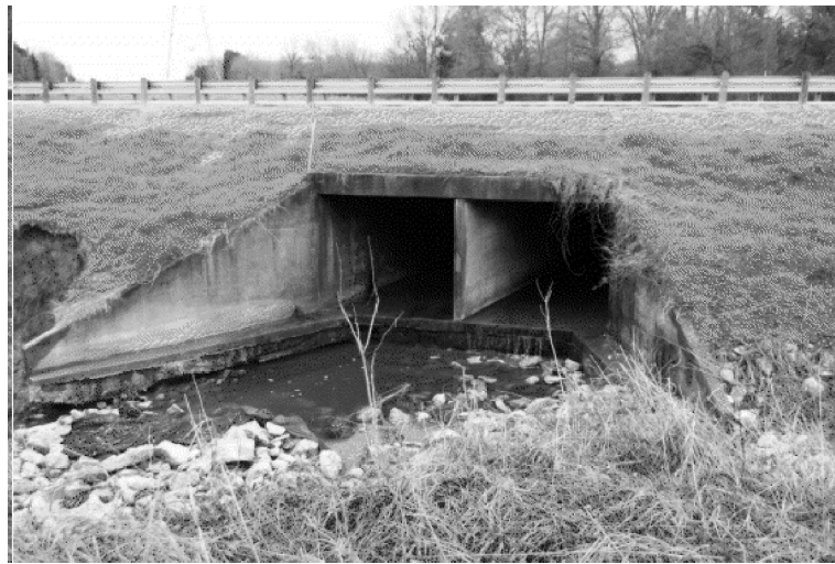
PIC:1 - LOOKING SOUTH SCOUR IN DOWNSTREAM RESHAPE, EMBANKMENT & ROCK RIPRAP
