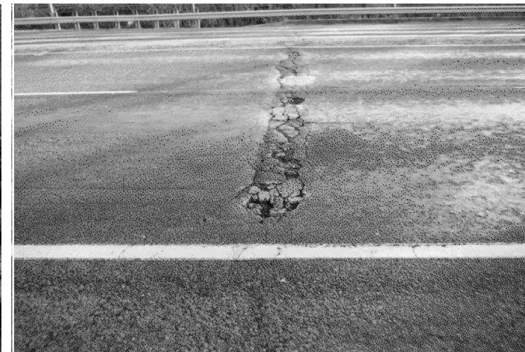
PIC:5 - LOOKING SOUTH CRACKING & SPALLING ON ASPHALT IN WB AT EAST APPROACH JOINT REPAIR
