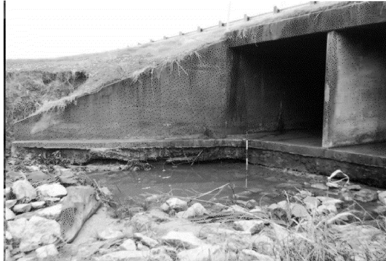
PIC:4 - LOOKING SOUTHEAST SCOUR EXPOSED IN DOWNSTREAM TOEWALL EMBANKMENT & ROCK RIPRAP
