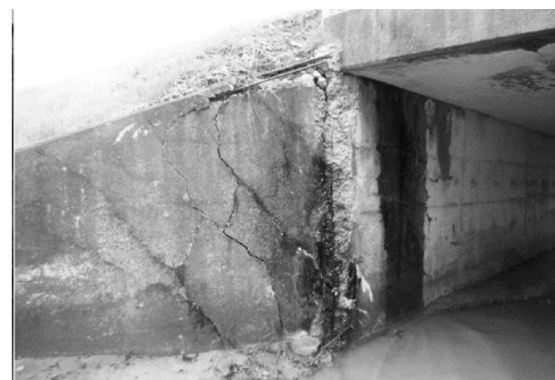
PIC:7 - LOOKING WEST CRACKED, FRACTURED & SPALLED WITH EXPOSED REBAR ON SOUTH WINGWALL LOCATION #3 - WINGWALL REPAIR
