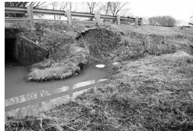
PIC:3 - LOOKING SOUTH SCOUR & EROSION WEST CORNER EMBANKMENT RESHAPE & EMBANKMENT
