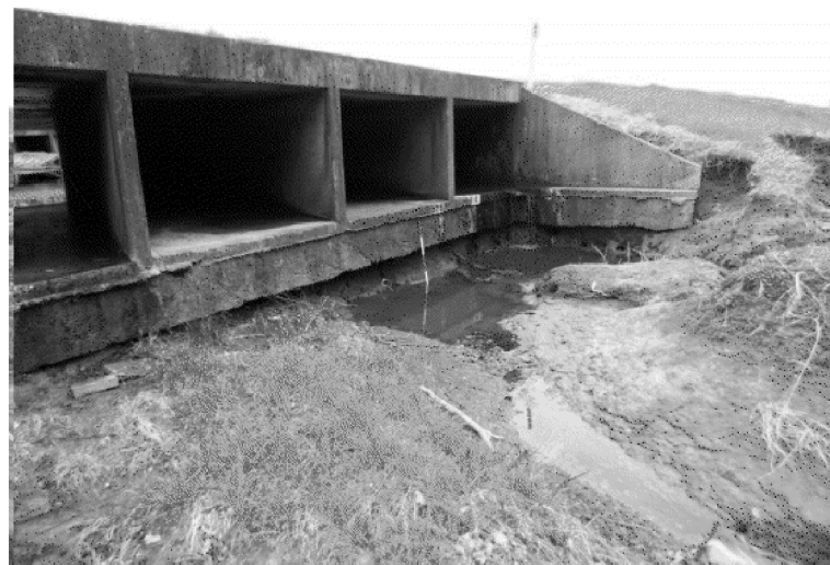
PIC:2 - LOOKING SOUTHWEST SCOUR HOLE DOWNSTREAM CHANNEL UNDERMINED BOTTOM SLAB & NW WW FOOTING EMBANKMENT & ROCK RIPRAP
