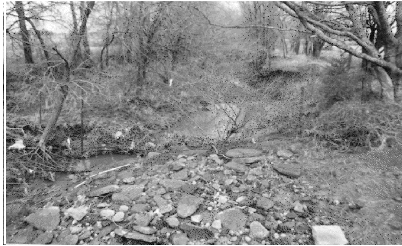
PIC:1 - LOOKING SOUTHEAST DEBRIS IN DOWNSTREAM RESHAPE DITCH
