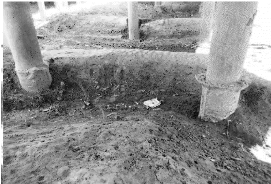
PIC:2 - LOOKING EAST BENT 4 - EXPOSED DRILLED SHAFTS EROSION AT WEST BANK BACKFILL/REGRADE BANK EROSION
