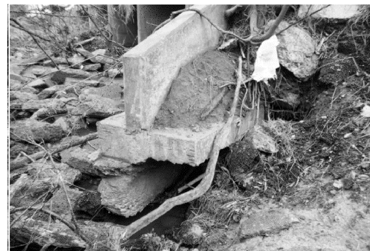
PIC:6 - LOOKING EAST UNDERMINED WEST WINGWALL BACKFILL & ROCK RIPRAP
