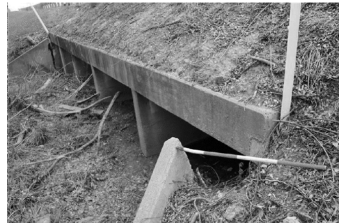
PIC:6 - LOOKING NORTH FAILED SOUTH WINGWALL
