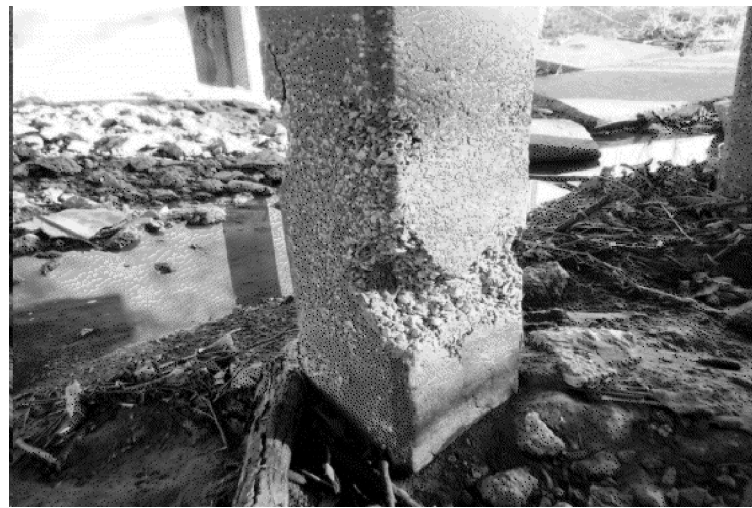
PIC:4 - LOOKING SOUTHEAST PILE 2 - SCALING, HONEYCOMBING & SPALLING ON LOWER END CONC STR REPAIR (VERT & OVERHEAD)
