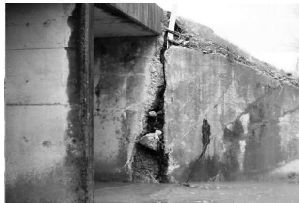
PIC:6 - LOOKING NORTHEAST TILTED & FRACTURED EAST WINGWALL LOCATION #4 - WINGWALL REPAIR
