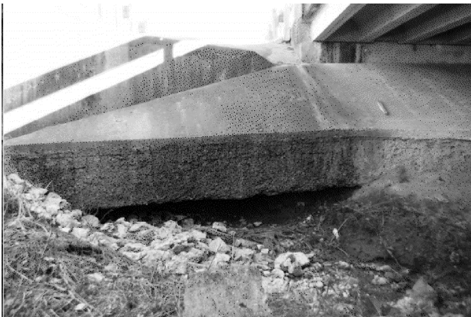
PIC:3 - LOOKING EAST NE CORNER RIPRAP BACKFILL 8' OF UNDERMINING FLOWABLE BACKFILL (8' +)
