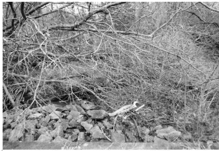
PIC:2 - LOOKING NORTHWEST DEBRIS AT DOWNSTREAM REMOVE DEBRIS & RESHAPE DITCH
