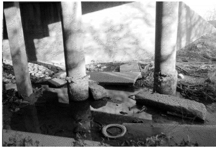
PIC:2 - LOOKING EAST BENT 2 - EXPOSED DRILLED SHAFTS EMBANKMENT & ROCK RIPRAP FOR EXPOSED DRILLED SHAFT
