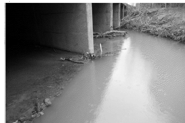
PIC:5 - LOOKING NORTH SCOUR AT UPSTREAM TOEWALL BACKFILL & ROCK RIPRAP
