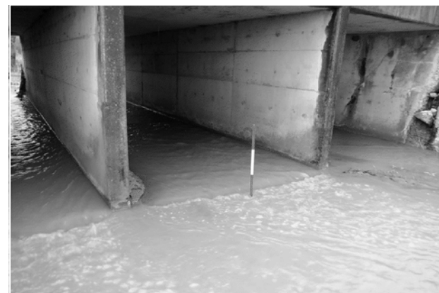
PIC:8 - LOOKING NORTH SCOUR IN DOWNSTREAM CHANNEL BACKFILL & ROCK RIPRAP - SCOURED AREA
