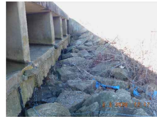
Pic. 4 Channel Bed Erosion (Down Stream)
