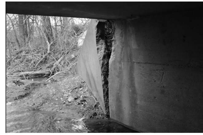
PIC:7 - LOOKING WEST FALLING WEST WINGWALL FRACTURED & SPALLED (6" SEPARATION GAP)
