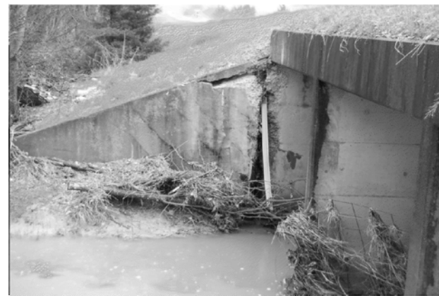
PIC:5 - LOOKING NORTHEAST TILTED & FRACTURED NORTH WINGWALL LOCATION #2 - WINGWALL REPAIR
