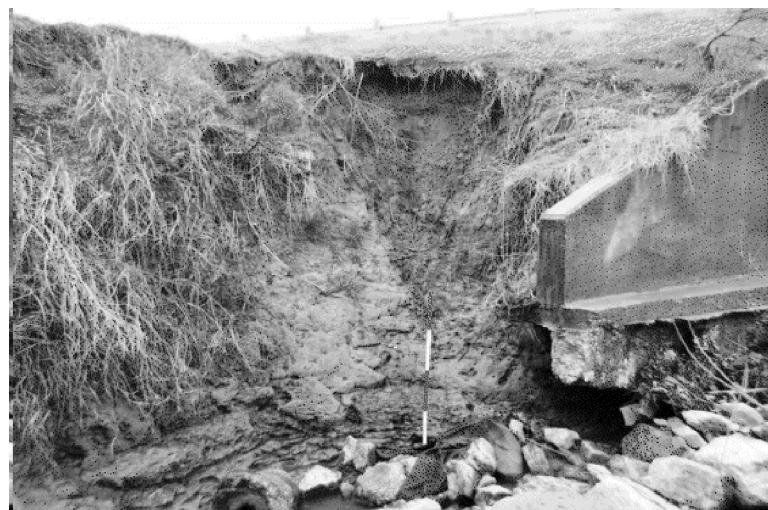
PIC:5 - LOOKING EAST SCOUR NORTH CORNER & UNDERMINED WW EMBANKMENT & ROCK RIPRAP
