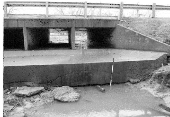
PIC:2 - LOOKING NORTHWEST SCOUR DOWNSTREAM TOEWALL BACKFILL & ROCK RIPRAP
