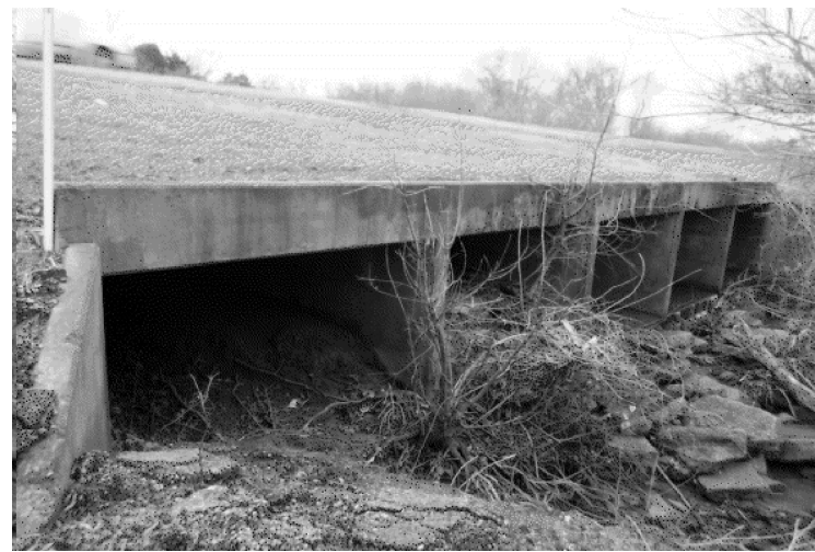
PIC:1 - LOOKING SOUTH DEBRIS AT DOWNSTREAM REMOVE DEBRIS & RESHAPE DITCH
