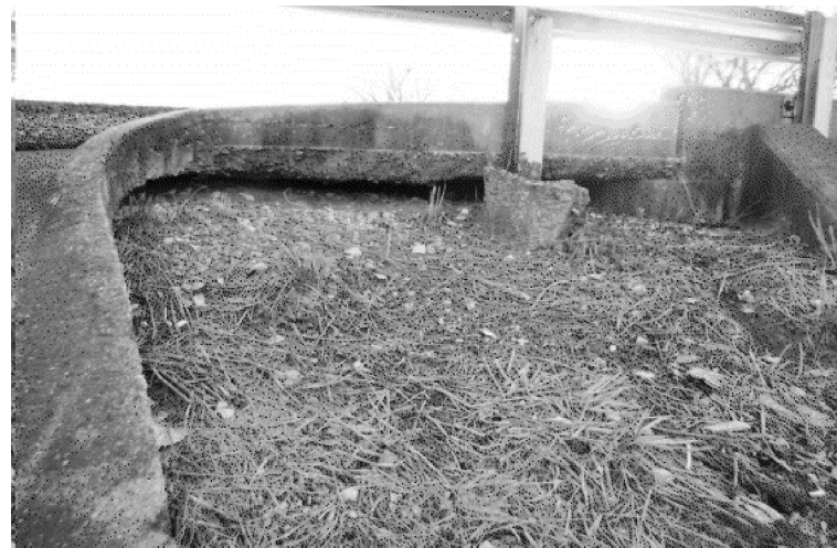
PIC:6 - LOOKING SOUTH UNDERMINING OF EMBANKMENT AT NE CORNER FLOWABLE BACKFILL NE CORNER
