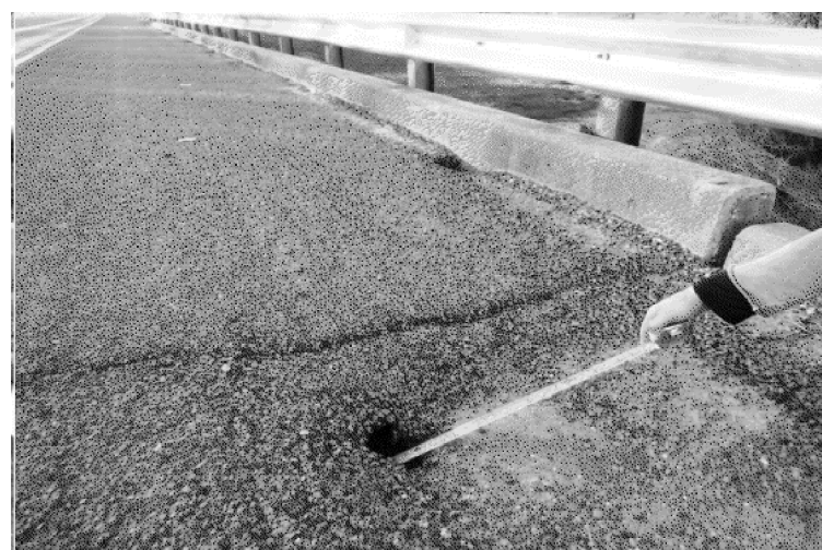
PIC:7 - LOOKING NORTHWEST HOLE IN ASPHALT AT NORTH SHOULDER ON EB APPROACH FLOWABLE BACKFILL
