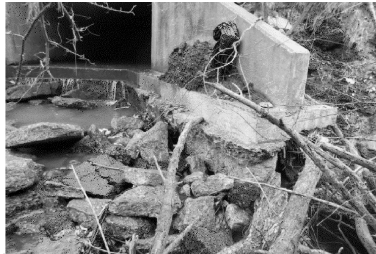
PIC:4 - LOOKING SOUTHEAST DOWNSTREAM SCOUR EXPOSING TOEWALL & WEST WINGWALL BACKFILL & ROCK RIPRAP
