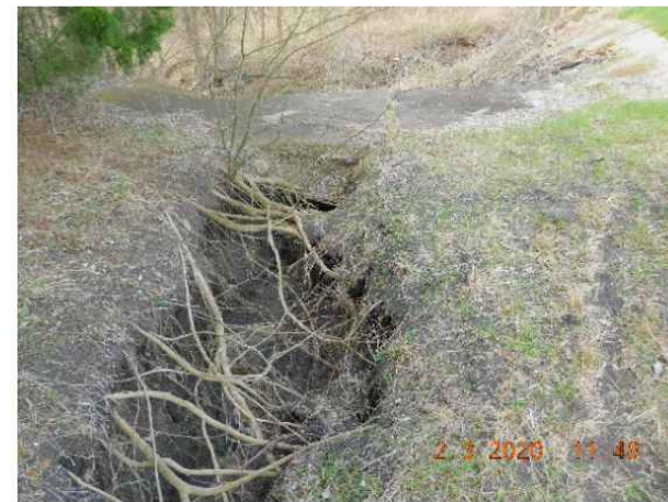
Pic. 6 Washed Out Ditch At SE Riprap
