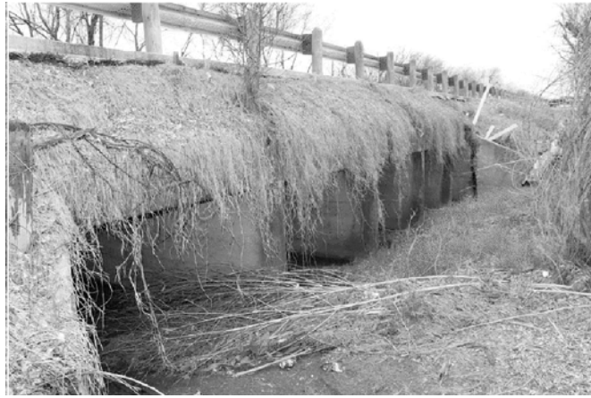
PIC:1 - LOOKING NORTHWEST DEBRIS CLEAN - UPSTREAM
