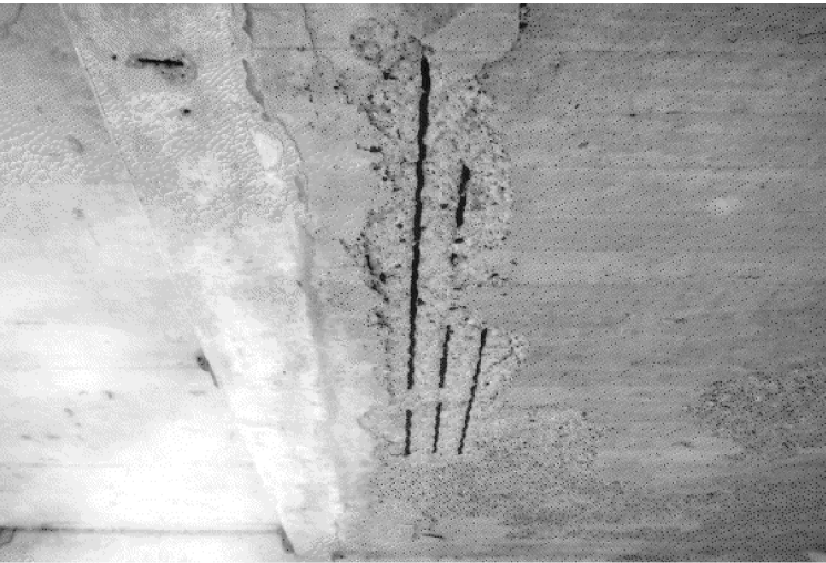
PIC:3 - LOOKING WEST SPAN 3 - SCALING & SPALLING WITH EXPOSED REBAR ON SLAB SOFFIT CONC STR REPAIR (VERT & OVERHEAD)
