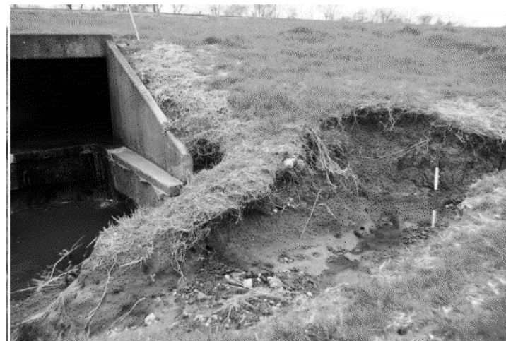
PIC:4 - LOOKING SOUTHWEST EROSION EMBANKMENT & BOTTOM OF WW EMBANKMENT & RESHAPE DITCH EMBANKMENT & ROCK RIPRAP
