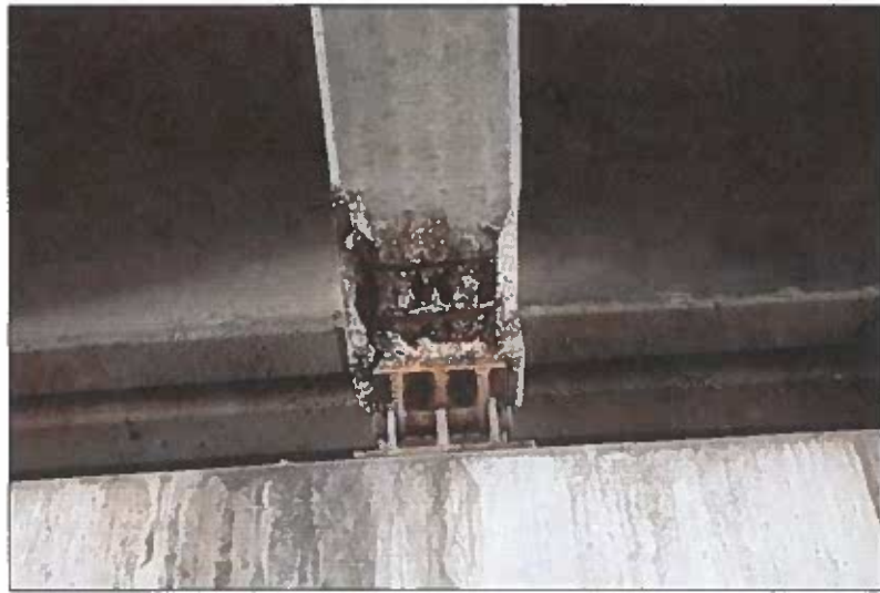
① SPALL IN BEAM 11 FROM NORTH SPAN 2 AT WEST END
