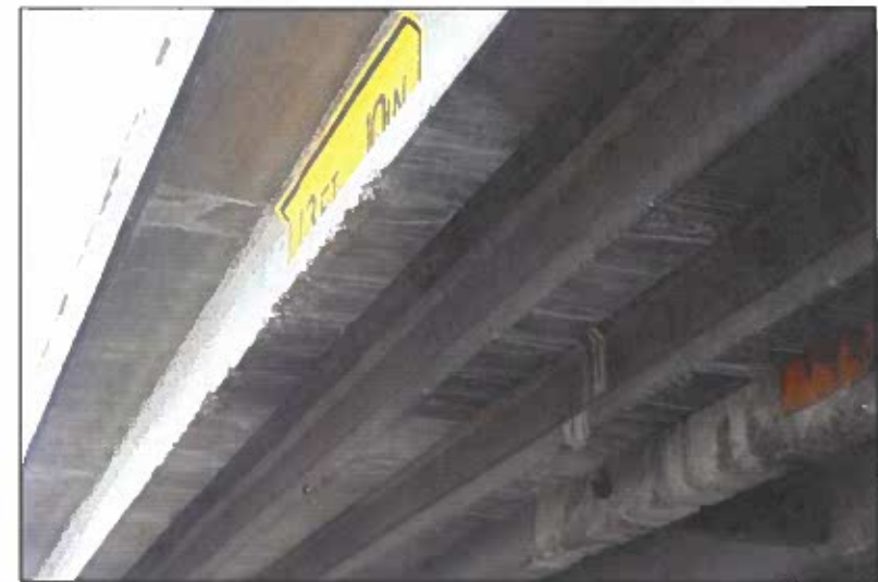
③ TYPICAL IMPACT DAMAGE TO BEAMS SPAN 3
