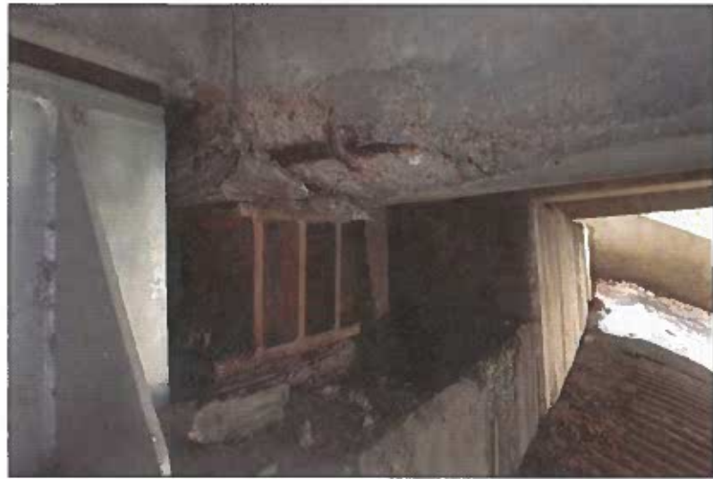
① SPALL AT EAST END OF BEAM 3 FROM SOUTH SPAN 5
