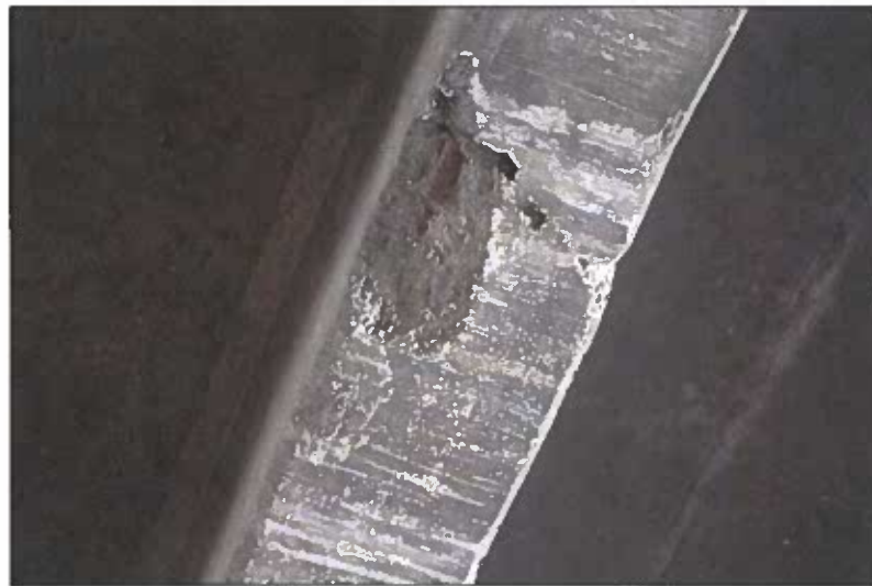
④ IMPACT SPALL BEAM 8 FROM NORTH SPAN 3
