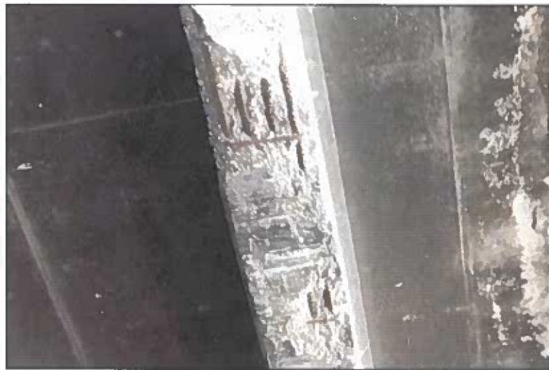
② IMPACT SPALL WITH EXPOSED REBAR BEAM 5 FROM SOUTH SPAN 3
