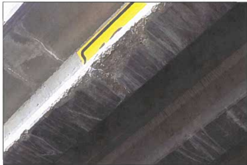
④ EXPOSED TENDON BEAM 1 FROM SOUTH SPAN 3
