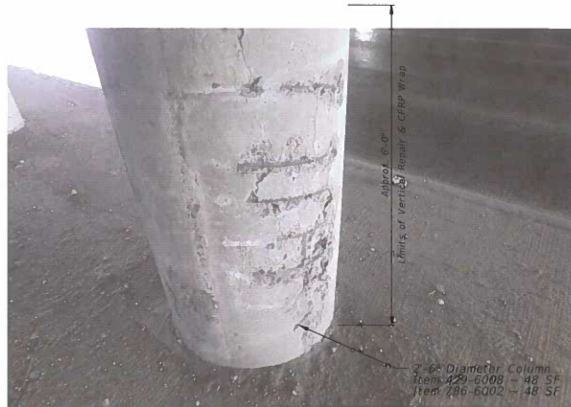
BENT 4R COLUMN DETERIORATION PHOTO
