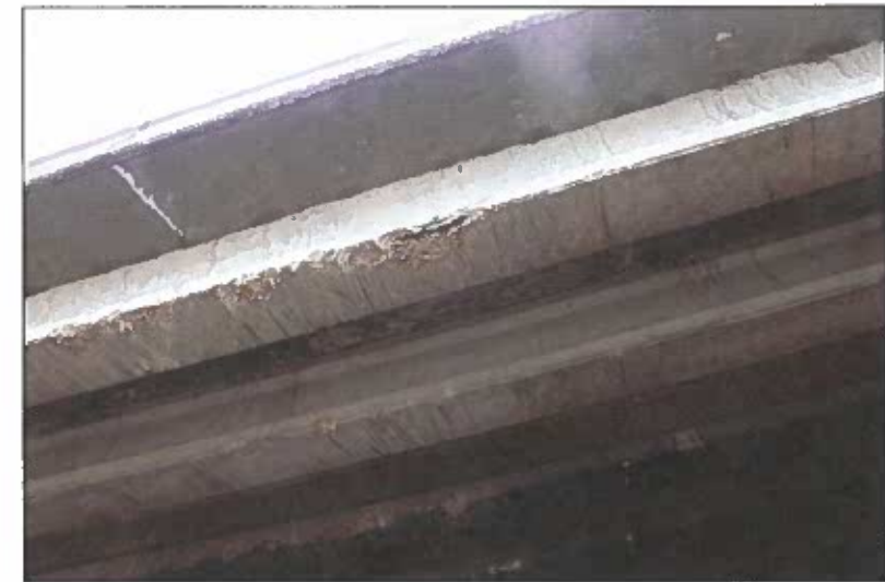
⑥ EXPOSED STRANDS BEAM 1 FROM NORTH SPAN 3
