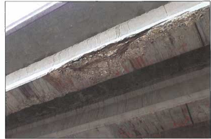
③ SEVERED STRANDS BEAM 1 FROM NORTH SPAN 3
