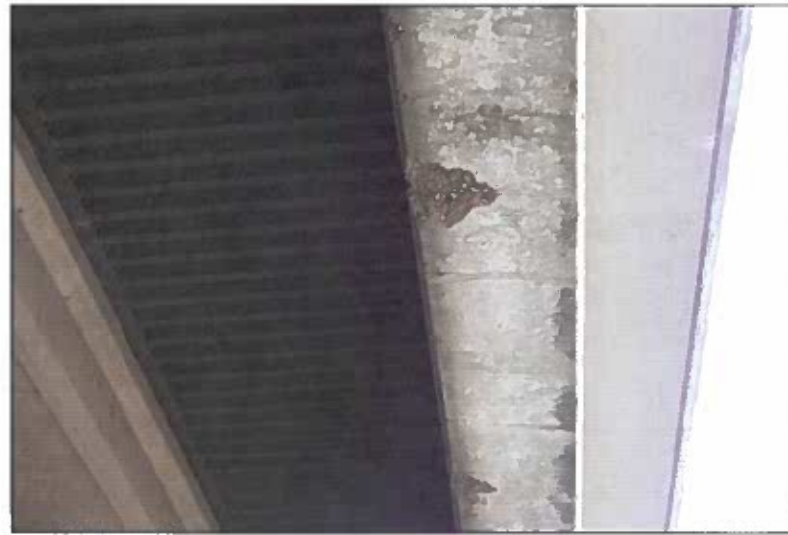
② IMPACT DAMAGE NORTH BEAM SPAN 2
