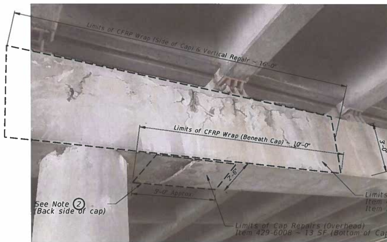
BENT 5R CAP DETERIORATION PHOTO LOOKING EAST ~ 9/10/2020
