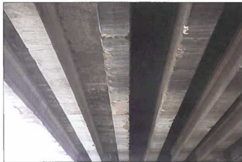
⑦ TYPICAL IMPACT DAMAGE TO BEAMS
