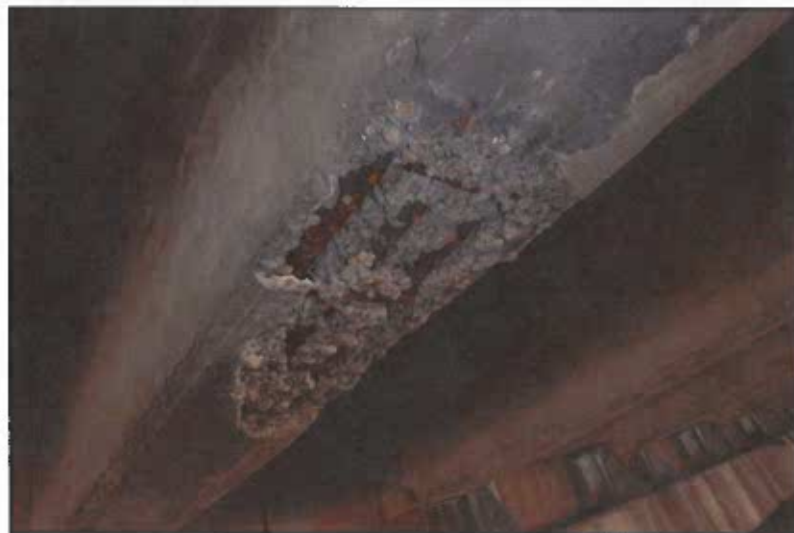
⑤ SPALL WITH EXPOSED REBAR BEAM 10 FROM SOUTH SPAN 1
