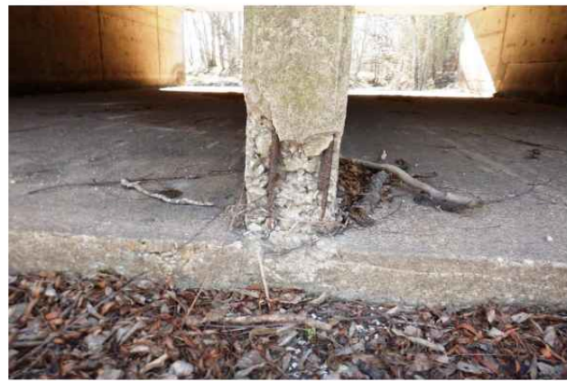
SPALL WITH EXPOSED REBAR ON UPSTREAM END OF WEST INTERIOR WALL LOOKING SOUTH
