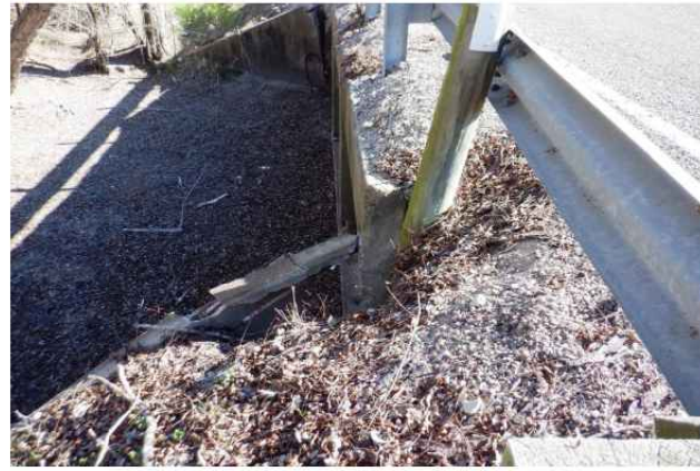
LOSS OF EMBANKMENT AT NW CORNER WITH LOSS OF EMBEDMENT OF GUARDFENCE POST LOOKING EAST
