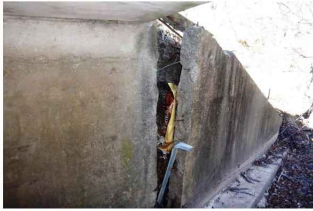
FAILED NW WINGWALL LOOKING NORTHWEST
