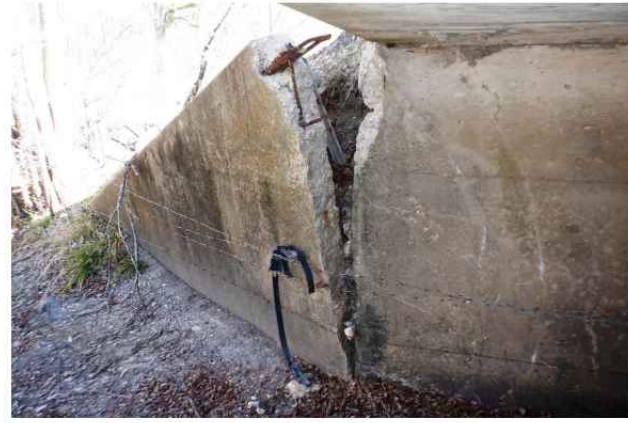
FAILED NE WINGWALL LOOKING NORTHEAST
