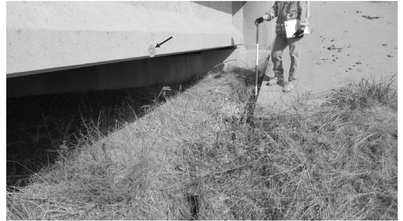
NORTHWEST ABUTMENT - LOOKING NORTHWEST VIEW 3944 NOTE: MODERATE EROSION ALONG NORTH EMBANKMENT RIPRAP. EROSION HAS EXPOSED RIPRAP TOE UP TO 15" DEEP. NORTHEAST EXTERIOR BEAM OF NORTHWEST SPAN HAS A MINOR SPALL IN BOTTOM FLANGE.
