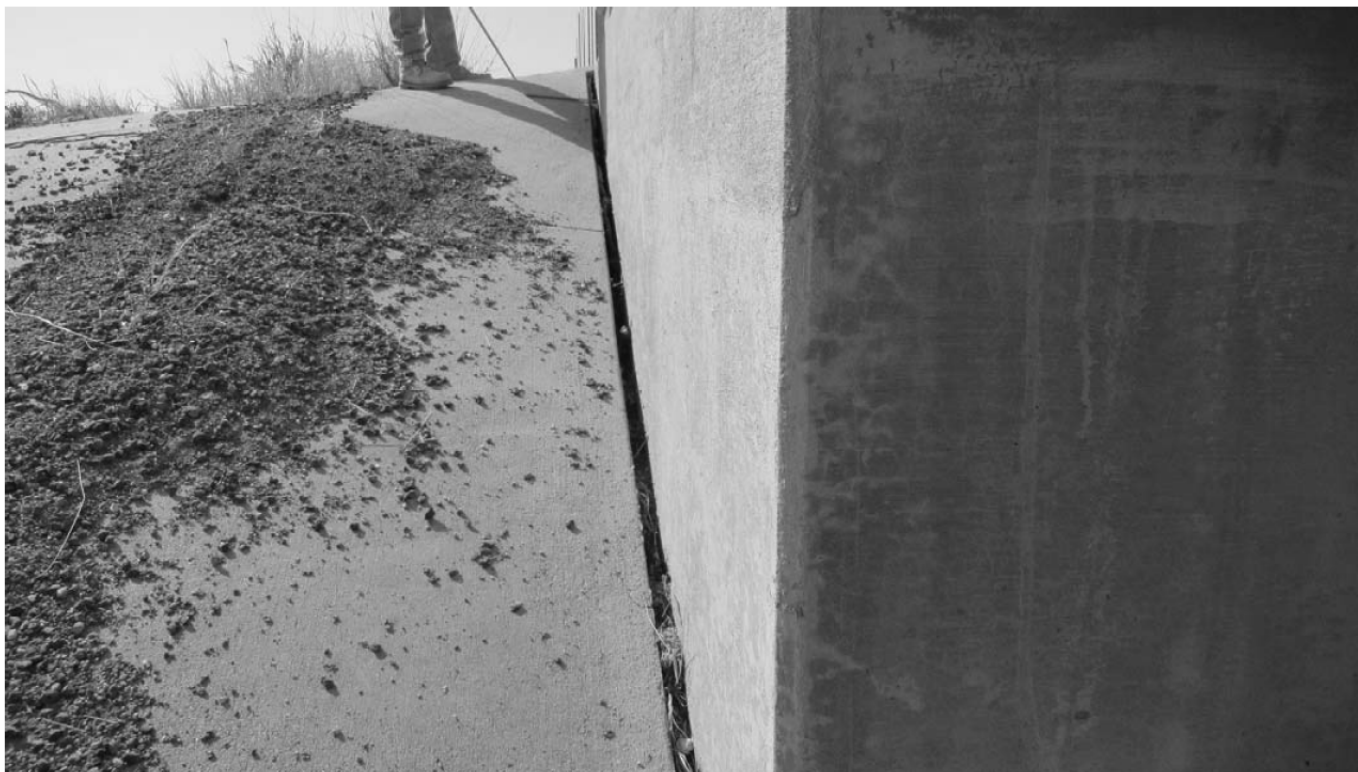
EAST EMBANKMENT - LOOKING SOUTHEAST VIEW 3954 NOTE: UP TO 1.5" WIDE AND 12" DEEP GAP BETWEEN EMBANKMENT RIPRAP AND EAST WINGWALL.
