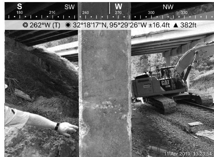
Spalls in Column
