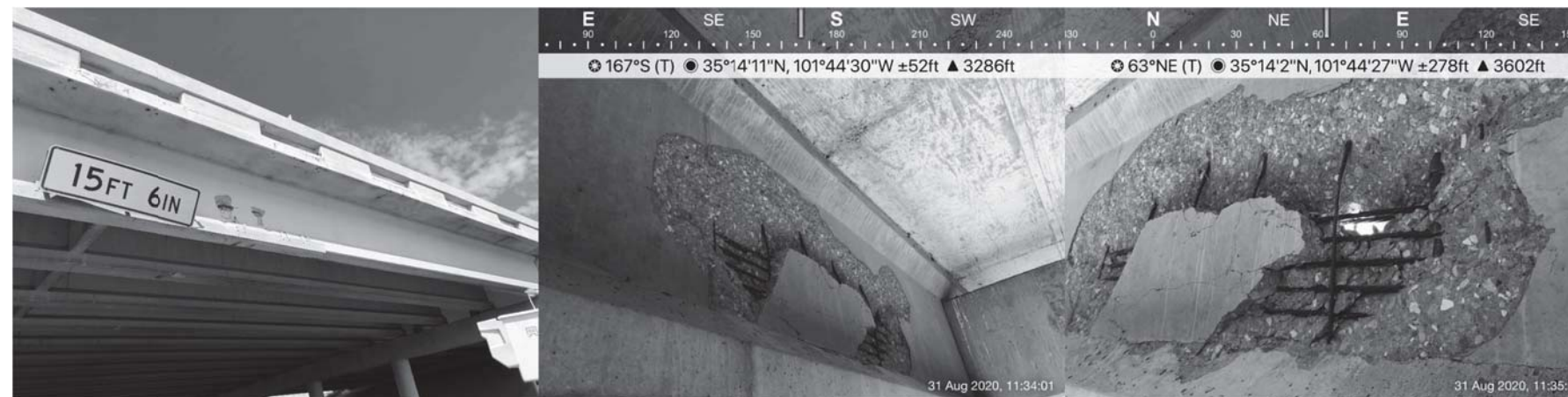
PHOTOS OF DAMAGED BEAM
